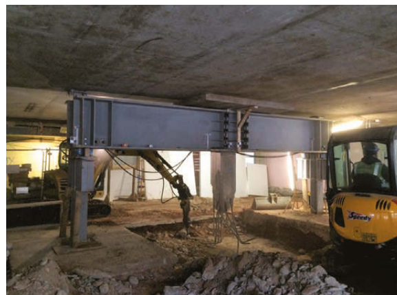
↓ FIGURE 2: Lowering existing foundations to increase floor-to-ceiling height at George Green Library, University of Nottingham
