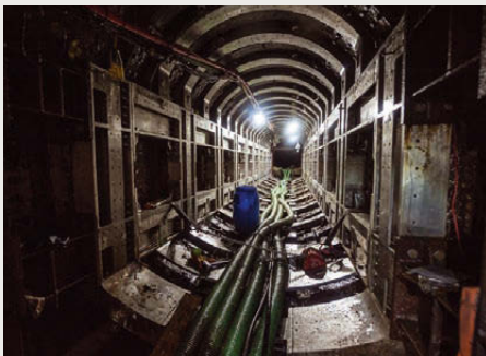
King's Scholars Pond Sewer Rehabilitation London, UK Submitted by: Transport for London
