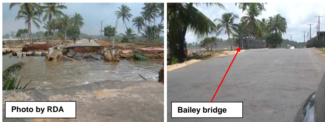
Figure 2.59: Destroyed bridge (Type 1) at Akurala and the replaced Bailey bridge
