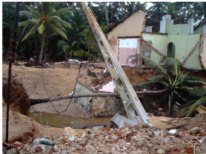
Figure 2.3: Scour damage seen in Kahawa (Galle District)
