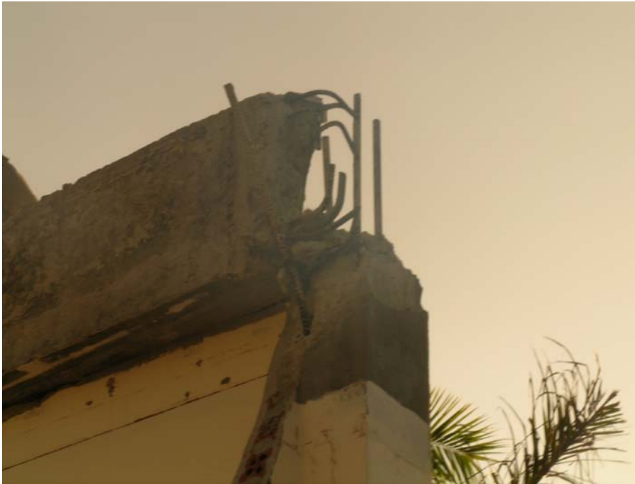
Figure 3. 24: Typical example of poor connection detail. The beam reinforcement is insufficiently anchored to the column reinforcement, leading to a lack of integrity of the connection and partial collapse of the structure shown as DC4 on the left hand side of Figure 3.32.
