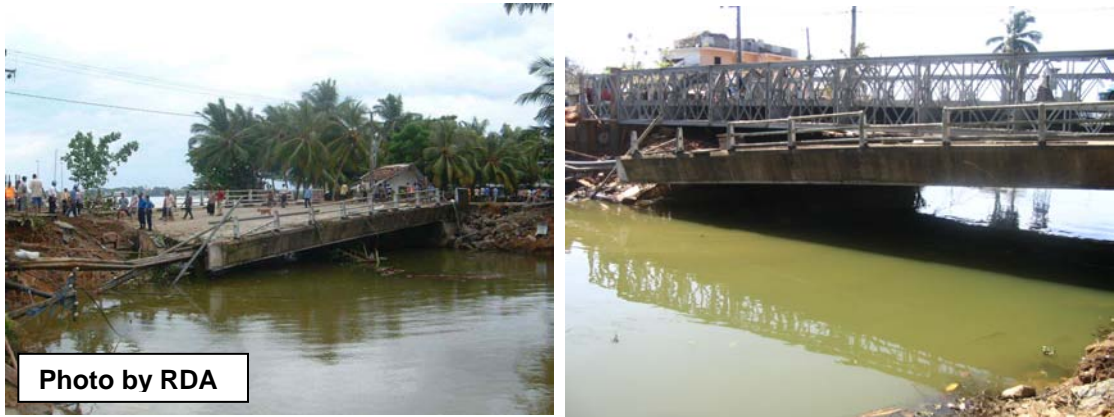
Figure 2.60: Collapsed Magalle Bridge (Type 1) south of Galle due to abutment erosion and scour damage. Temporary Bailey bridge in place to restore the vital crossing
