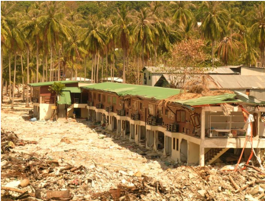
Figure 3. 19: Major damage to a resort on Phi Phi Island. The structure is located about 50m from the north beach and has extensive damage to lower storey windows and masonry walls. Debris damage to the roof is visible.
