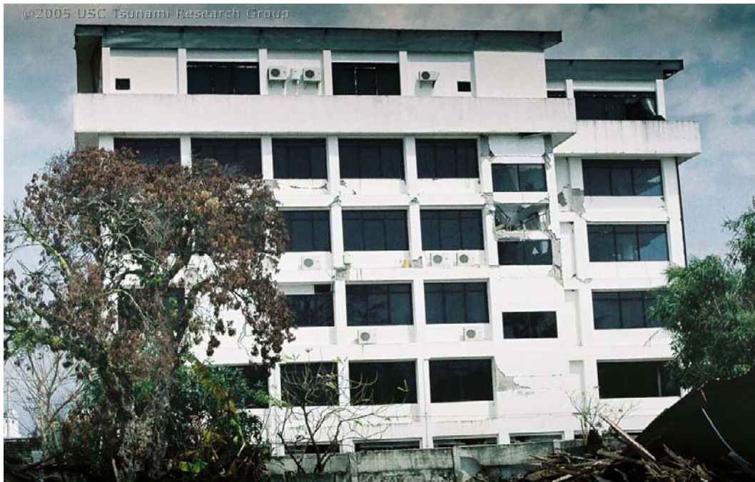
Figure 1.7: Ground shaking damage to 6-storey RC frame structure in Banda Aceh (Source: http://www.usc.edu/dept/tsunamis/2005/tsunamis/041226_indianOcean/sumatra/sumatra.html )
