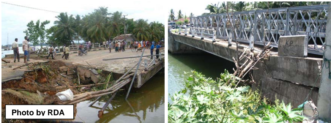
Figure 2.61: Exposed retained side of the abutment in the landward side at damaged Magalle bridge. Protected abutment on the seaward side by abutment structures running parallel to the road
