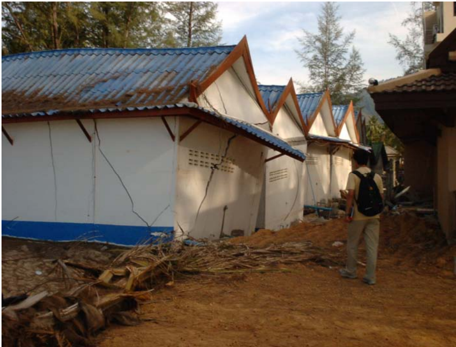
Figure 3. 9: Foundation failure of bungalows on Bang Tao beach front.
