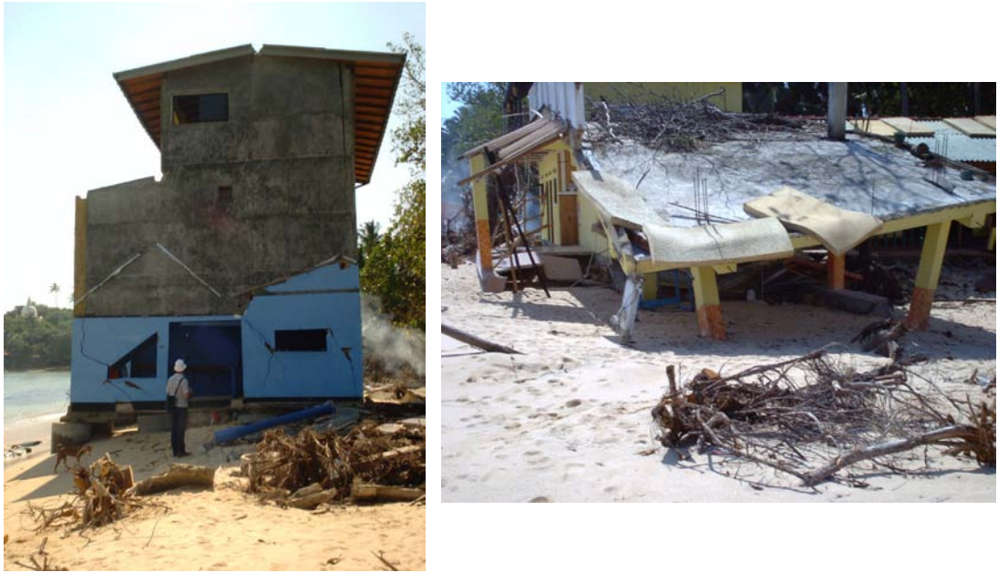
Figure 2.5: Damage to hotel structures observed on the beachfront of Unawatuna (Galle District)
