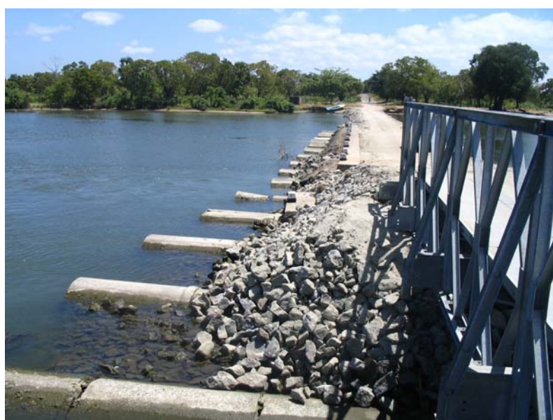
Figure 2.68: Restored causeway bridge in Kinniya near Trincomalee (Photo by Anton Pillai, Arup)
