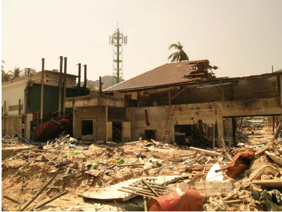
Figure 3. 20: Local power station and telecommunications building extensively damaged on Phi Phi Island. The exhaust pipes for the diesel generators remain standing at left hand side of the picture.
