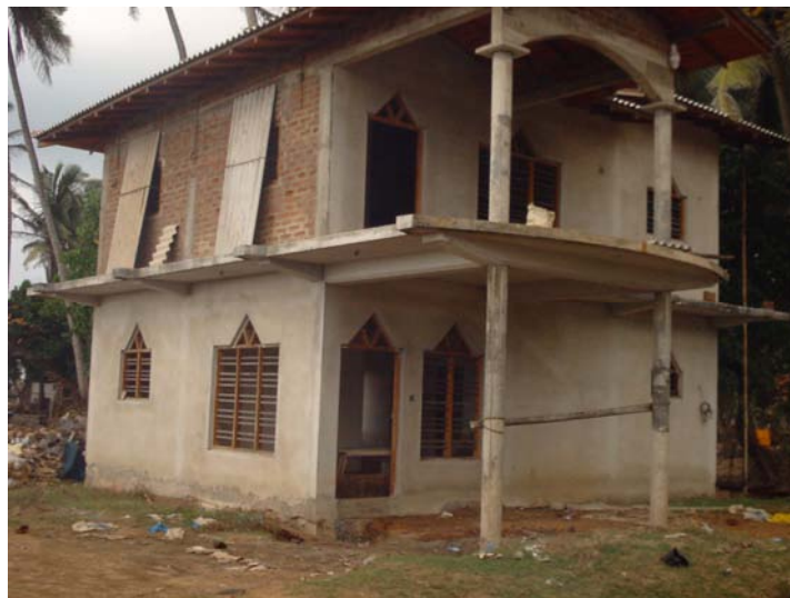
Figure 2.21: Example of the low-rise RC detached housing and small commercial buildings class of structure
