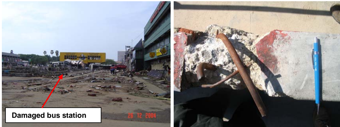
Figure 2.36: Heavily damaged Galle bus station (photo by Dennis Knight, Halcrow). Tensile failure of reinforcing bars of columns supporting the roof structures of the bus station
