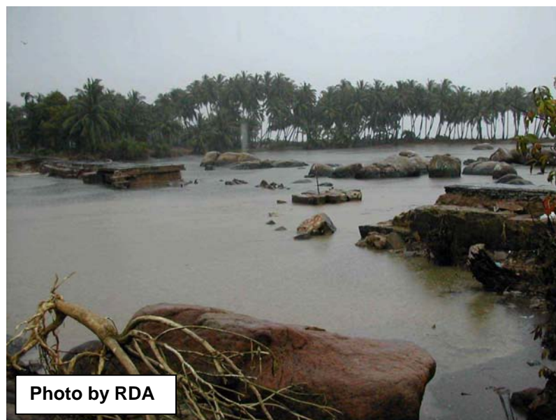
Figure 2.66: Destroyed Komari causeway bridge on the Road A4 from Colombo to Batticaloa
