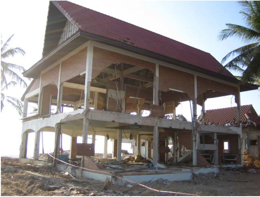
Figure 3. 11: Damage to a two storey resort on Bang Niang Beach in Khao Lak, situated approximately 50m from the sea.
