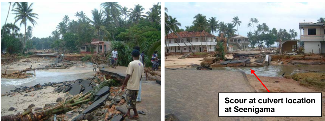
Figure 2.54: Heavy damage to the road near Hikkaduwa due to scouring making the road impassable (Photo by RDA). Completely washed away culvert in Seenigama making Road A2 impassable (Photo by RDA)
