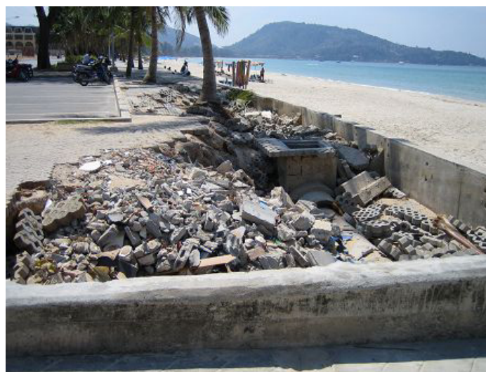
Figure 3. 42: Damaged pavement at Patong Beach, approximately 30m from the sea.
