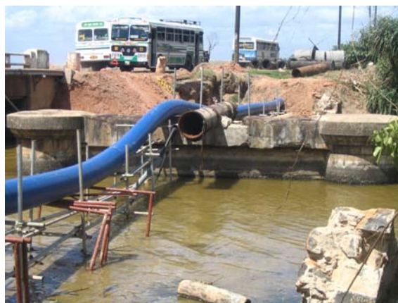
Figure 2.69: Newly restored water supply across an old bridge crossing in Dondra adjacent to the bridge where the abutments were eroded
