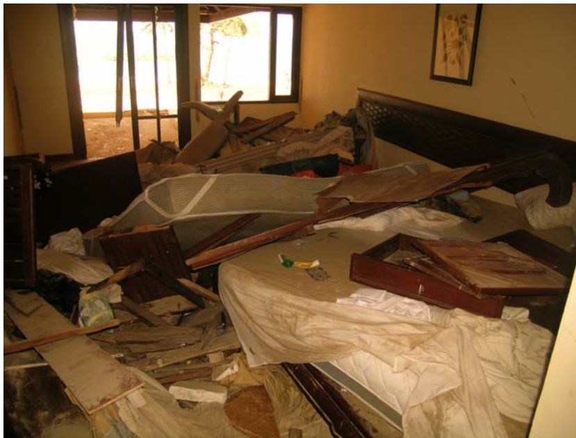
Figure 3. 50: The condition in the interior of a second floor hotel room in Khao Lak following the tsunami.
