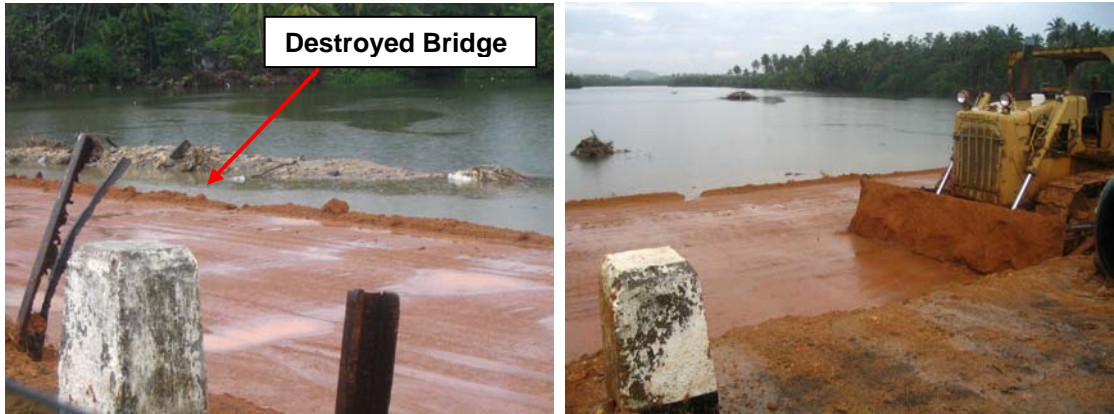
Figure 2.65: Destroyed causeway bridge at Kosgoda (north of Balapitiya). Backfilling and leveling taking place to lay a new railway track
