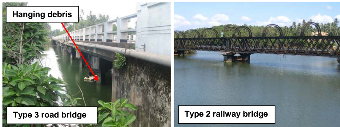
Figure 2.63: Two parallel 80m span bridges (Types 2 and 3) at Weligama that performed well. Note the presence of a fishing net suspended from the base of the road bridge deck, indicating water probably overtopped the bridge during the tsunami
