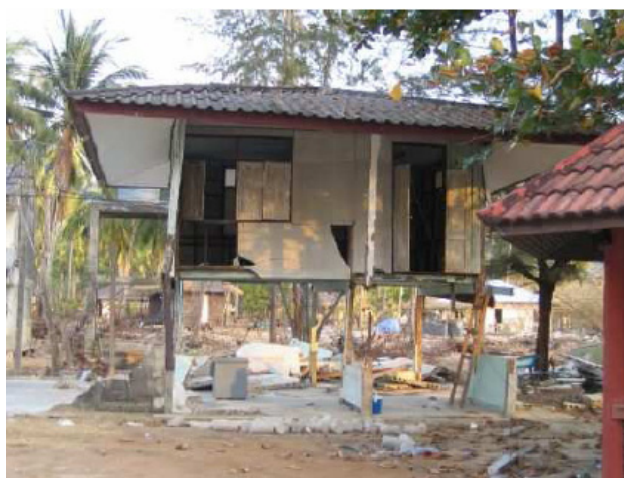
Figure 3. 26: Timber frame structure in near collapse damage state located approximately 100m from the shore line at Kamala Beach.
