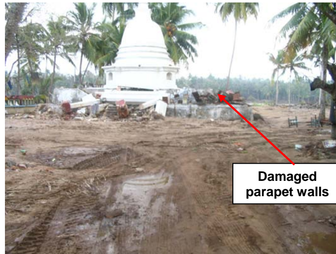
Figure 2.32: Damaged parapet walls and columns at the Buddhist temple located about 800m from the coastline
