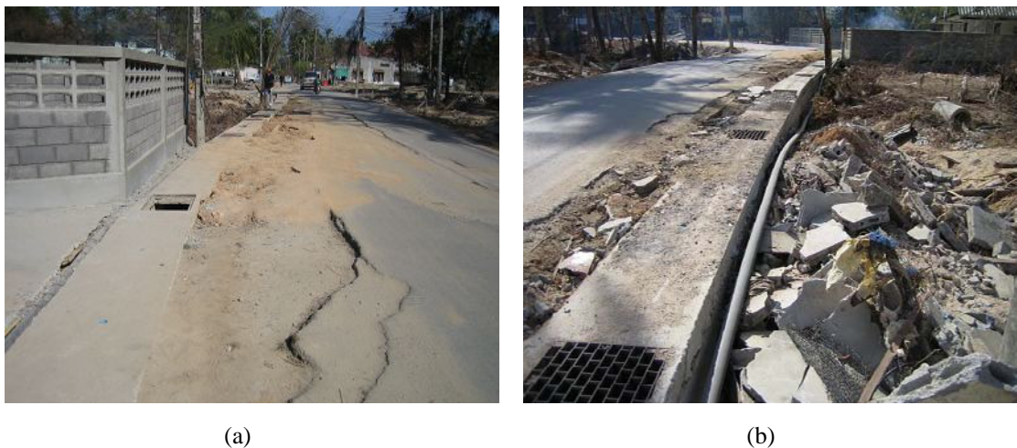
Figure 3. 41: Road damage near Bang Thao Beach, approximately 120m inland.
