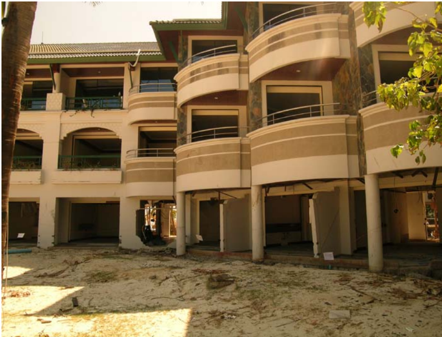
Figure 3. 22: The Cabana Resort on Phi Phi Island. Although this resort was close to the beach, it was at the western end and therefore probably more sheltered. Structural damage is restricted to windows on the lower two storeys and a few masonry panels on the ground floor.
