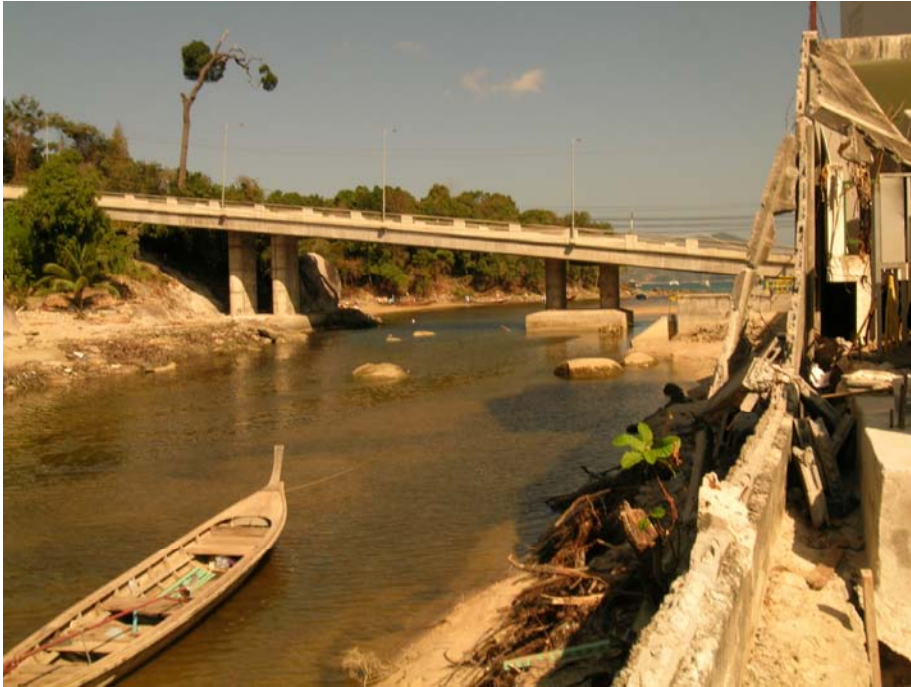
Figure 3. 43: No damage was observed on the cross-river bridge at the south of Patong Beach, however the pile caps under the piers have been partially exposed by erosion.
