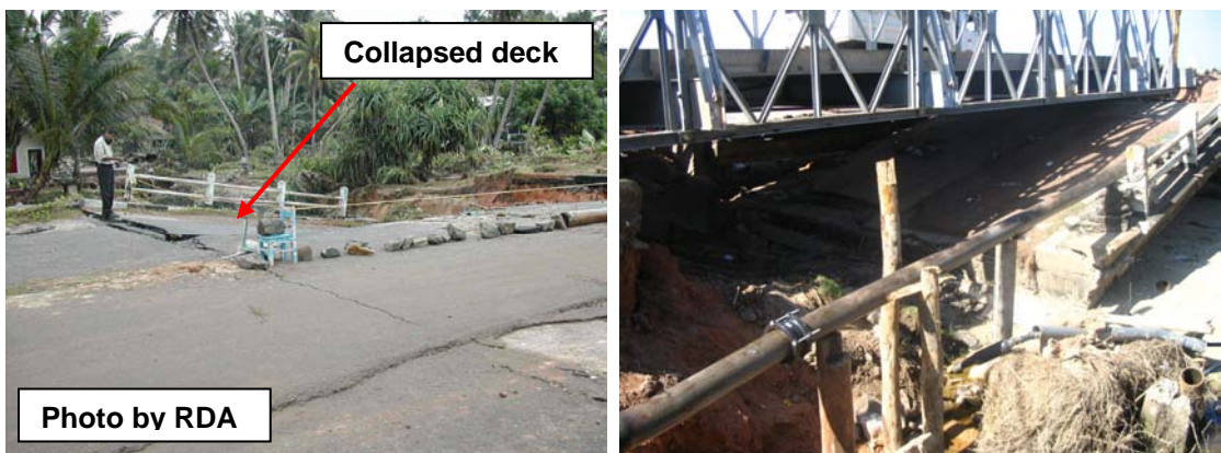
Figure 2.62: Collapsed southbound carriage of Goviyapana bridge (Type 1). Collapse due to erosion and scour damage to the abutment on the landward side. Temporary Bailey bridge in place to restore the carriage way
