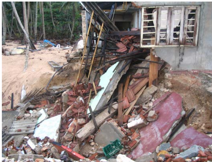
Figure 2.27: Collapse of part of the Cat. C masonry structure to a scour hole in Kahawa
