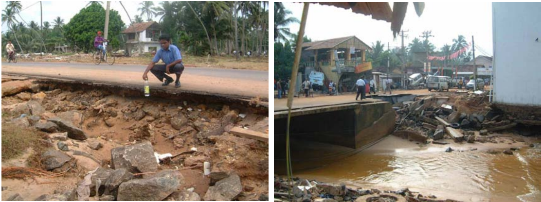
Figure 2.53: Light scour damage at the roadside exposed to the sea (Photo by RDA). Collapse of part of the road in Hikkaduwa due to scour in the exposed side to the sea (photo provided by Dennis Knight, Halcrow-Sri Lanka)
