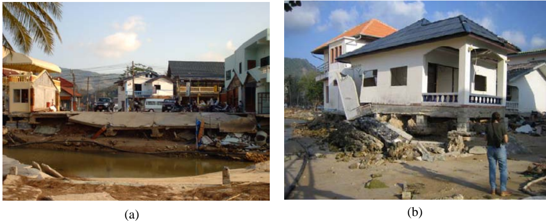
Figure 3. 40: Photographs of building damage at Kamala Beach taken at survey locations 1 and 2 shown on Figure 3.39: (a) taken at location 1, shows the sea wall failure at Kamala caused by beach erosion, (b) the footings of the house at location 2 are left exposed by the erosion caused by the tsunami.
