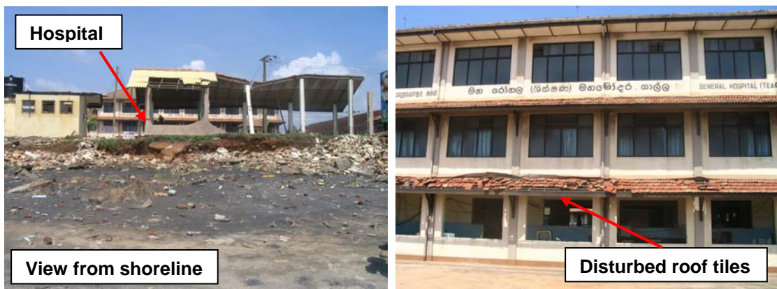
Figure 2.74: Mahamodara hospital (Galle) suffered moderate damage but lost equipment in the ground floor due to inundation
