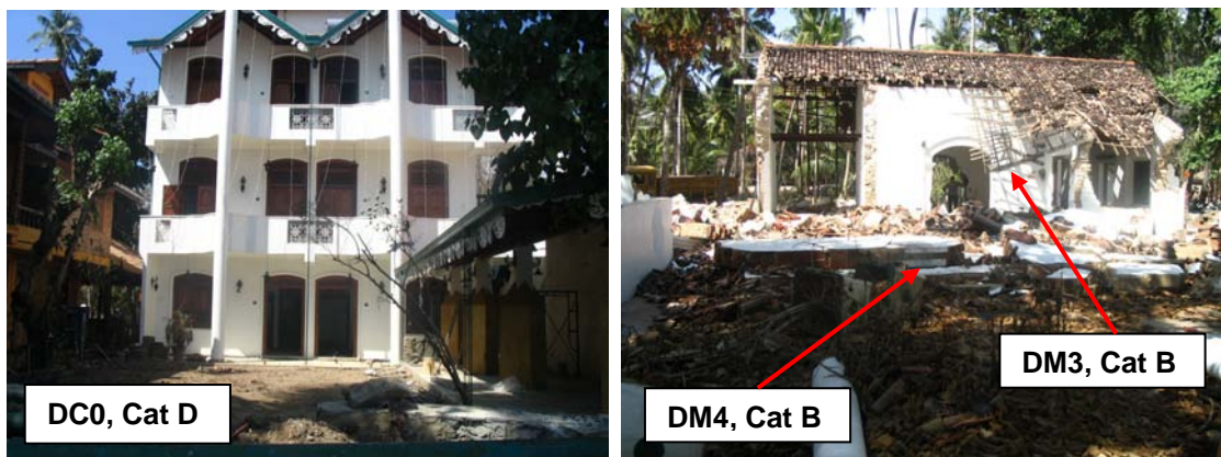
Figure 2.39: Undamaged hotel 20m from the shoreline. Collapse and heavy damage to a Cat B masonry house at the same distance
