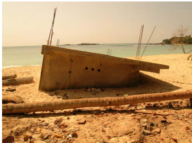
Figure 2.6: Evidence of Liquefaction damage to a small public utility building in Unawatuna (Galle District)
