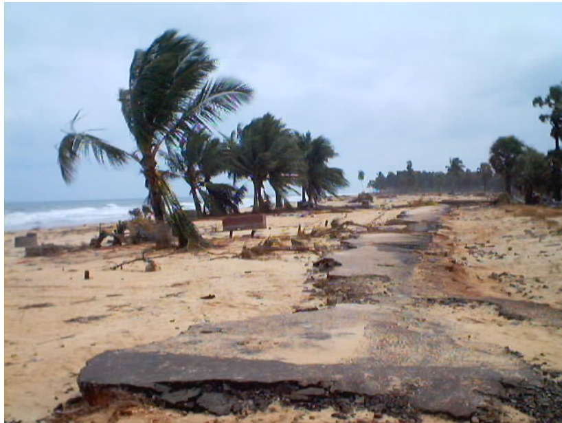
Figure 2.56: Typical heavily damaged road section near Batticaloa (Photo by Anton Pillai, Arup)
