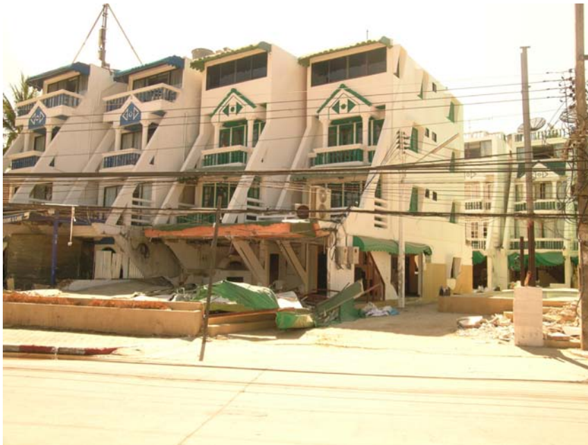
Figure 3. 4 Heavily damaged ground floor infill walls and columns of the Patong Swiss Hotel on Thaweewong Road, located about 90m from the sea front .
