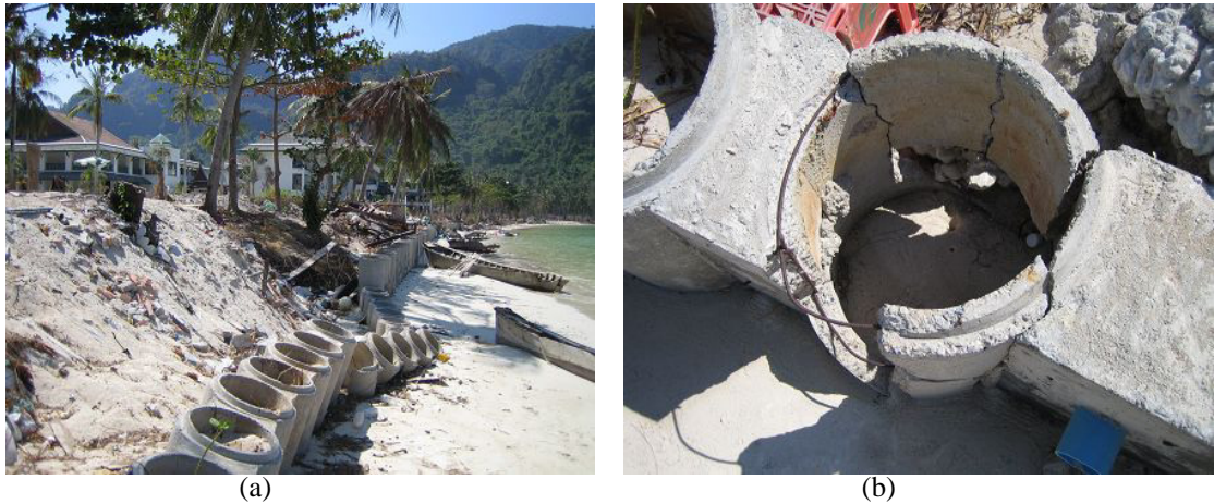
Figure 3. 45: Damaged 500mm inner diameter gravity retaining sea wall with sand infill on Loh Dalam Bay in Phi Phi Island located at approximately 10m from the coastline.
