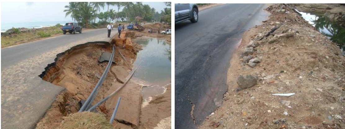
Figure 2.55: Collapsed section of Road A2 in Kahawa due to scouring on the exposed land side (Photo by RDA) and the state after repair as observed by EEFIT
