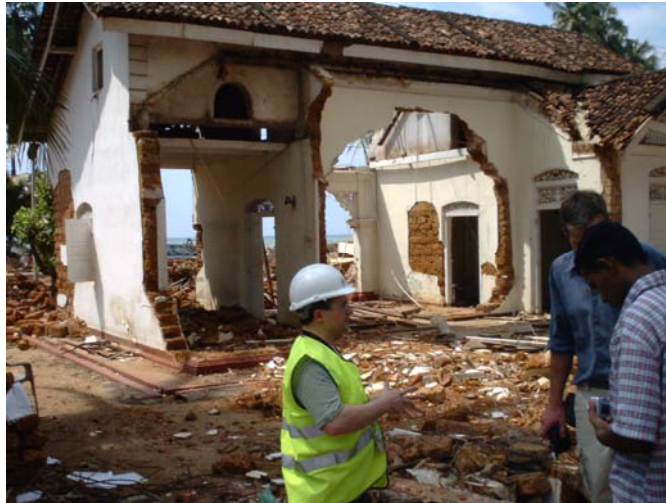
Figure 2.2: Typical damage to brick masonry walls parallel to the coastline, observed in Paiyagala (Kalutara District)
