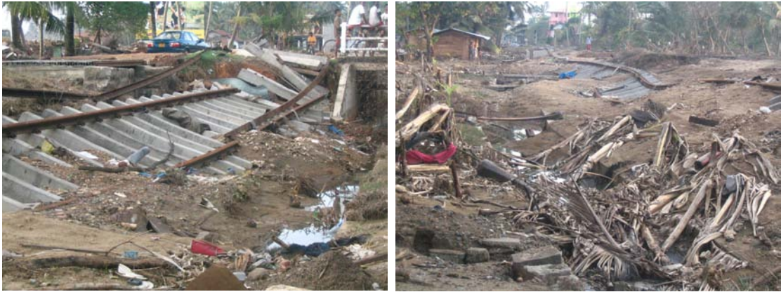
Figure 2.57: Damaged section of railroad near Hikkaduwa due to collapse of the embankment possibly driven by erosion and scouring
