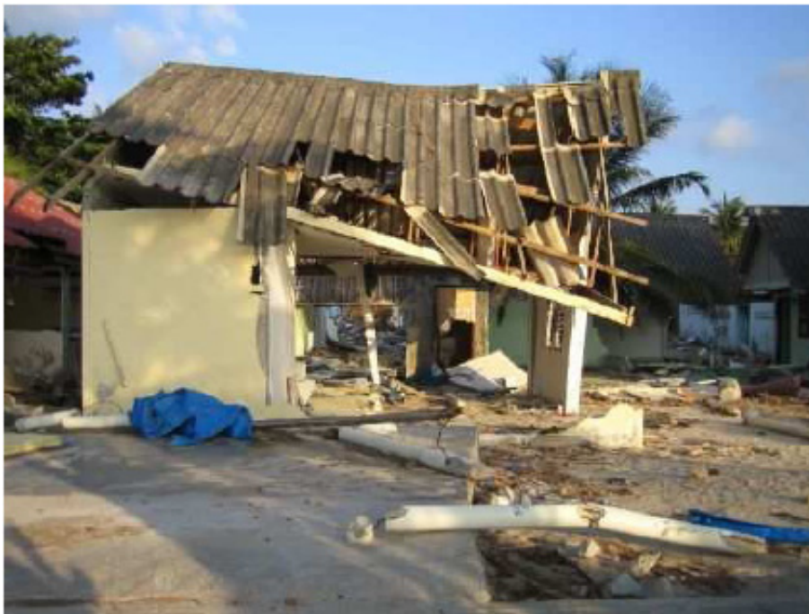
Figure 3. 6: Seriously damaged single storey house located 100m from the shore line at Kamala Beach. Example of typical timber roof system and its poor connection to the supporting structure.
