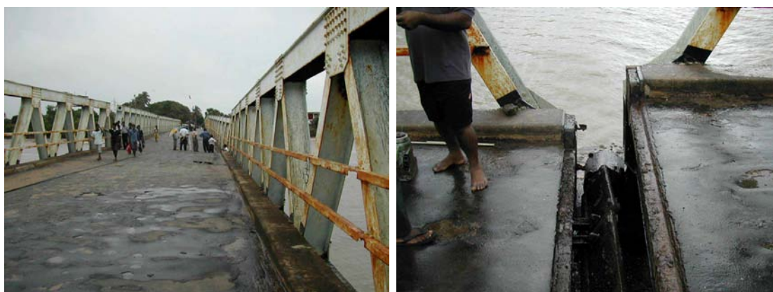
Figure 2.67: Severe distortions to the Arugambe bridge due to tsunami impact and foundation settlement and shearing at the connections to the piers (Photos by RDA)
