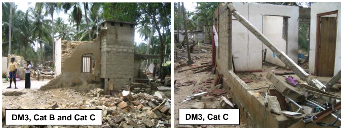
Figure 2.30: Heavily damaged (DM3) masonry structures at about 300m from the coastline in Peraliya
