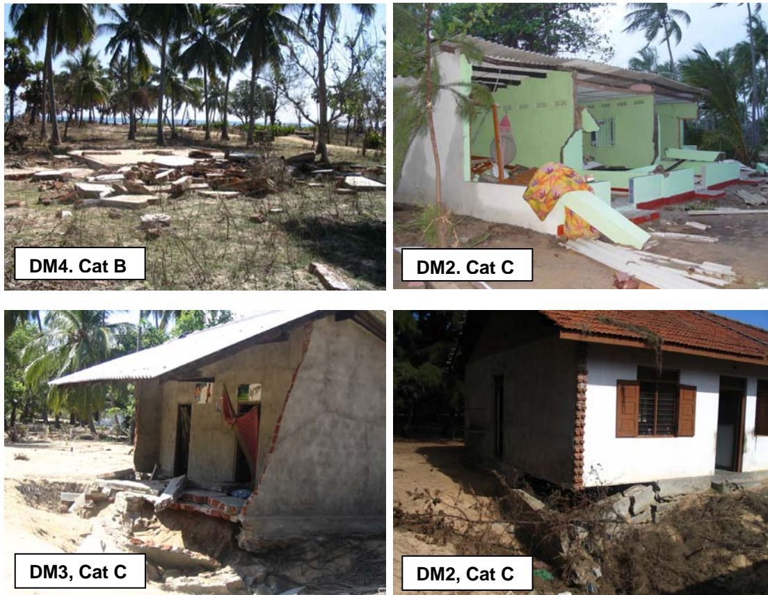
Figure 2.49: Typical damage to masonry houses in Eastern and Northeast Provinces (Pillai, 2005)
