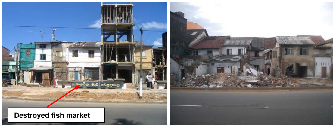
Figure 2.37: Damaged commercial buildings behind Galle Harbour on Road A2
