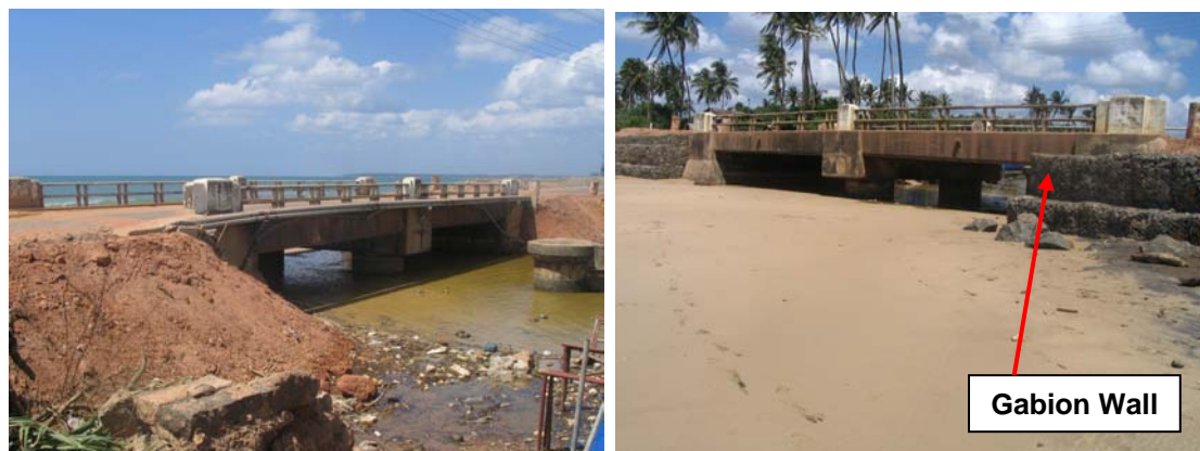
Figure 2.64: Damage to Devundara (Dondra) bridge (Type 1) approaches. Approaches restored and gabion protection wall constructed on the side exposed to the sea
