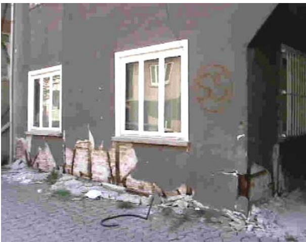
Figure 5.10: Damage to Himis house caused by soil failure
