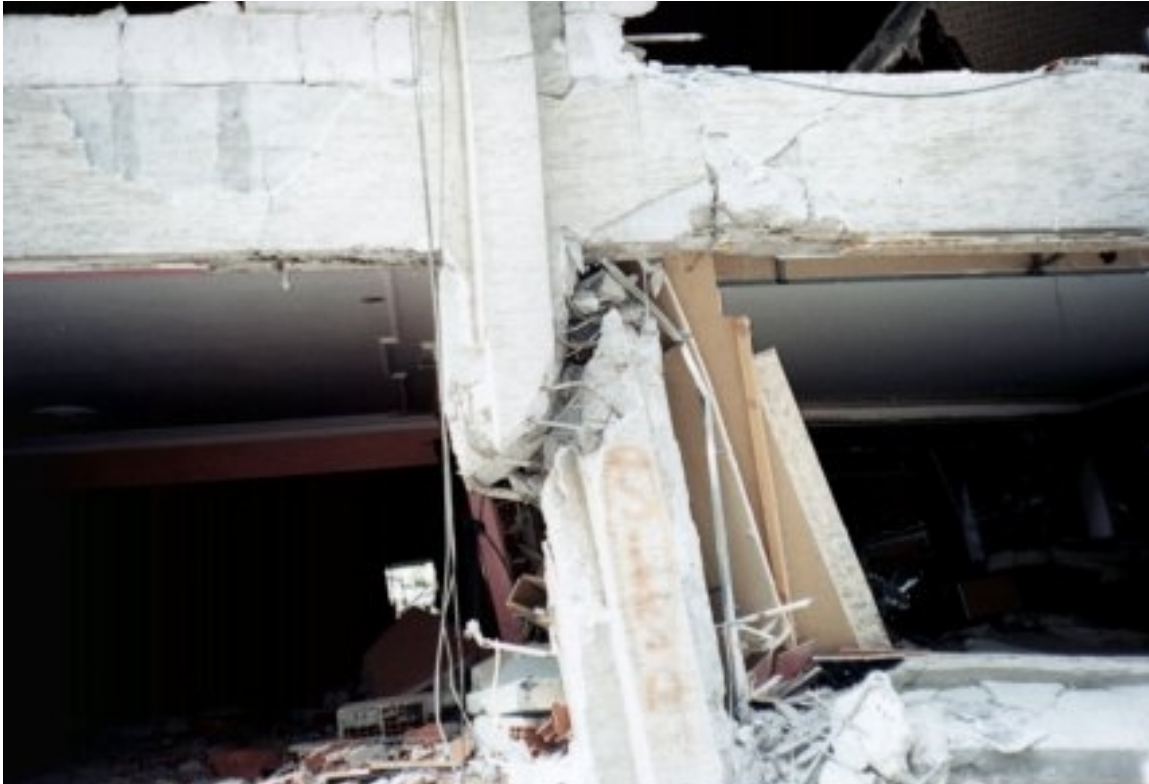
Figure 5.31: Shear failure of ground floor column
