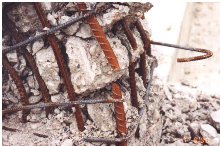
Figure 6.4c: Detail of failed connection at base of columns. Note the ruptured longitudinal bars
