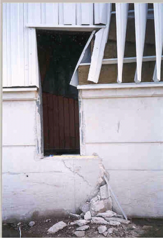
Plate 4.9 Ford Otosan, Gölcük Plant Body Shop west wall. Failure and closure of door in west wall illustrates compression in north-south direction of approximately 400mm (photograph taken on 5 September 1999).
