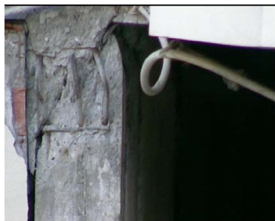
Figure 5.30: Shear failure in column
