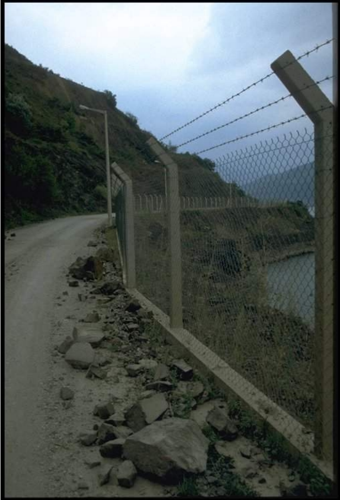
Plate 4.23 Minor rockfall debris observed on the road to Yuvacik Dam.
