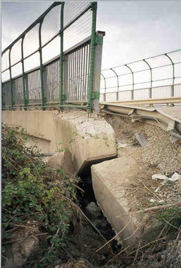
Plate 4.33 Differential settlement of approach embankment and damage to bridge abutment on access road to Toyota Factory outside Adapazari (photograph taken on 8 September 1999).
