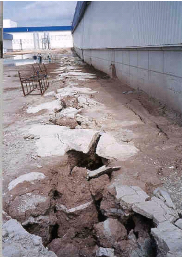
Plate 4.8 Ford Otosan, Gölcük Plant Body Shop west wall. View from southwest corner looking north. Fissure in ground has formed along alignment of cement grout columns, which were installed across the site as ground improvement to increase bearing capacity and resist liquefaction susceptibility. Note differential settlement distortion of wall (photograph taken 5 September 1999).
