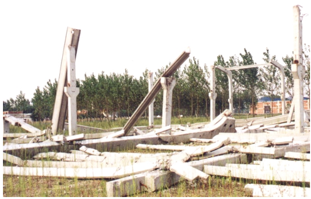
Figure 6.6b: Typical failure pattern
