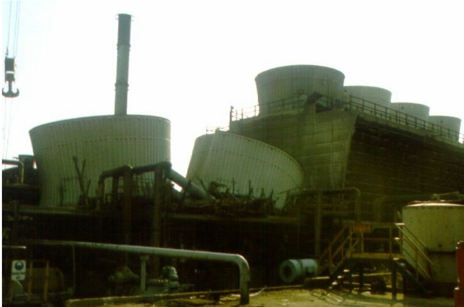
Figure 6.22: Collapsed Wooden Cooling Towers at Petkim
