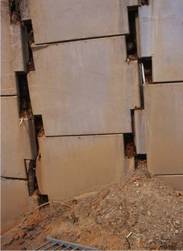
Plate 4.31 Reinforced earth wall for E80 highway approach ramp at Arifiye. Damage to wall panels on the eastern side of the ramp. The ramp on the left side has settled with respect to that on the right. Opening of panel joints has been exacerbated by the horizontal distortion of the ramp about a 'hinge point' on the opposite side of the ramp.
