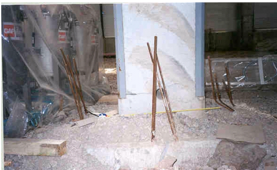
Figure 6.30a: Column Damage in Bodyshop
