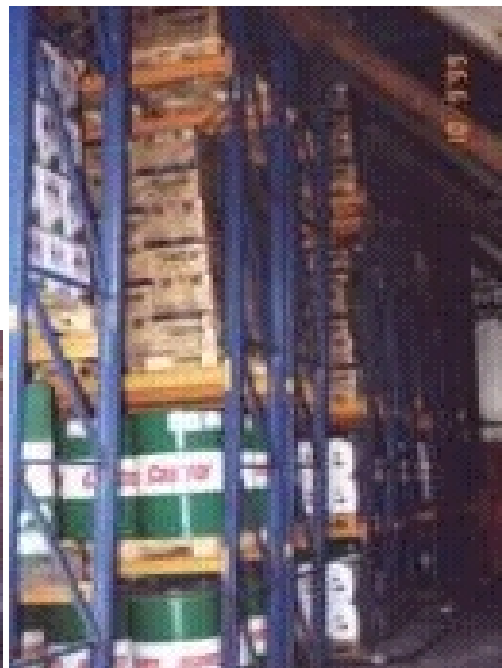
Fig 6.21c: Racking tilted over. Note new props in top right corner
