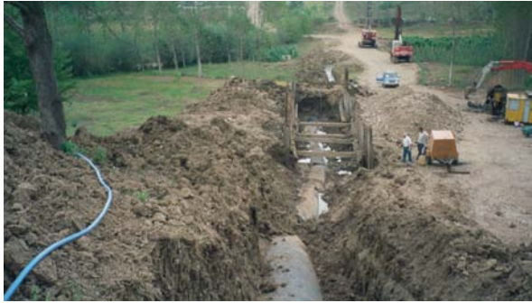
Figure 7.22: Damaged run of pipeline in a region of high ground disturbance
