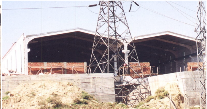
Figure 6.14.b: Failure of cladding – factory near Korfez. The EOT crane in this building needed to be replaced post earthquake.
