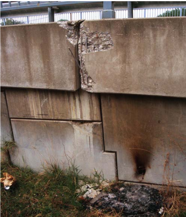
Plate 4.32 Reinforced earth wall for E80 highway approach ramp at Arifiye. Pounding damage to cope units.
