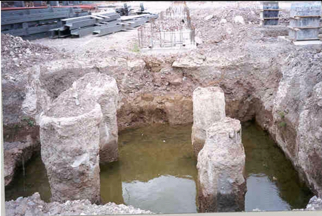
Plate 6.1: Ford Otosan Plant, Golcuk. Press Shop under construction. View to west of pile cap excavation showing 4 pile group of 600 to 700 mm diameter piles at 2000 mm centres. Main reinforcement is 10 number 16mm deformed steel bars. Confining steel is 10 mm deformed steel with unknown pitch (5 September 1999).
