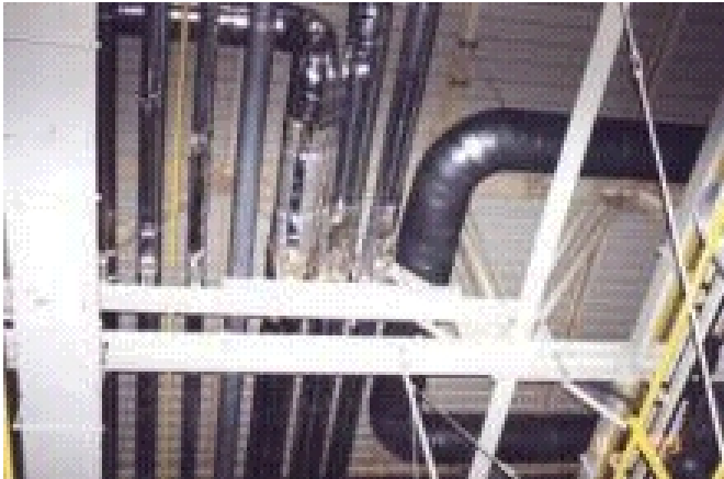
Figure 6.24: Services run in the roof
