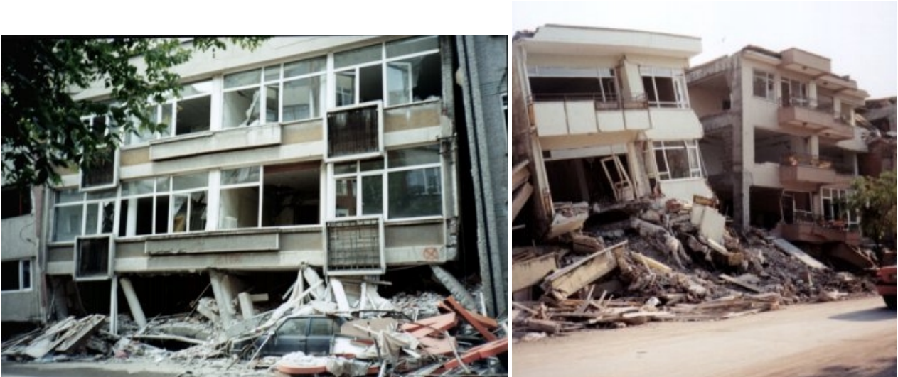
Figure 5.17: Buildings in Cark Cad., Adapazari for which the lower 2 storeys columns had collapsed.
