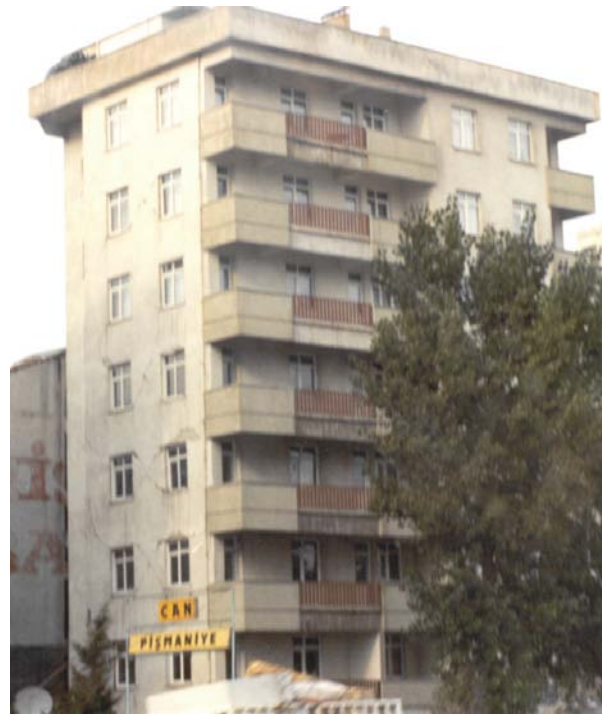
Figure 5.28b: X cracks in the lateral wall between opening
