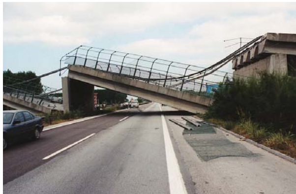
Figure 7.3: Collapsed bridge on E80 highway (photo: N.Apaydin)
