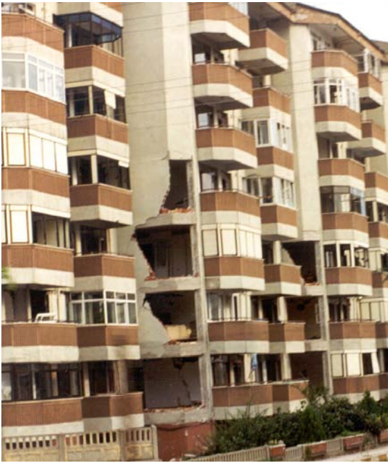
Figure 5.28a: Composite diagonal and out of plane failure of infill
