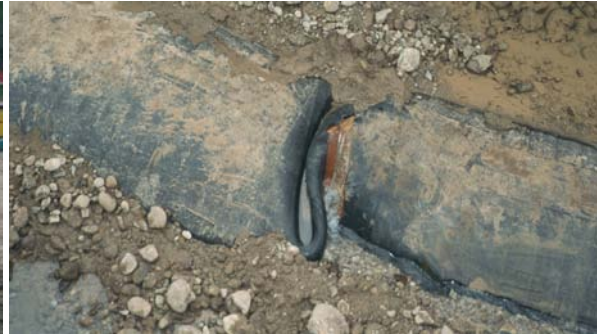
Figure 7.23: Local distortion of pipe due to displacement imposed by ground movement
