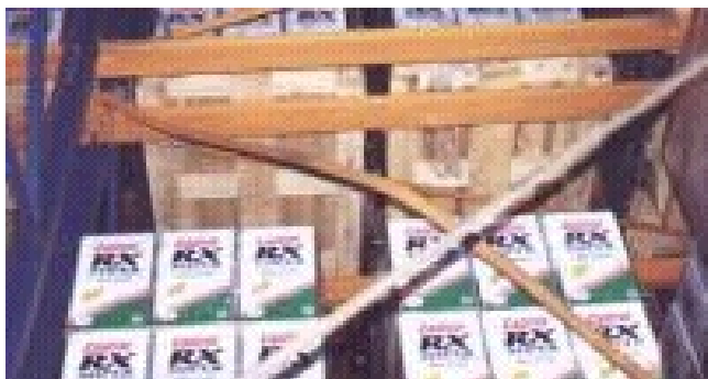
Fig 6.21b: Buckling of bracing to racking system. Diagonal from bottom left to top right is new bracing installed post earthquake
