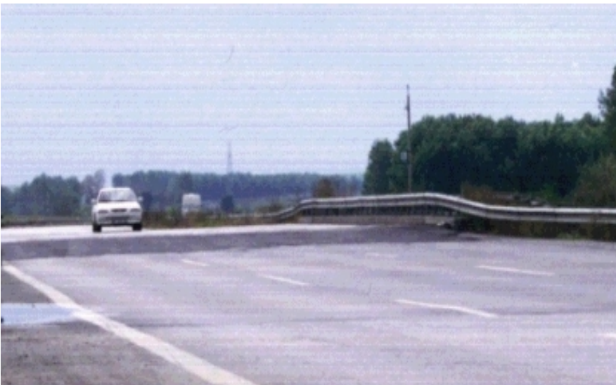
Plate 4.34 Differential settlement of earth embankment on-ramp and off-ramp to highway bridges formed bump-on and bump-off structures .
