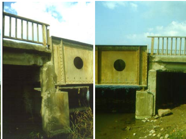
Figure 7.13 Pounding Damage to Supports
