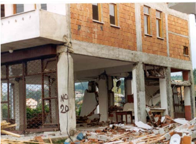
Figure 5.29: Hinges forming at bottom and top of columns.
