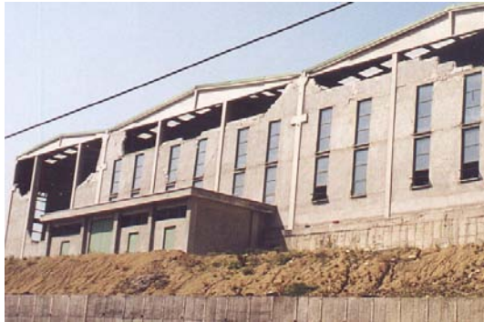
Figure 6.14a: Failure of cladding – factory near Korfez
