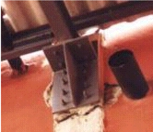
Fig 6.20c: Near failure of connection for canopy roof connecting two buildings
