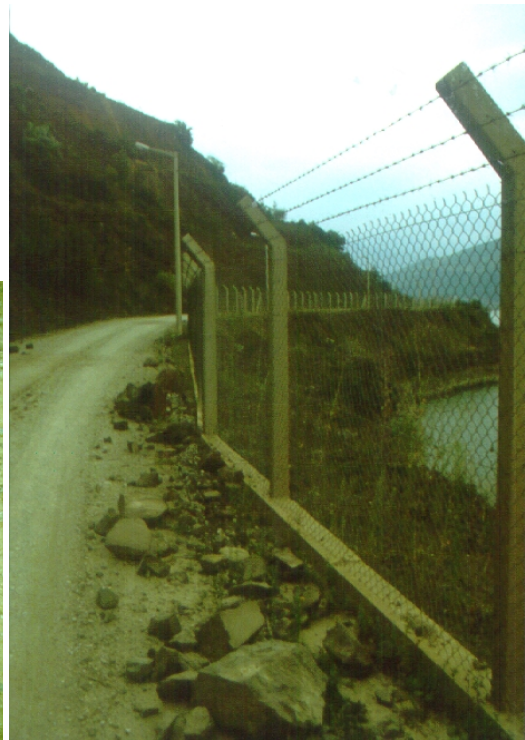
Figure 7.21 Small Rockfall Adjacent to it
