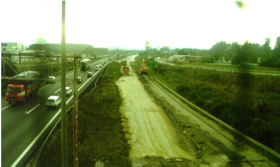
Figure 7.5: Road repair resulting from fault rupture
