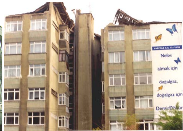
Figure 5.27b: Roof failure in a 8- storey building in Izmit
