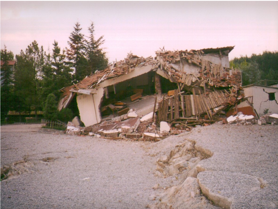
Plate 4.10 Fault rupture at Yuvacik bisected school building causing collapse. At this location the fault was divided into two ruptures oriented 285^\circ with a central graben 5m to 8m wide. The main rupture had 1.5m right lateral offset and 0.7m vertical offset (photograph taken on 18 September 1999).
