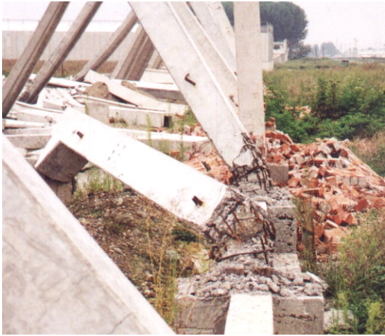
Figure 6.4a: Typical failure of main columns
