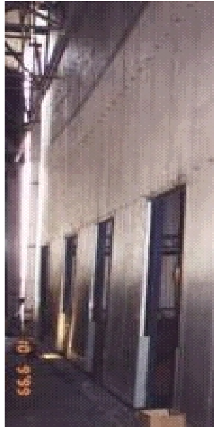
Fig 6.21a: Tilt of warehouse when compared to adjacent loading bay
