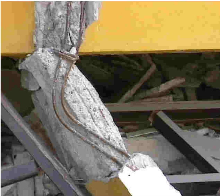
Figure 5.5a: Slender column, lack of bonding and absence of stirrups
