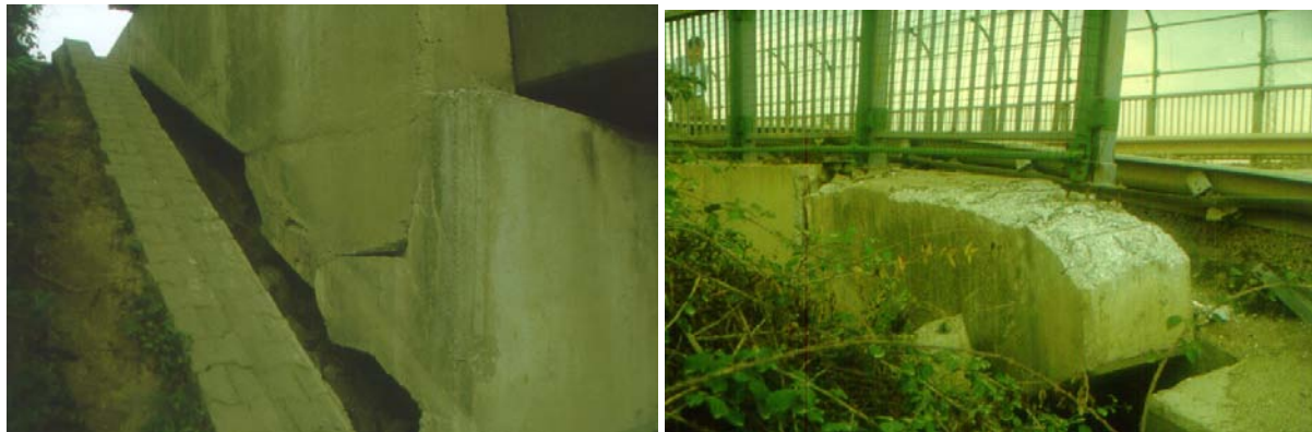
Figures 7.6, 7.7: Movement of overpass abutment and of road bridge abutment close to fault rupture
