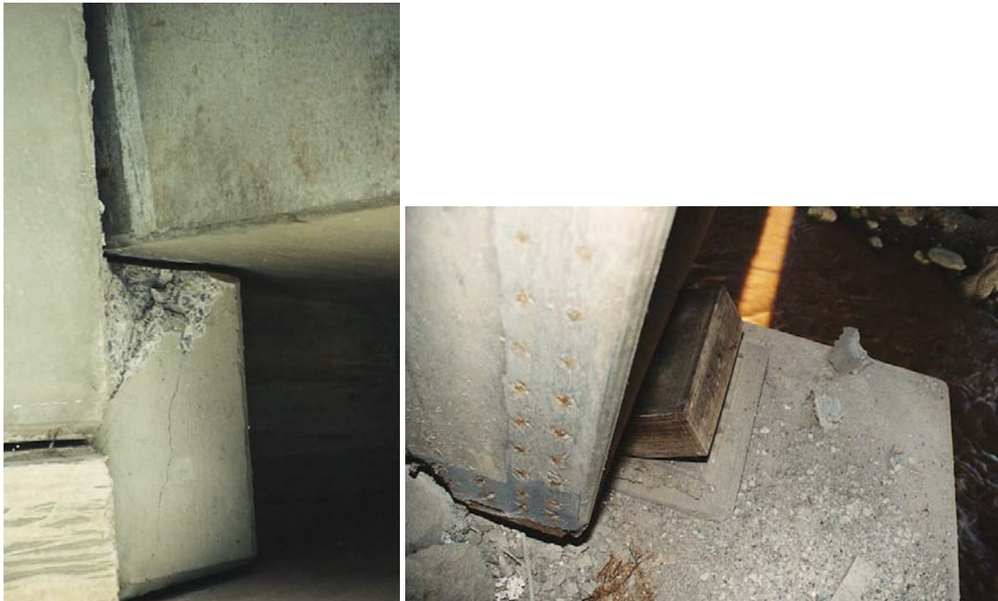
Figures 7.8, 7.9: Spalling and damage to bearing pad at seat of bridge deck (photo: N.Apaydin, H.Aydin)
