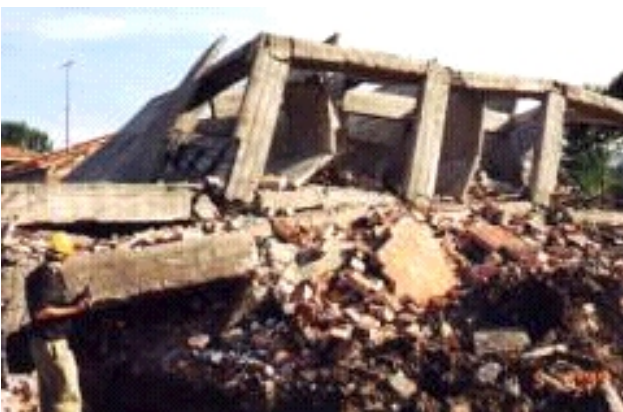
Figure 5.16a: Overturning of the frame with loss of infill
