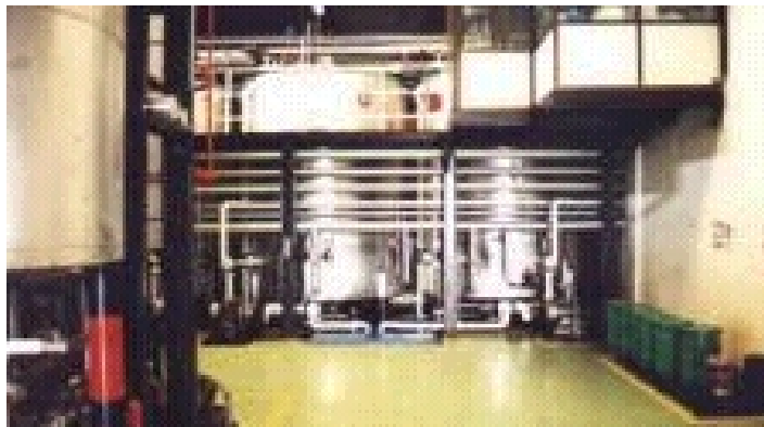
Fig 6.20a: Main processing area. Steel frame, and process plant undamaged
