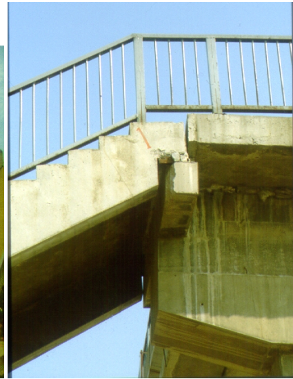
Figure 7.15: Detail of damage to the access staircase
