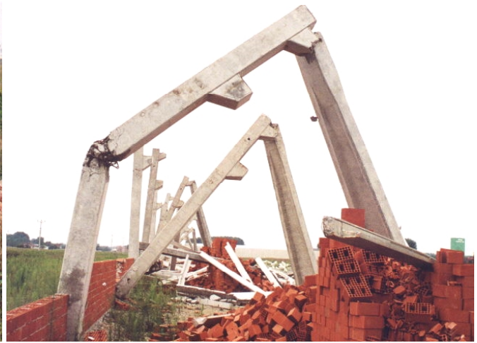
Figure 6.4b: Failure of main columns with part built external cladding
