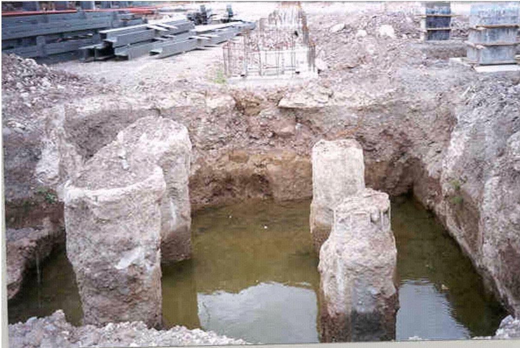
Plate 4.1 Ford Otosan, Gölcük Plant Press Shop under construction. View to west of pile cap excavation showing 1.2 m of reddish brown gravelly sand fill overlying loose alluvial sand. Evidence of jet grouting at site can also be seen. Foundations comprise four-pile groups with 600 to 700 mm diameter piles at 2000 mm centres. Main reinforcement is 10 number 16mm deformed steel bars and confining steel is 10 mm deformed steel. (photograph taken on 5 September 1999).
