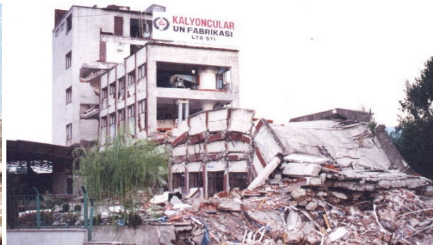
Figure 6.13b: Failure of RC factory south Marmara Sea area
