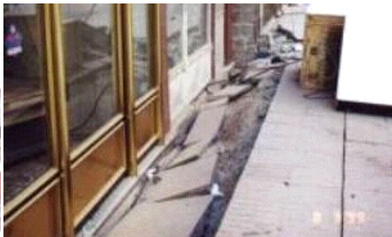
Figure 5.23b: Soil failure. The building is undamaged
