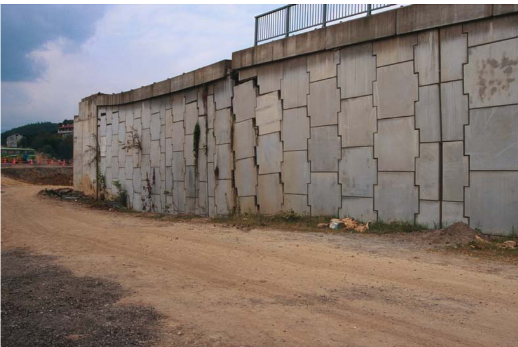
Plate 4.30 Reinforced earth wall for E80 highway approach ramp at Arifiye. View toward the southwest. Culvert crosses the ramp beneath the nearer end of the damaged coping units. Vertical movement joints in the panels run up from the edges of the culvert.
