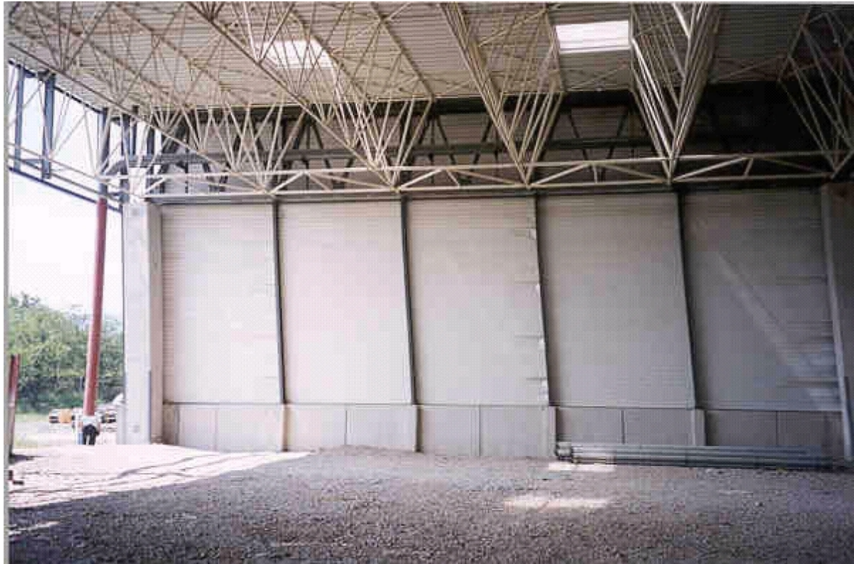
Figure 6.30b: Bodyshop west wall showing distortion of columns. Roof has kept its shape and pipe work from roof clearly shows horizontal displacement.
