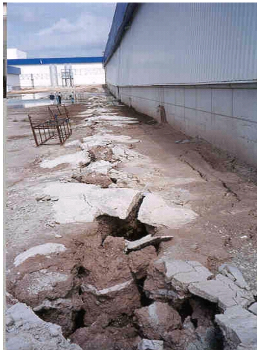
Figure 6.30c: Fissure in ground formed along alignment of cement grout columns.
