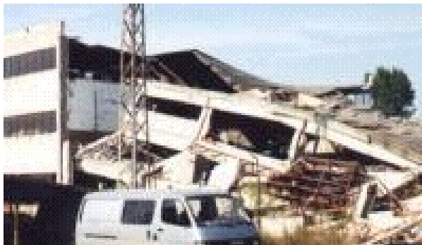
Figure 6.13a Failure of in-situ concrete and steel roof trussed factory near Yuvacik
