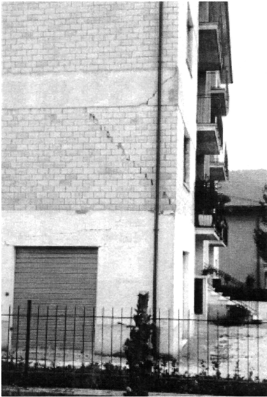
Plate 2.35: Building damage: Nocera SMI site
