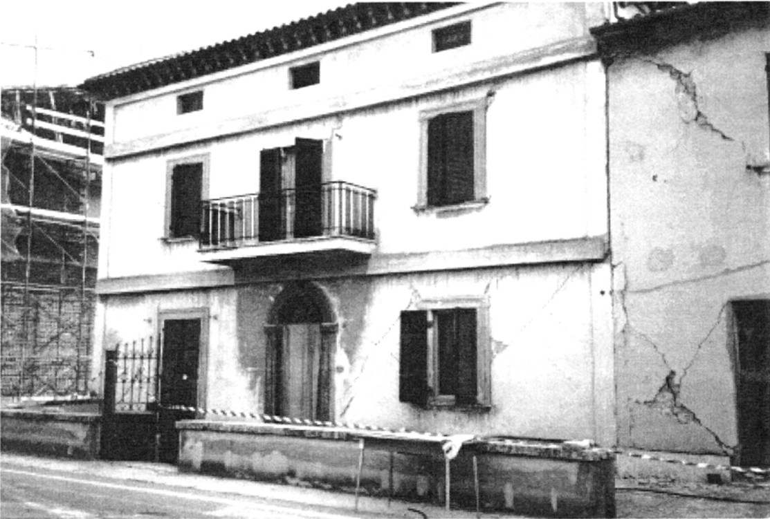
Plate 2.20: Shear failure in lower and upper storey walls: Nocera Scalo
