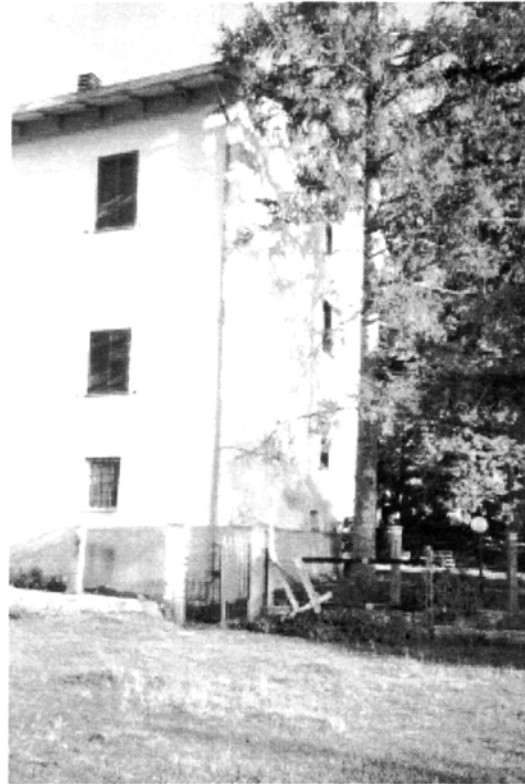
Plate 2.32: Damage to farmhouse: Colfiorito SMI site
