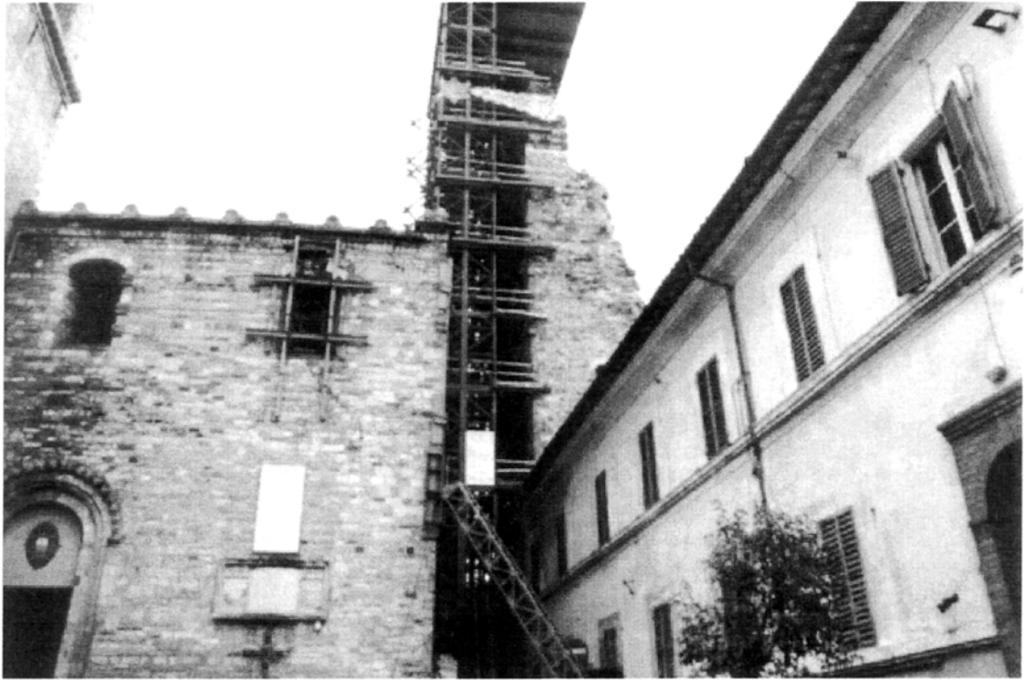
Plate 3.31: Nocera Umbra: shoring work after the collapse of the Civic Tower (right) and urgent repair measures to the Cathedral
