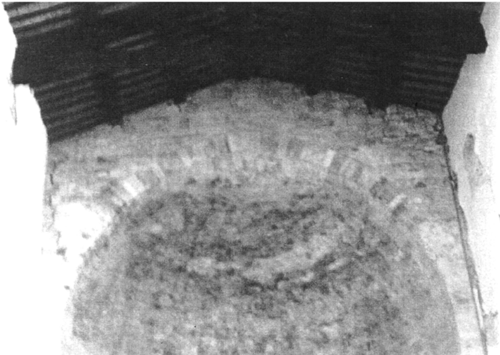
Plate 3.24: Santa Maria Maggiore: vertical crack at connection between apse and lateral walls
