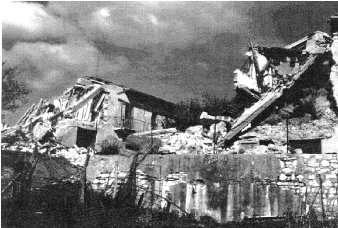
Plate 2.11: Collapsed buildings with modifications in newer masonry
