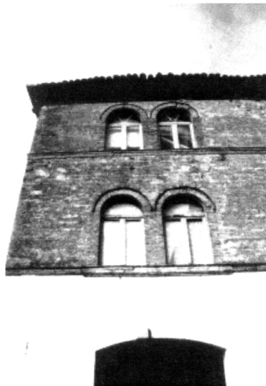
Plate 3.38: Nocera Umbra: central sub vertical cracks in building opposite San Filippo church, associated with ground movement
