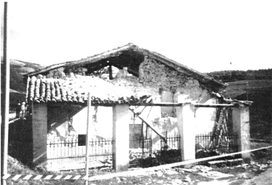
Plate 2.24: Masonry wall peeling: Cesi
