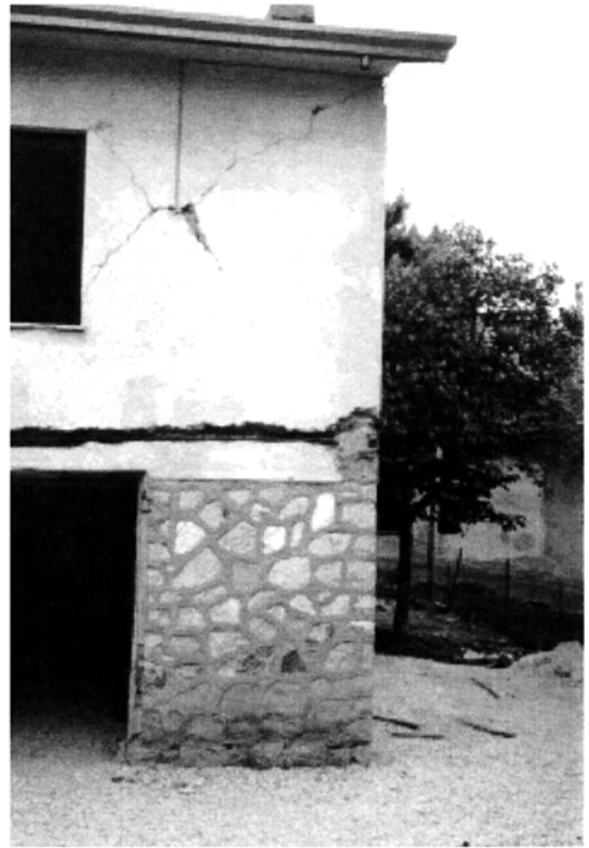
Plate 2.36: Building damage: Nocera SMI site
