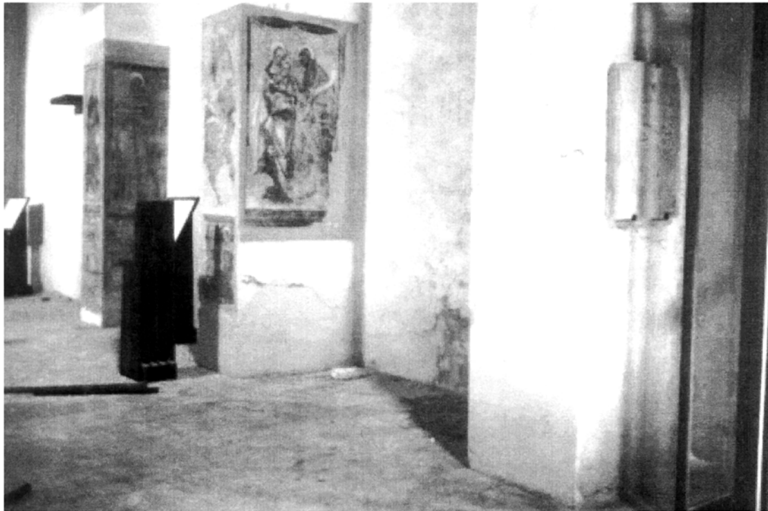
Plate 3.33: Pinacoteca, Nocera Umbra: horizontal cracks at the base of columns
