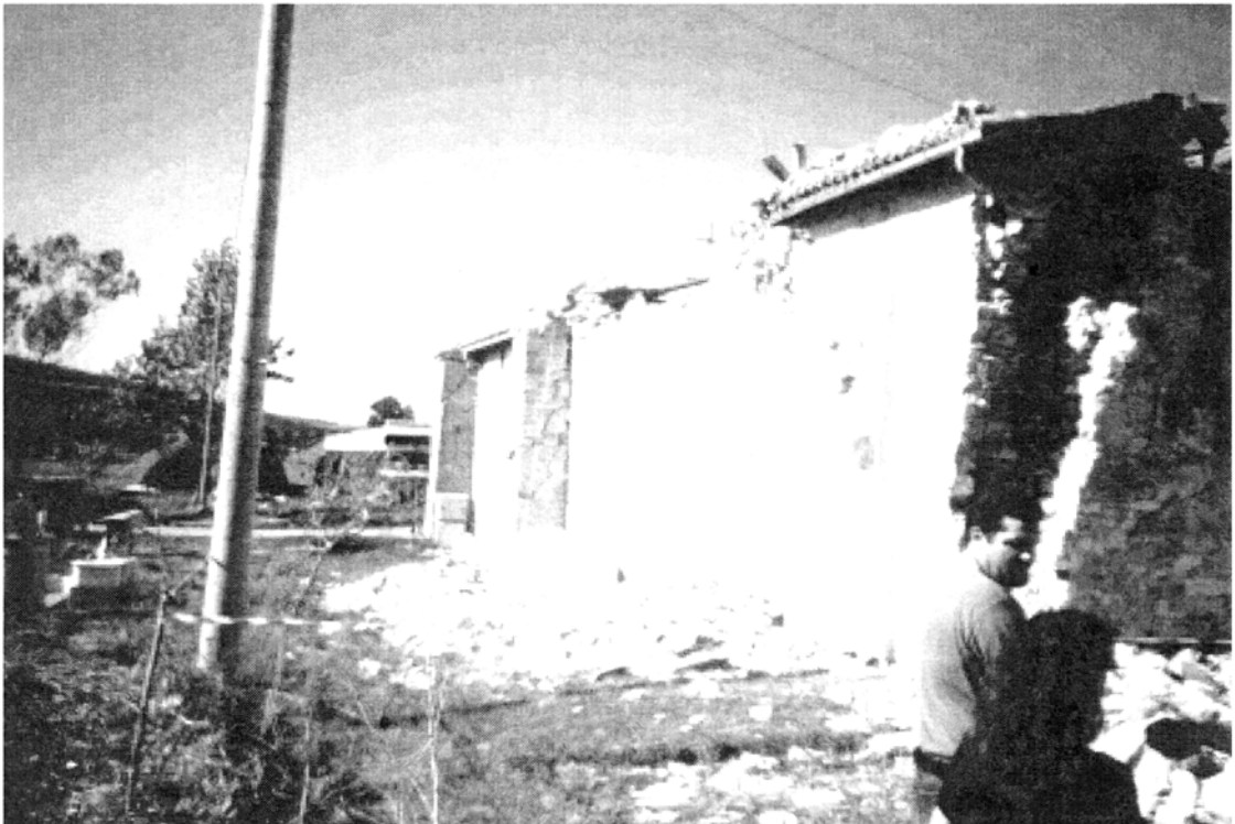
Plate 2.26: Shear cracking in buttress of church: Cesi
