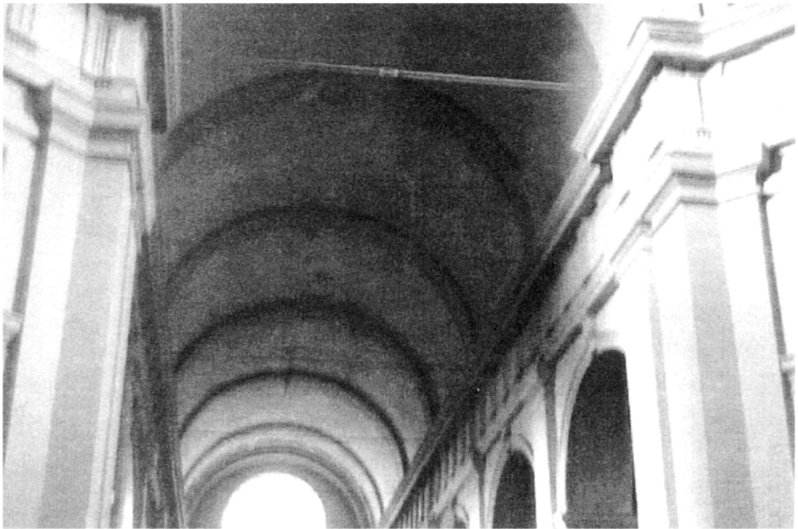
Plate 3.19: San Rufino Cathedral: longitudinal cracks along the intrados of the main nave barrel vault
