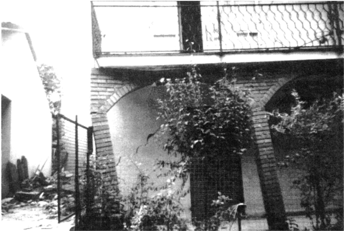
Plate 2.27: Column sideways failure mechanism: Isola
