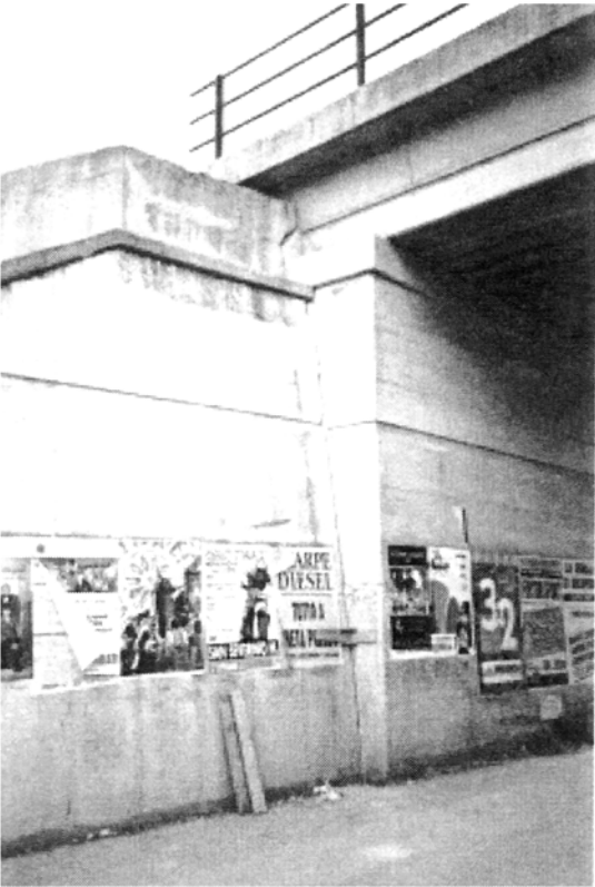
Plate 2.28: Embankment displacement: Isola
