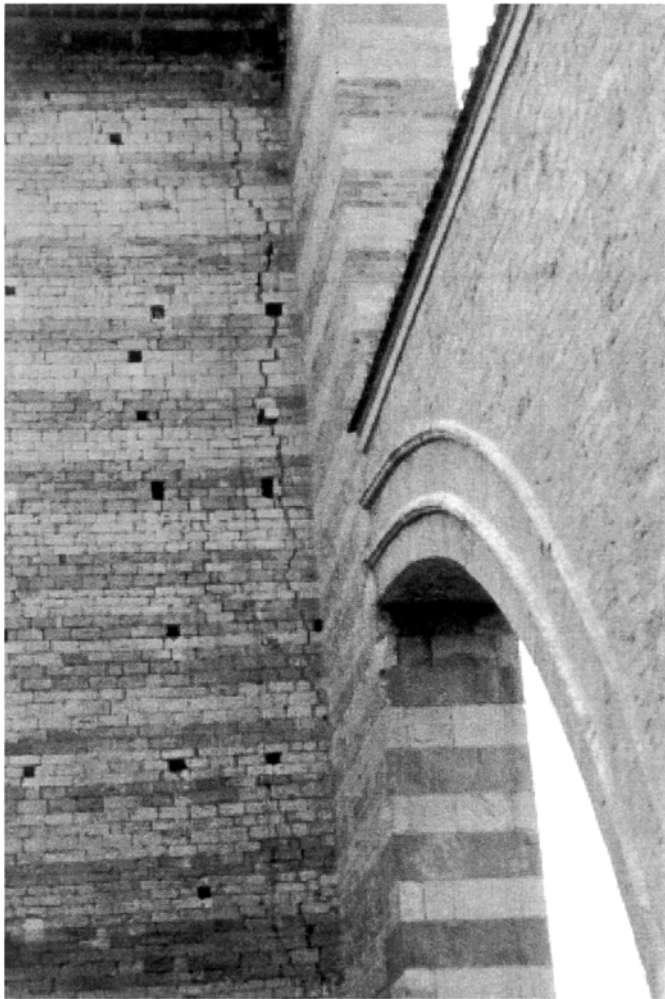
Plate 3.9: Santa Chiara Basilica: vertical cracks on the northern longitudinal wall
