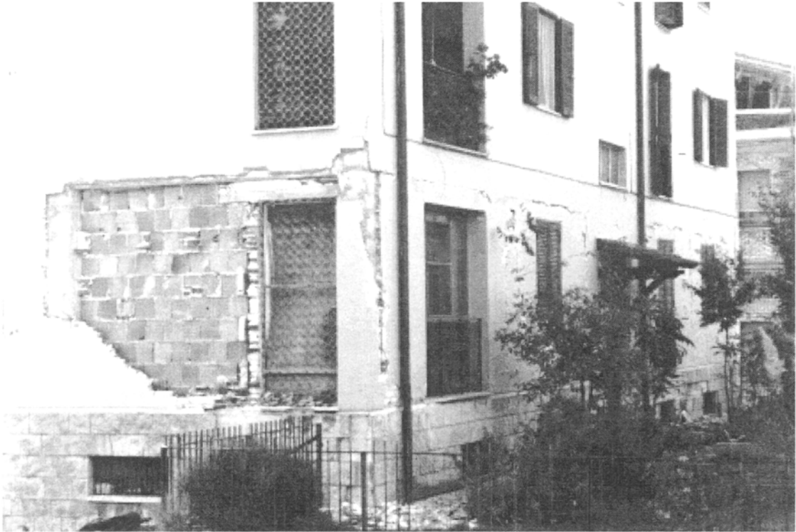
Plate 2.21: Failure of masonry infill in reinforced concrete frame building: Nocera Scalo
