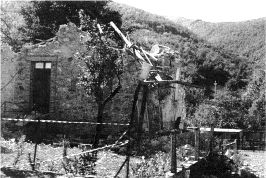
Plate 2.13: Partly collapsed unreinforced masonry building: Casenove
