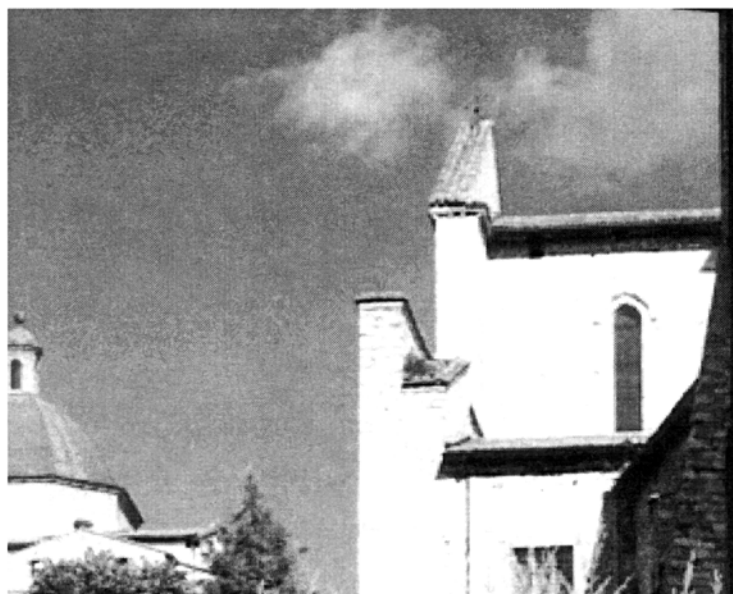
Plate 3.8: Santa Chiara Basilica: subvertical cracks on the southern longitudinal wall
