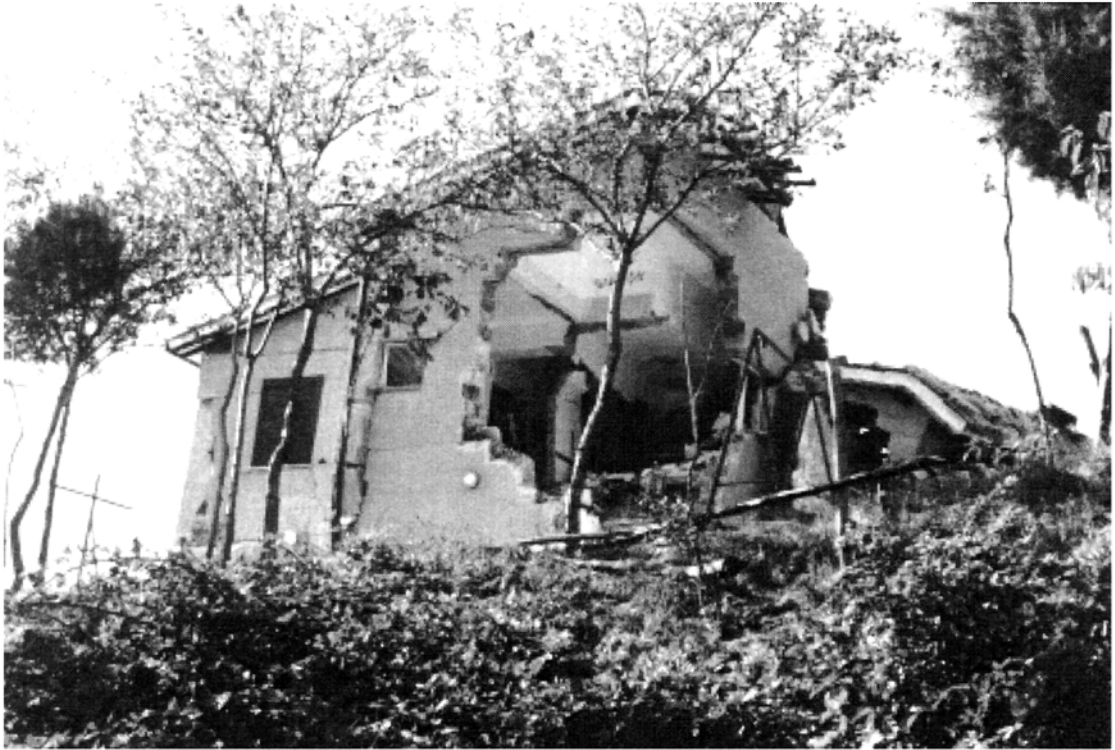
Plate 2.17: Clay block masonry with corner failure: Collecurti
