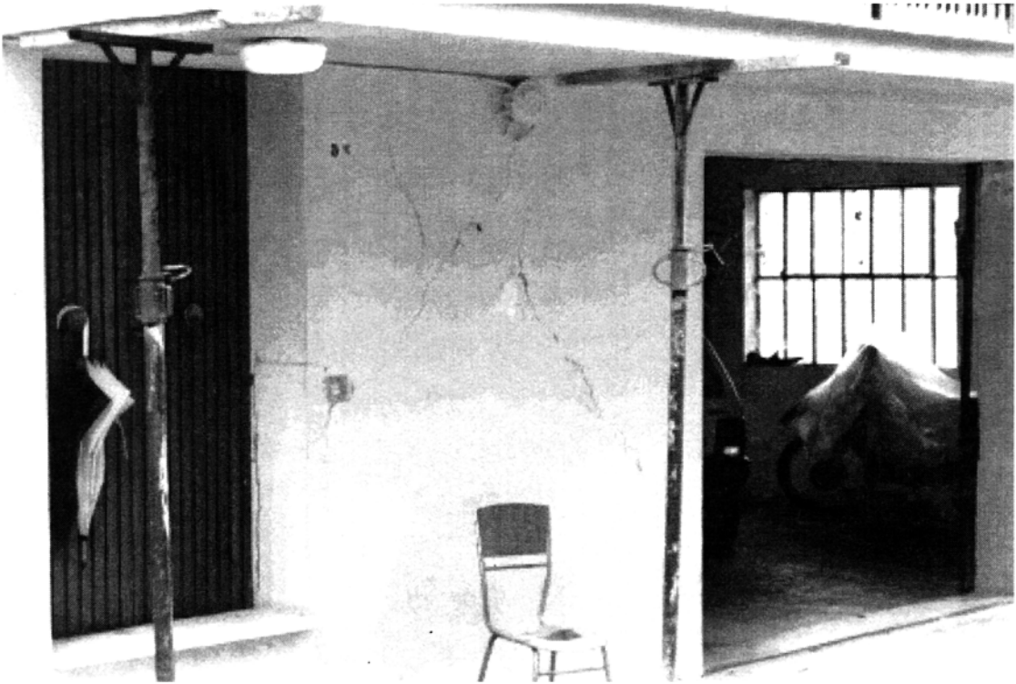
Plate 2.40: Building damage: Nocera SMI site
