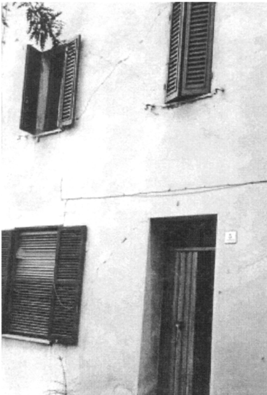
Plate 2.37: Building damage: Nocera SMI site
