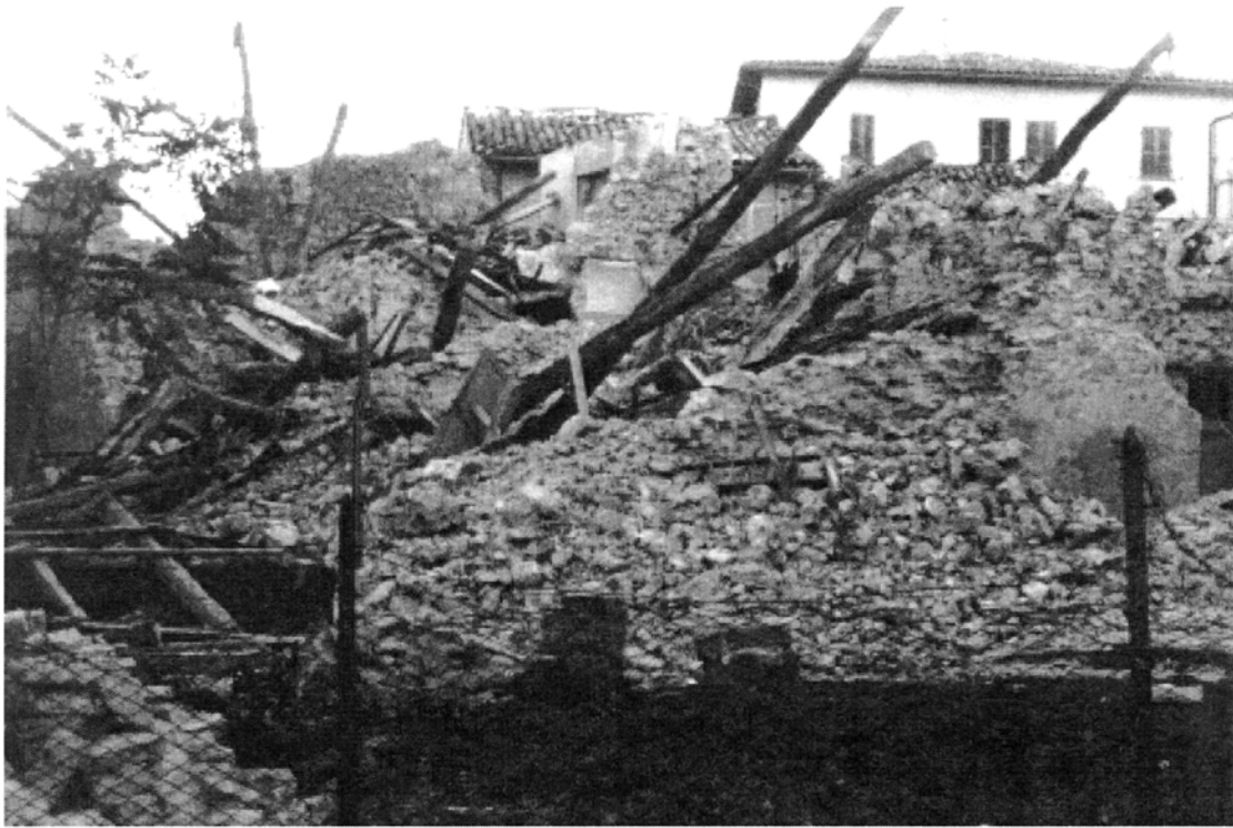
Plate 2.15: Totally collapsed unreinforced masonry building: Annifo
