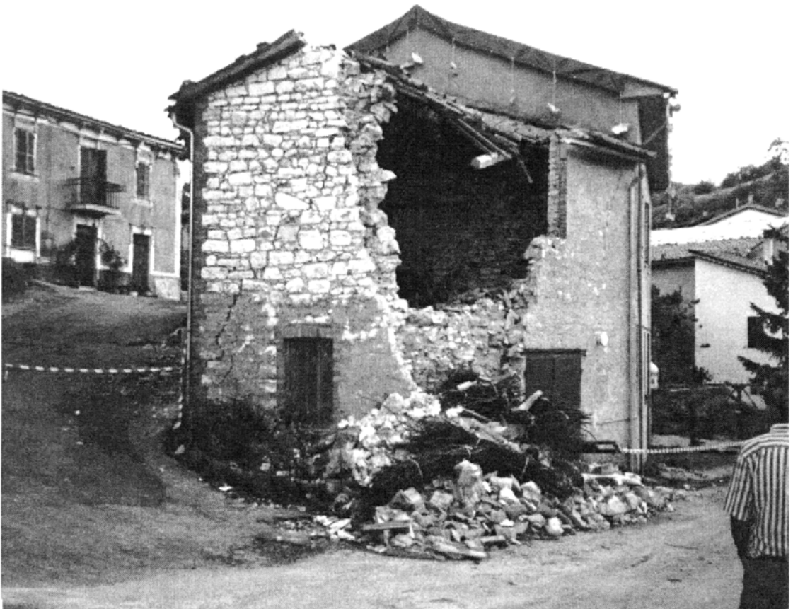
Plate 2.14: Partly collapsed unreinforced masonry building: Annifo
