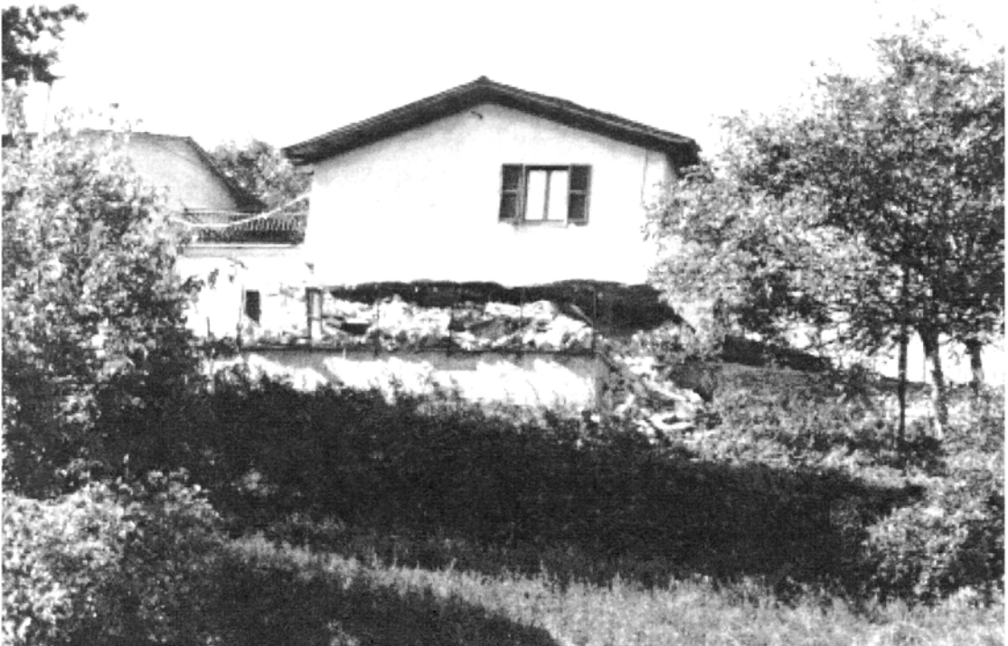
Plate 2.18: Failure of lower storey walls: Collecurti
