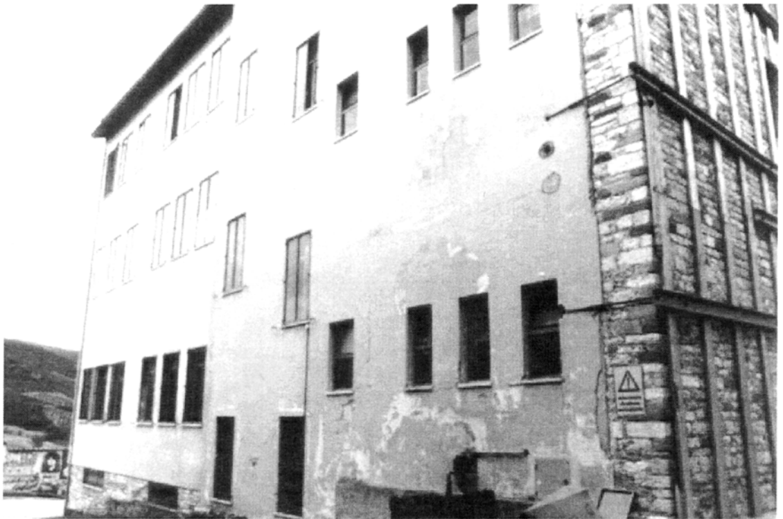
Plate 3.32: Comune, Nocera Umbra: detachment of perpendicular walls and shear cracks in infill panels within new reinforced concrete structure
