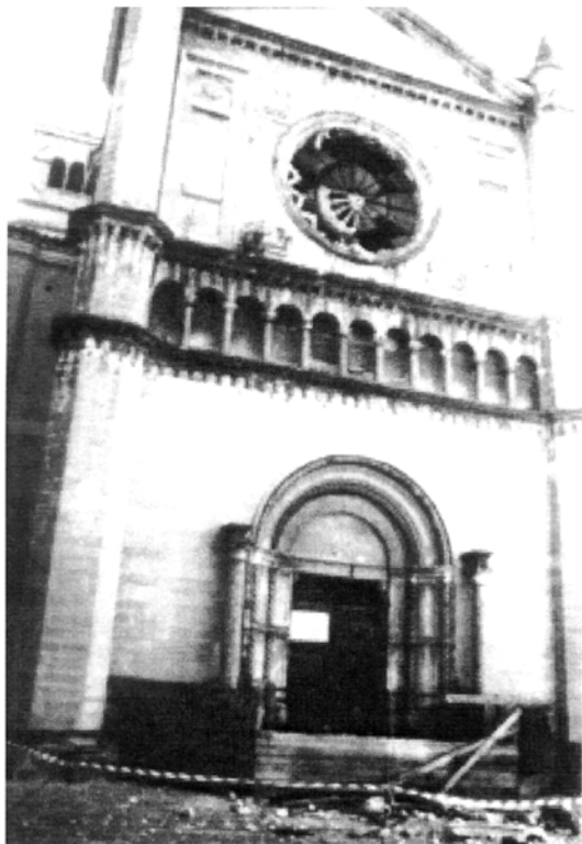
Plate 3.37: San Filippo Church, Nocera Umbra: damage to the upper part of the façade (overturning mechanism)
