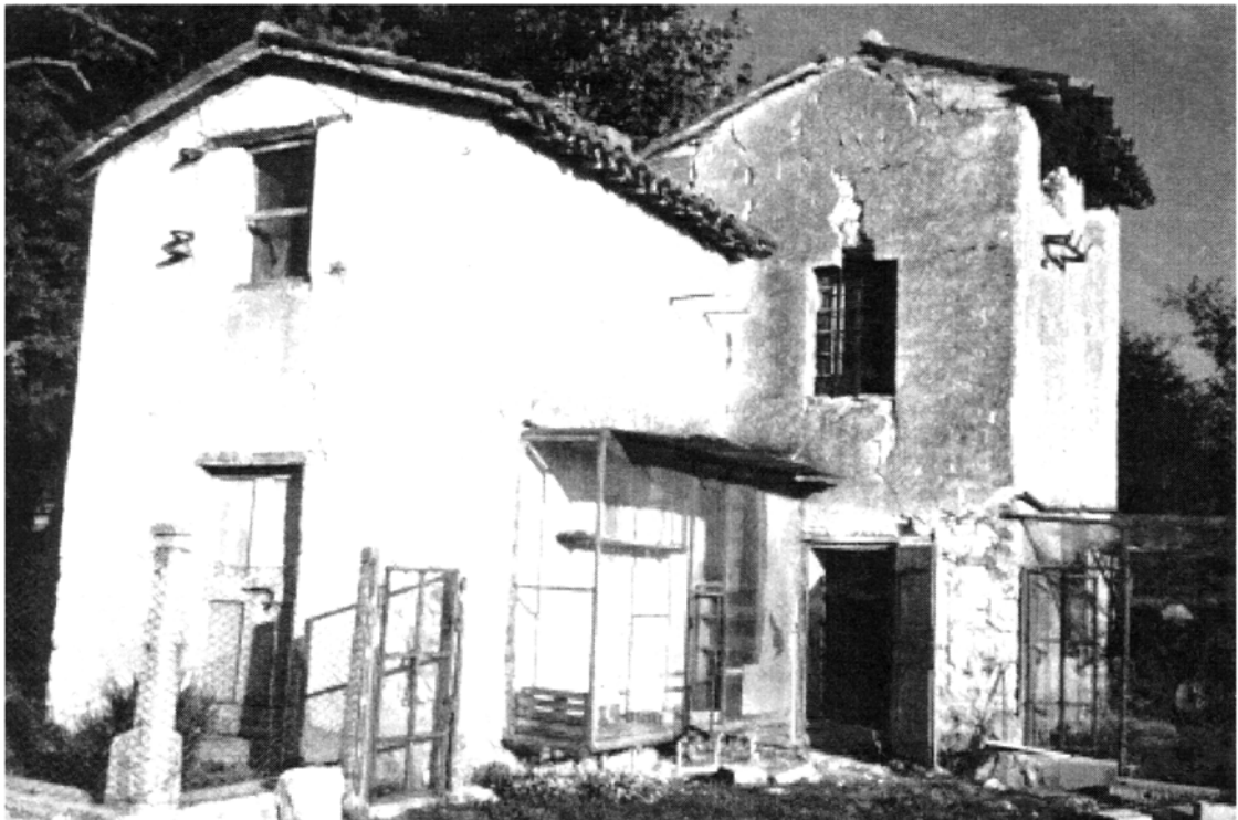
Plate 2.30: Damage to masonry buildings: Colfiorito SMI site
