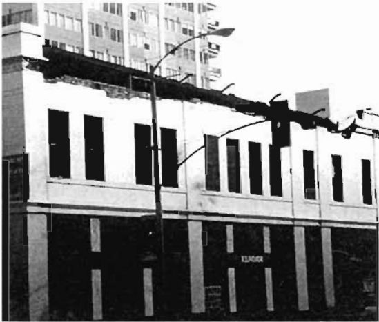
Plate 6.194: Fallen parapet with stays but no roof ties
