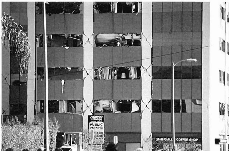
Plate 6.59: X-cracking in columns
