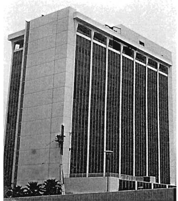
Plate 6.112: Flexural wall cracks in First Interstate Bank building
