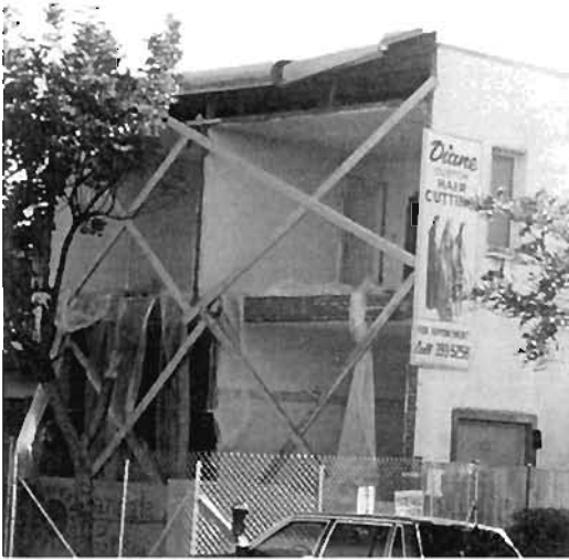
Plate 6.167: Collapsed house front
