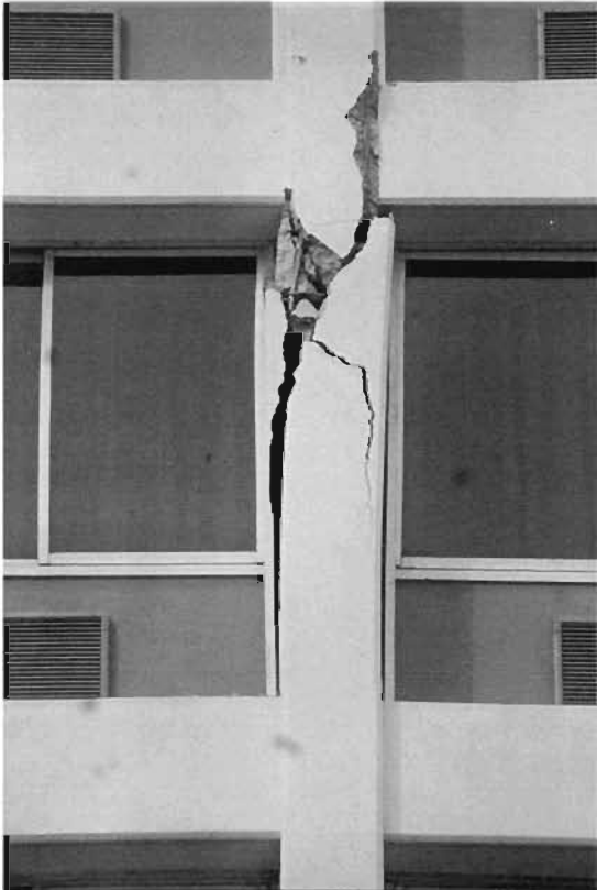
Plate 6.100: Close-up of X-cracking in columns
