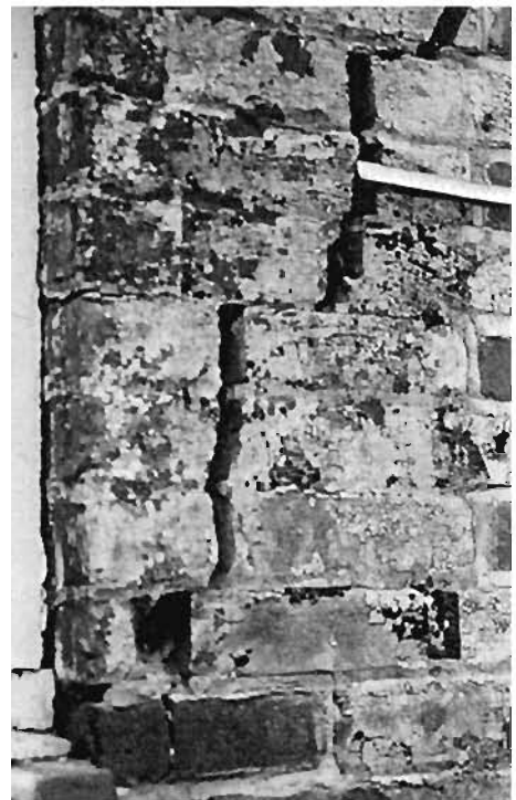
Plate 6.199: In-plane cracking of masonry by door
