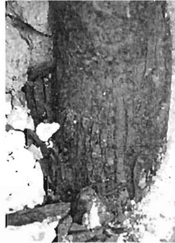
Plate 6.175: Corroded steel post
