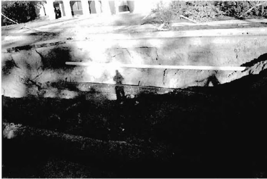
Plate 3.16: Upward bending of lifelines on Balboa Boulevard; burst gas mains caused extensive fires here
