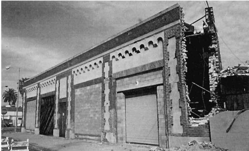
Plate 6.189: Local collapse in building retrofitted only at roof
