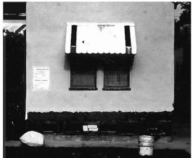
Plate 6.154: Damaged crawl space
