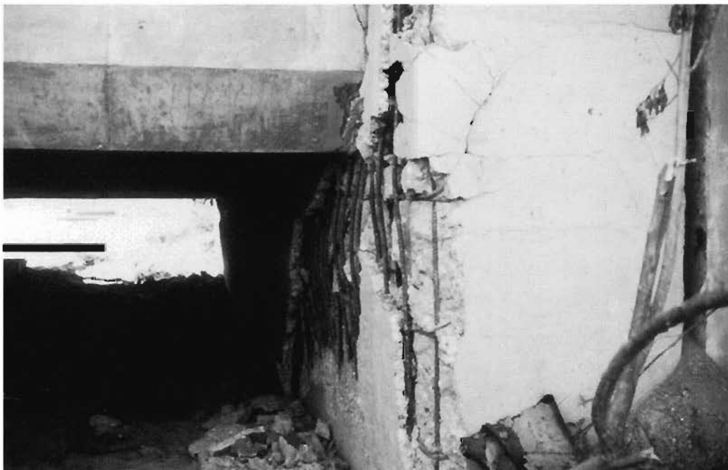
Plate 5.4: S5-E14 connector - damage to abutment wall
