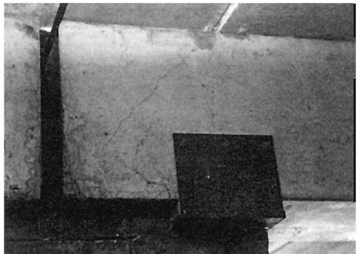
Plate 6.35: Old cracking at end of beams
