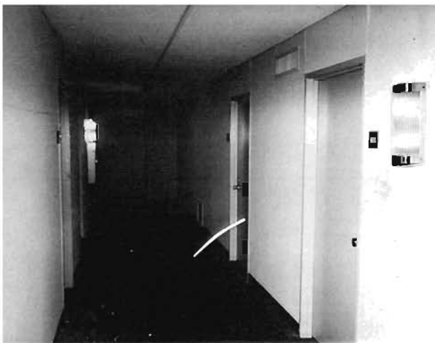
Plate 6.109: Minor damage to wall linings at 4th floor
