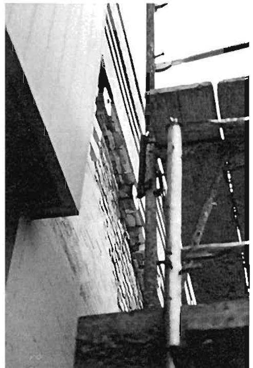
Plate 6.204: Plane of delamination and ties limiting extent of failure
