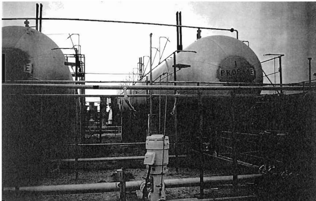
Plate 7-6 : Rotated horizontal cylindrical tank supported on concrete saddles, Van Nuys
