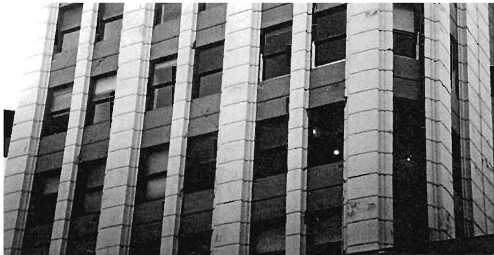
Plate 6.137: X-cracking in beams of 12 storey building in Santa Monica
