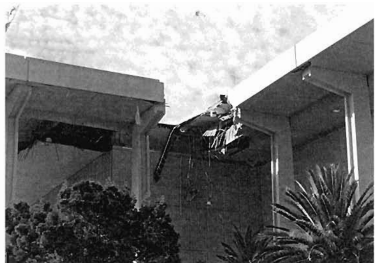
Plate 6.83: Fallen canopy in re entrant corner at rear
