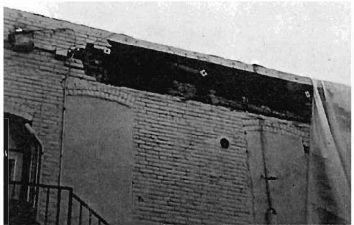
Plate 6.193: Fallen masonry in vicinity of wall ties
