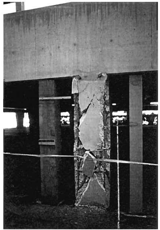
Plate 6.31: Shear cracking in columns on south side
