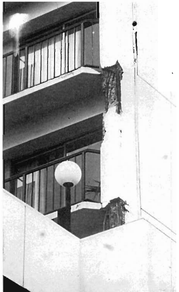
Plate 6.117: Buckled shear wall reinforcement above low level roof
