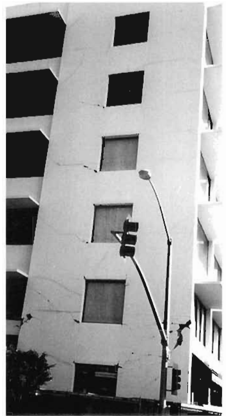
Plate 6.119: Wall cracks in coupled shear walls (NW corner)
