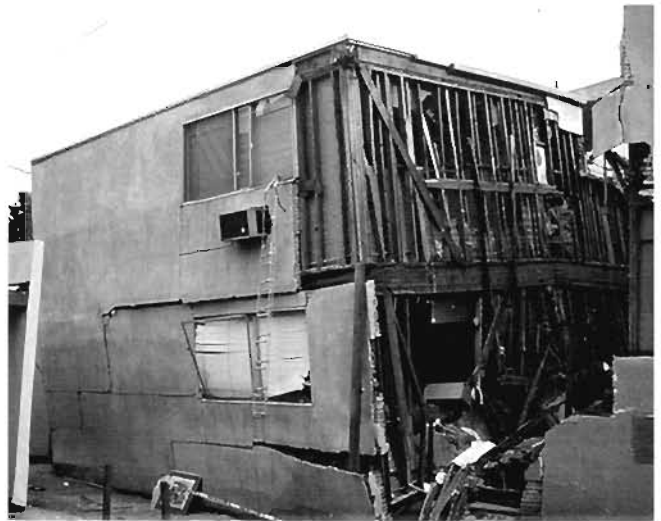
Plate 6.158: Collapsed part and part with collapsed soft storey
