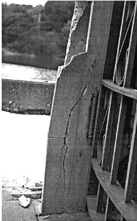
Plate 4.11: Upper Hollywood Reservoir - Damage to face of tower
