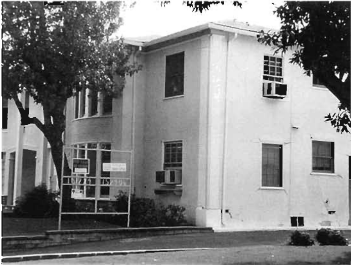
Plate 6 155: Stucco damage at crawl space in apartments
