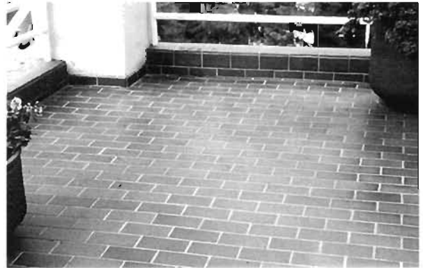
Plate 6.217: Diagonal crack in floor
