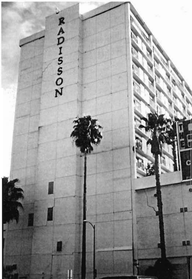
Plate 6.116: Cracked shear wall above low level roof
