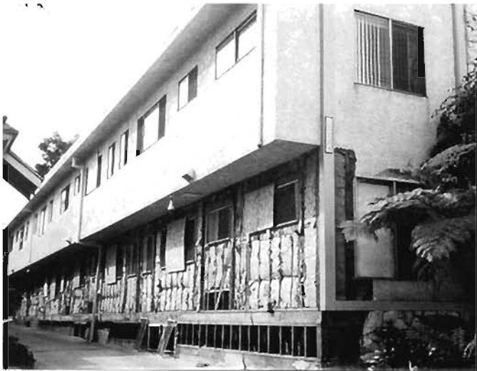
Plate 6 157: Stucco fallen from insulated timber frame apartment
