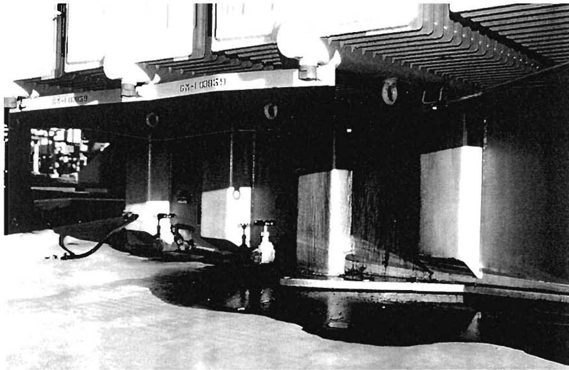
Plate 8-7 : Buckled brace and oil leakage at cooling fins of transformer, Sylmar converter station
