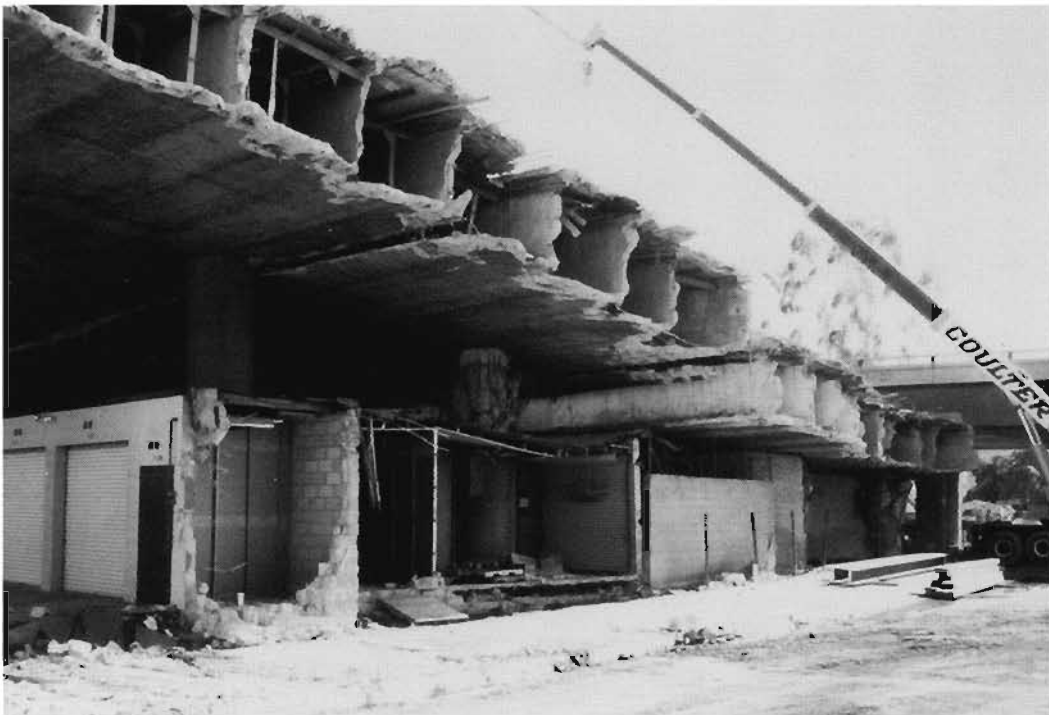
Plate 5.11: Santa Monica Freeway at La Cienega and Venice - influence of column height
