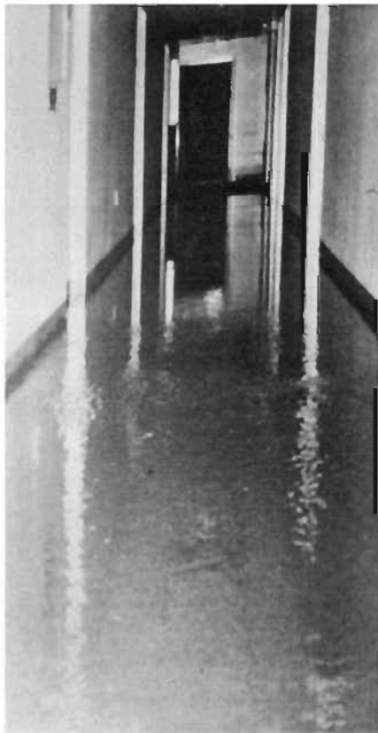
Plate 6.72: Flooded 6th floor corridor
