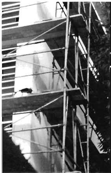
Plate 6.121: Comparable damage in SW corner
