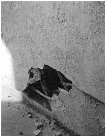
Plate 6.165: Damage exposing wall interior
