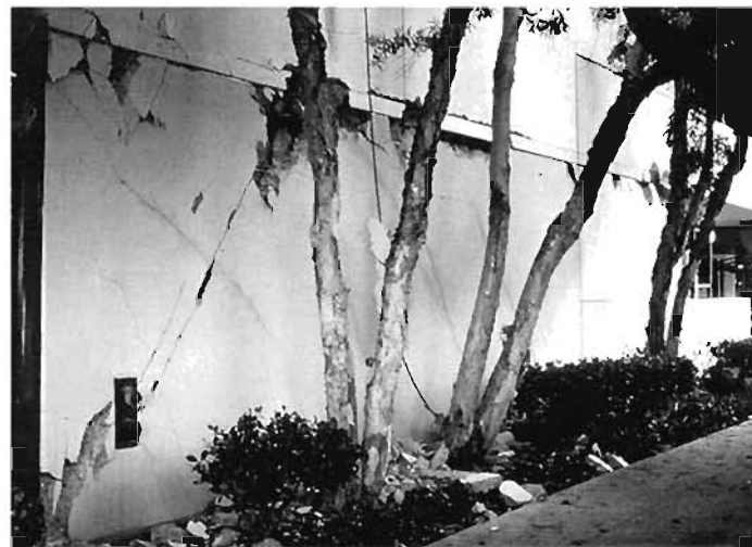
Plate 6.40: X cracking in shear wall panels at St John's Hospital car park
