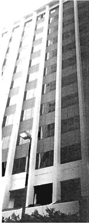
Plate 6.135: Horizontal cracking around window panels in first floor beam in office building,
