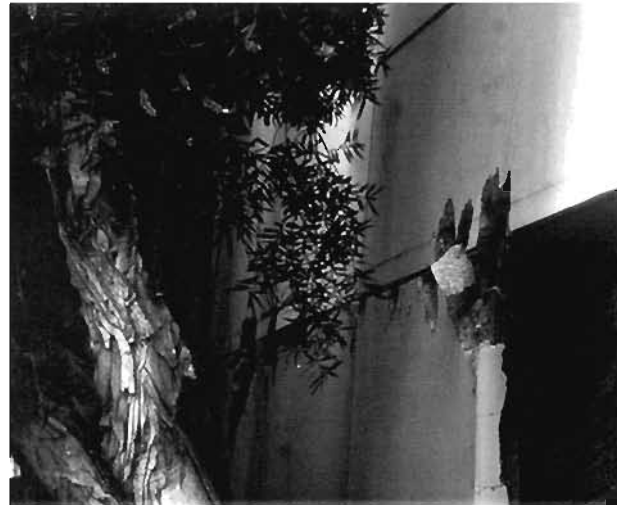
Plate 6.39: St. John's Hospital car park : cracked concrete at corners of opening in walls.
