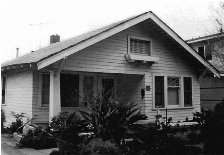
Plate 6.153: Collapsed crawl space
