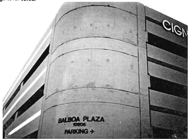
Plate 6.41: Undamaged curved wall of Cigna Garage
