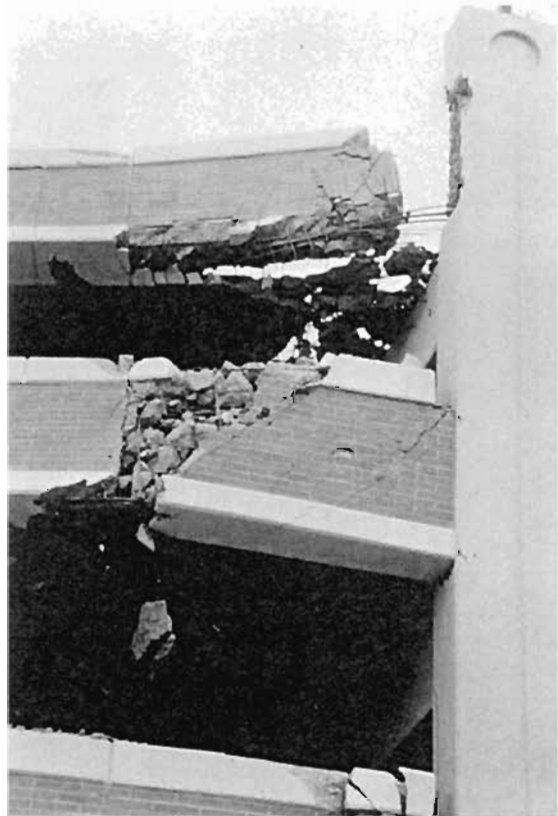
Plate 6.17: In-plane flexural failure of perimeter frame
