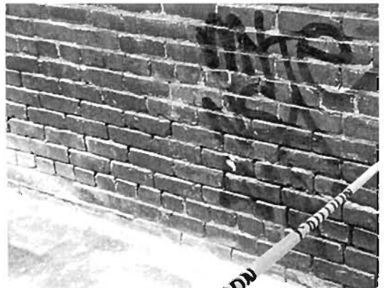
Plate 6.172: Cracking lower down
