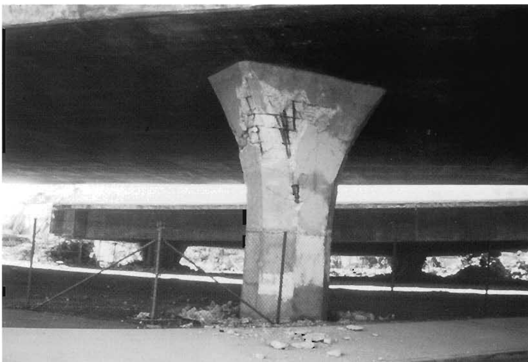
Plate 5.9: H118 at Mission and Gothic - column failures in Bent 2L
