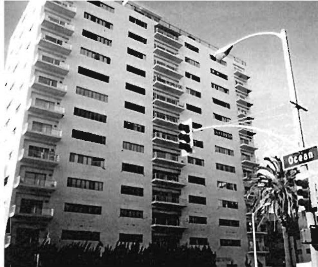
Plate 6.136: Damage to first floor window panels in apartments in Santa Monica
