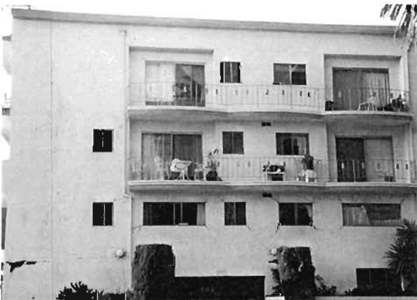
Plate 6.223: Damage in end shear wall in apartments in Santa Monica
