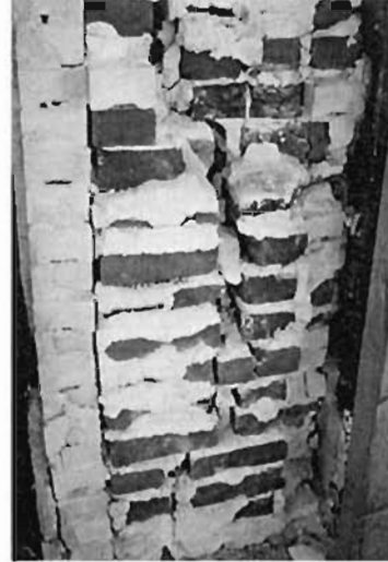
Plate 6.174: Disintegrating columns with steel posts
