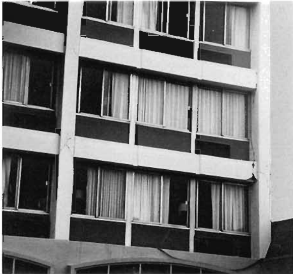
Plate 6.98: Close-up of cracking damage at second floor on North side
