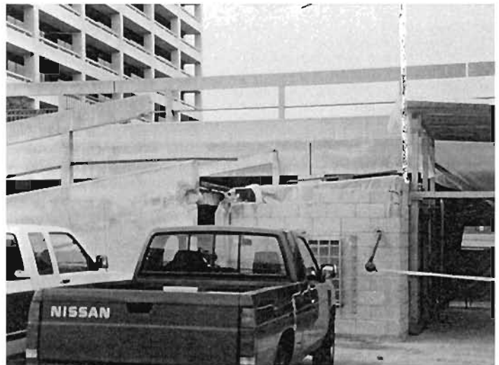
Plate 6.32: Collapsed car park ramp
