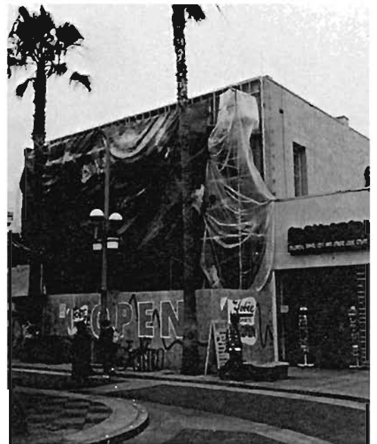
Plate 6.168: Collapsed shop front
