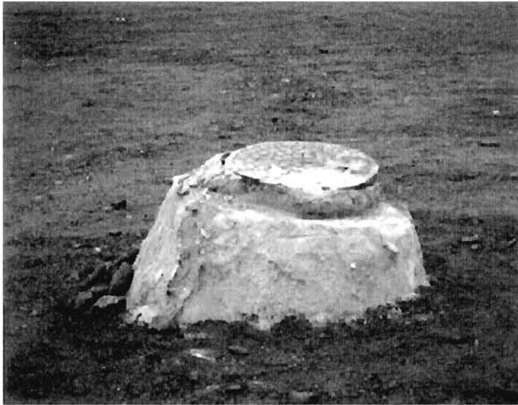
Plate 3.10: Subsidence between the quay walls; plate shows original level flush with the manhole cover and the subsidised ground level
