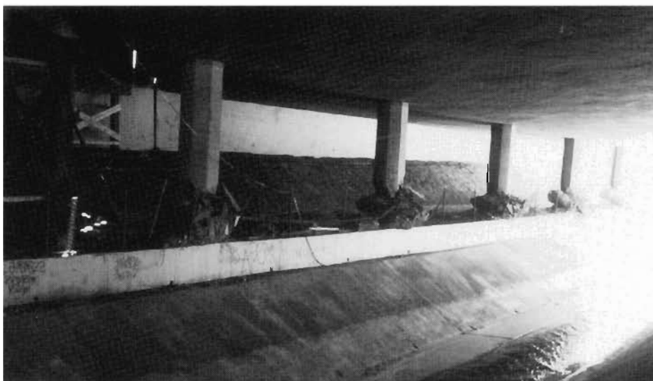
Plate 5.7: Column failures at Bull Creek Canyon bridge
