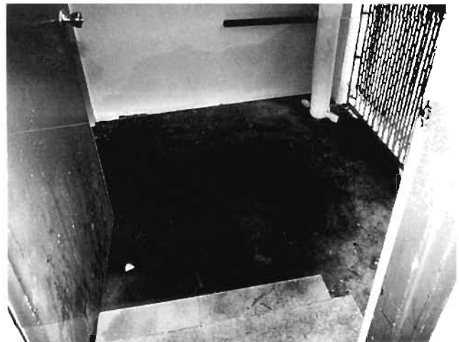
Plate 6.110: Carpetting and hydraulic fluid in stairwells by lift
