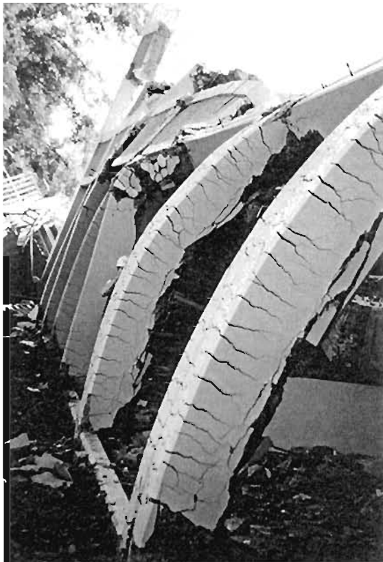
Plate 6.21: Closely spaced flexural cracks almost reaching compression face
