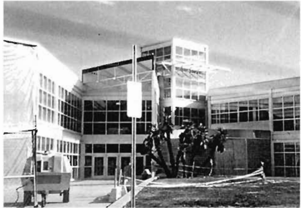
Plate 6.91: Steel framed book store with fallen tilt-up panels
