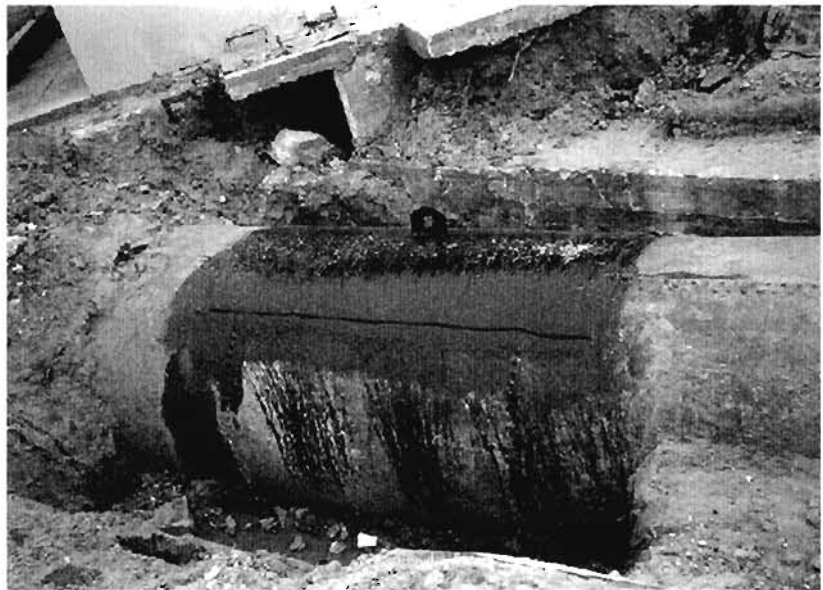
Plate 3.14: Breakage of main outlet pipe of Los Angeles Dam; plate shows recent repairs to the pipe following the earthquake
