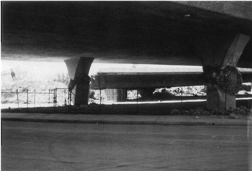
Plate 5.8: H118 at Mission and Gothic - column failures in Bent 3L
