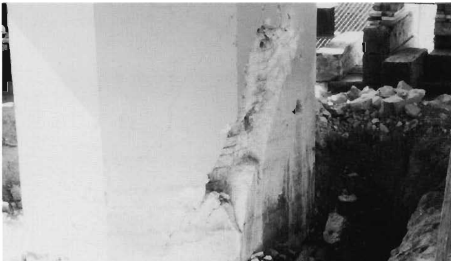
Plate 5.6: I405/H118 interchange - shear damage at base of column
