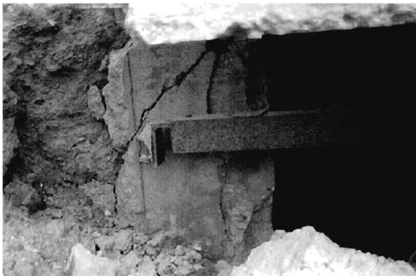
Plate 3.15: Ground movement causing failure of outlet pipe is confirmed by failure of foundation block of nearby pump house
