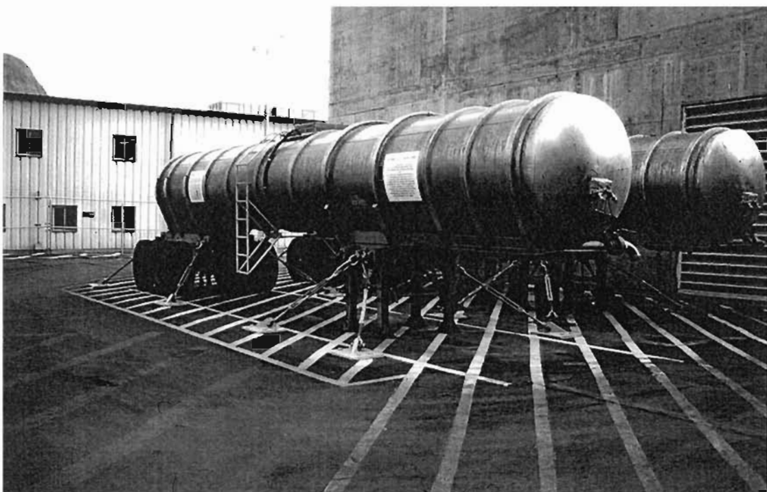
Plate 8-10 : Additional water supply designated for seismic emergency, San Onofre NPP
