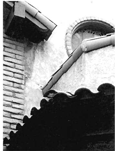
Plate 6.221: Cracking in irregularity above porch
