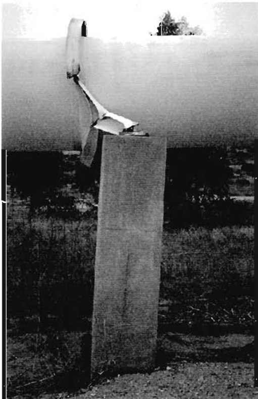
Plate 3.6: Sheared connection between the pipe and column; plate also shows leaning of the column and the gap between the column and foundation soil
