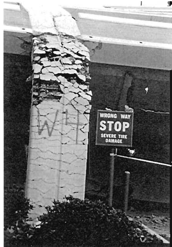
Plate 6.22: Spalling outside the well confined column cage
