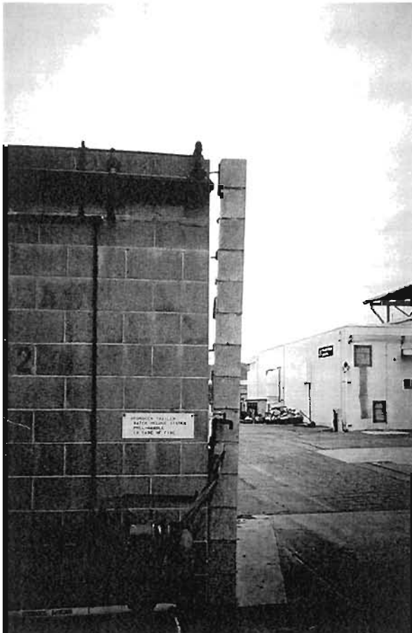
Plate 7-10 : Damage to blast wall due to inadequate continuity, Van Nuys
