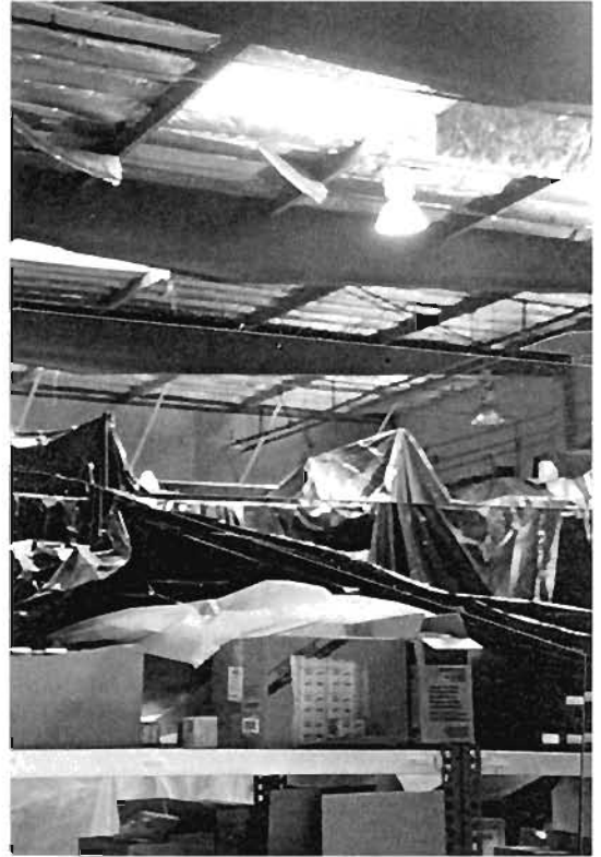
Plate 6.75: Interior and damage to plywood roof
