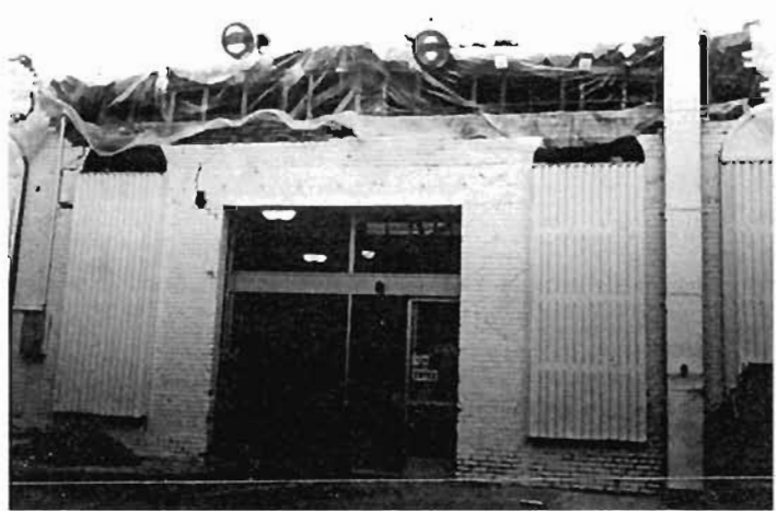
Plate 6.195: Failure of masonry in vicinity of wall ties
