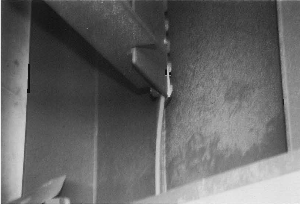
Plate 5.12: Peco Lyons Bridge - buckling of gusset plate
