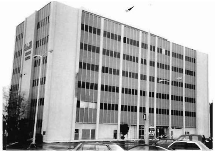
Plate 6.65: Rear view showing spalling at end walls
