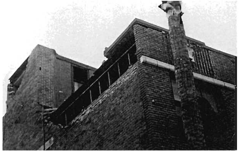
Plate 6.169: Top storey side wall collapse
