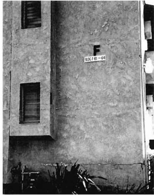
Plate 6.163: Low level horizontal crack despite absence of crawl
