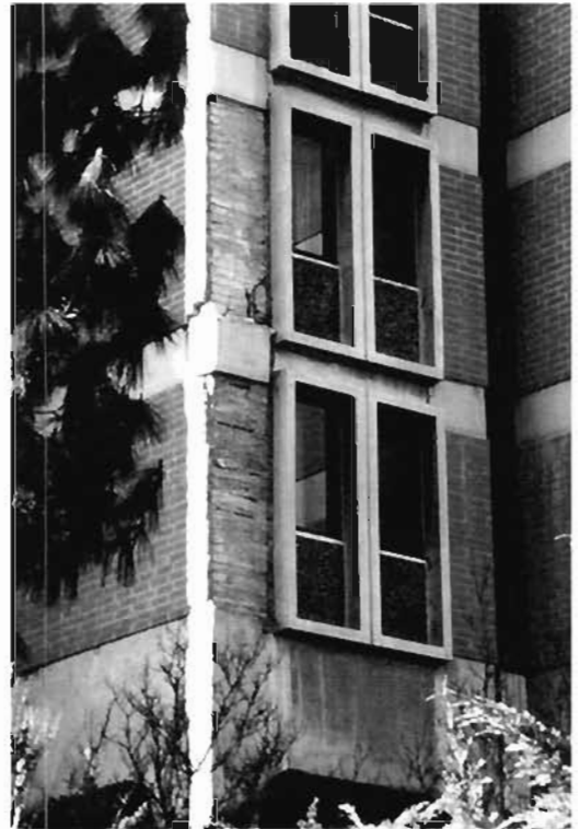
Plate 6.183: Fallen masonry at end of wall
