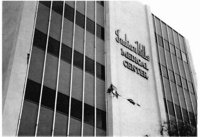
Plate 6.66: Side wall damage at fourth floor
