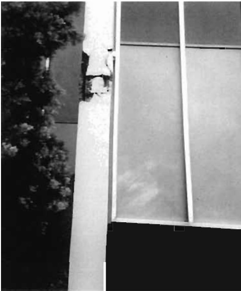
Plate 6.69: Side wall damage at front on first floor
