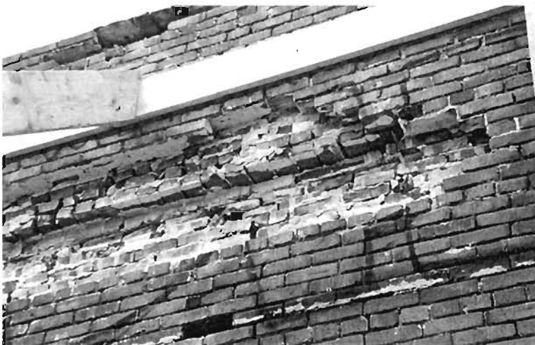
Plate 6.171: Delaminated outer skin
