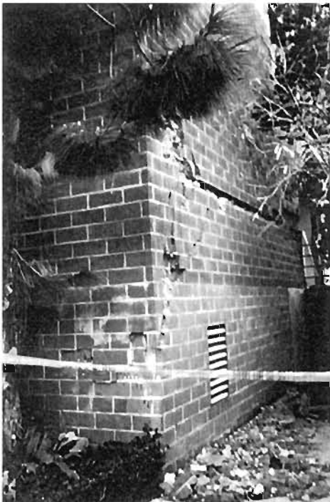
Plate 6.185: Low level disintegration of reinforced masonry
