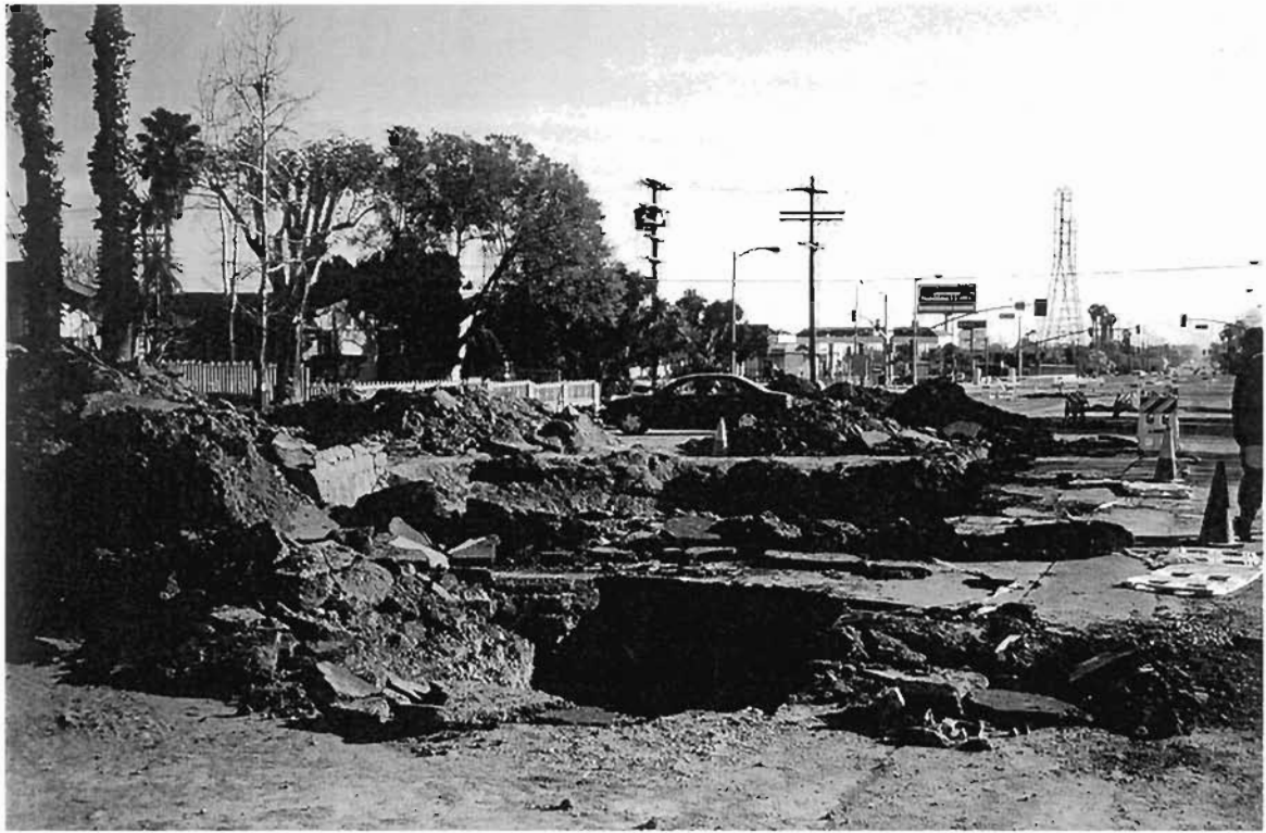
Plate 8-13 : Typical location of gas and water pipe breakage, Granada Hills
