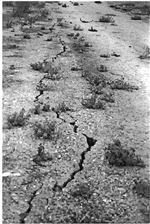
Plate 4.6: Lower San Fernando Dam Longitudinal crack in crest
