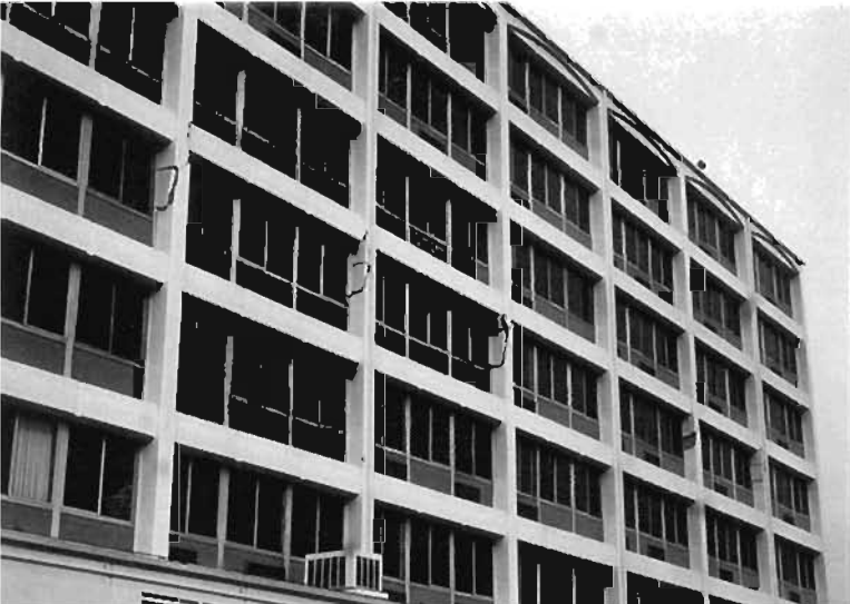
Plate 6.99: Damaged fourth floor columns, South side
