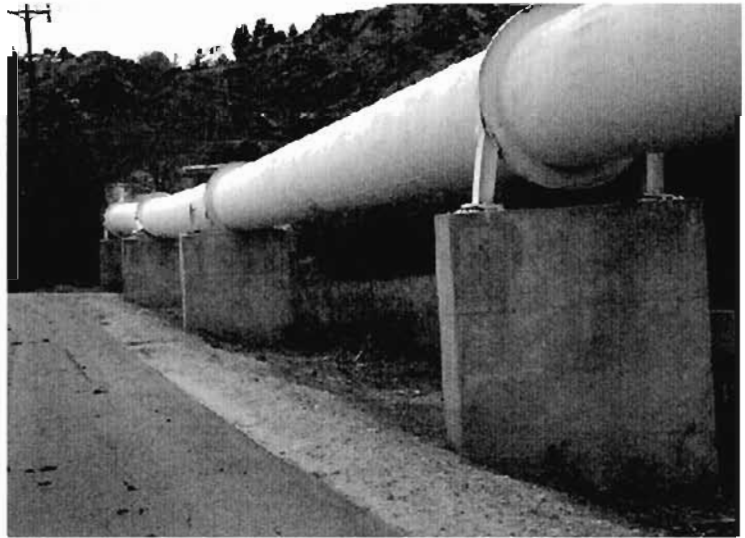
Plate 3.5: Pipeline on downstream side of Upper San Fernando Dam; the ground motion at this site was along the pipeline
