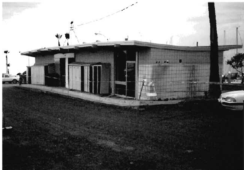
Plate 3.12: Structural damage due to subsidence following liquefaction; plate shows left hand side of building higher than right
