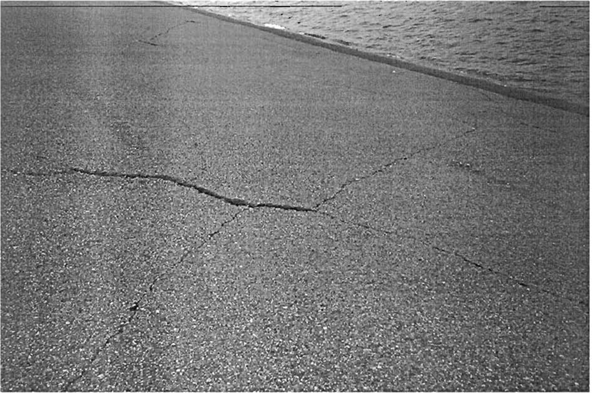
Plate 4.2: Los Angeles Dam - Diagonal Cracks in Asphalt Lining on Upstream Face
