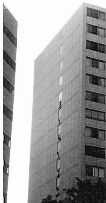
Plate 6.134: X-cracking in coupling beams on South face
