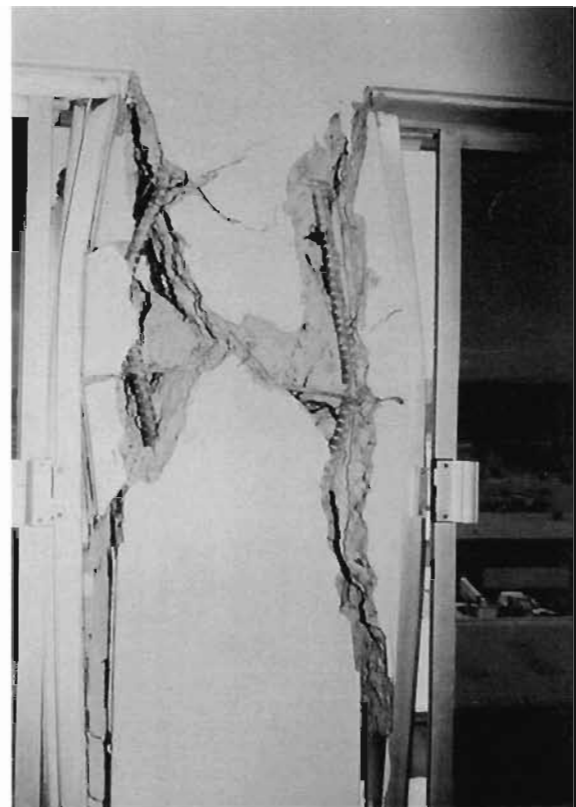
Plate 6.104: Internal view of X-cracking where tie failed
