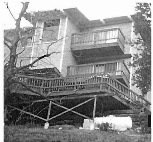
Plate 6.226: Undamaged building on crest of hill
