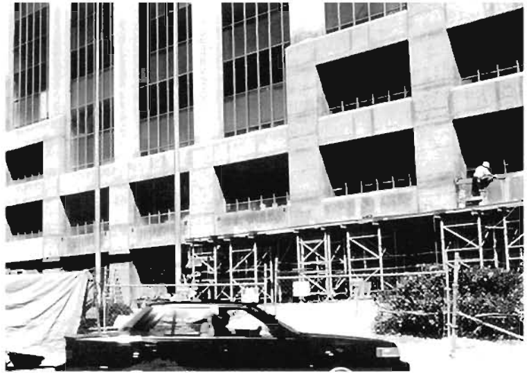
Plate 6.6: Extent of scaffold provides evidence of damage sustained
