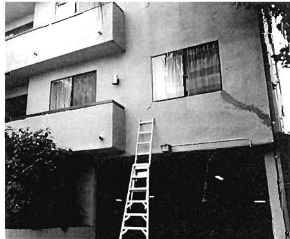
Plate 6.224: Crack above car park entrance at end of building
