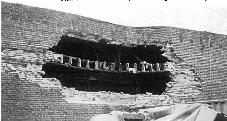
Plate 6.190: Wall collapse at unretrofitted intermediate floor
