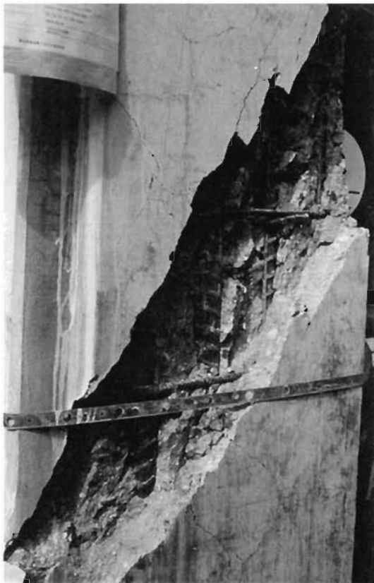
Plate 6.28: Shear cracking of column
