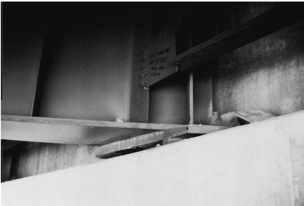
Plate 5.13: Peco Lyons Bridge - tension failure of cross-bracing
