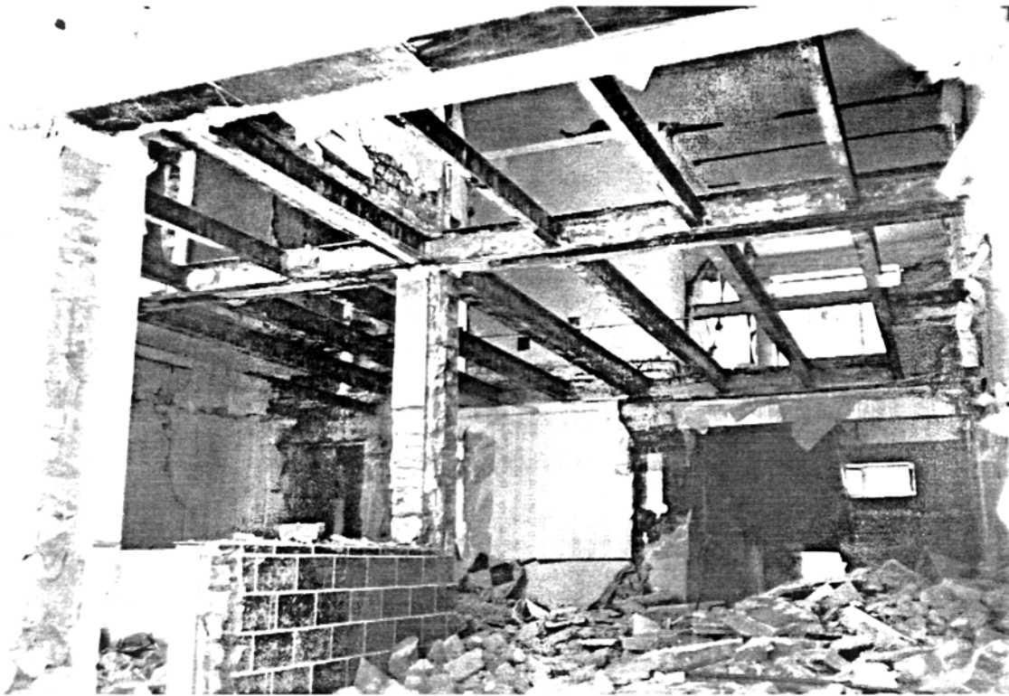
Picture 3.22 Two-storey Government Building, Rudbar Collapse of first floor jack arches without dislocation of I-beams
