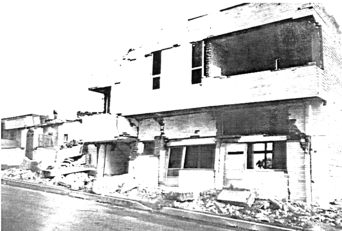
Picture 3.4 White Stone Clad House, Manjil Window frame supporting the spandrel wall and the roof after failure of load-bearing steel frame
