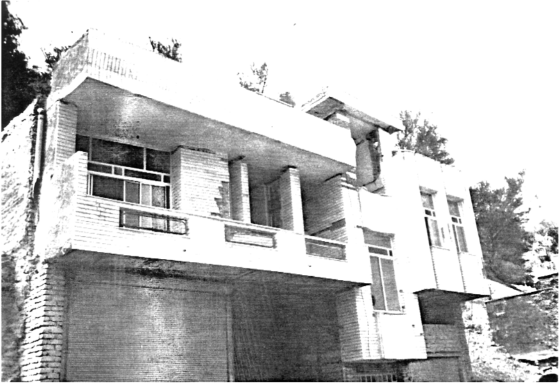
Picture 4.11 Two-storey Stone Clad House, Rudbar This relatively flexible steel frame house, founded on hard ground survived the quake with little damage
