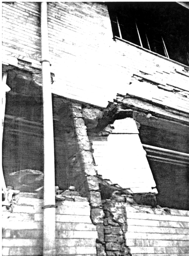
Picture 3.7 Vali-asr Hospital, Rudbar Multiple fixed-end bending failures in columns of the main building
