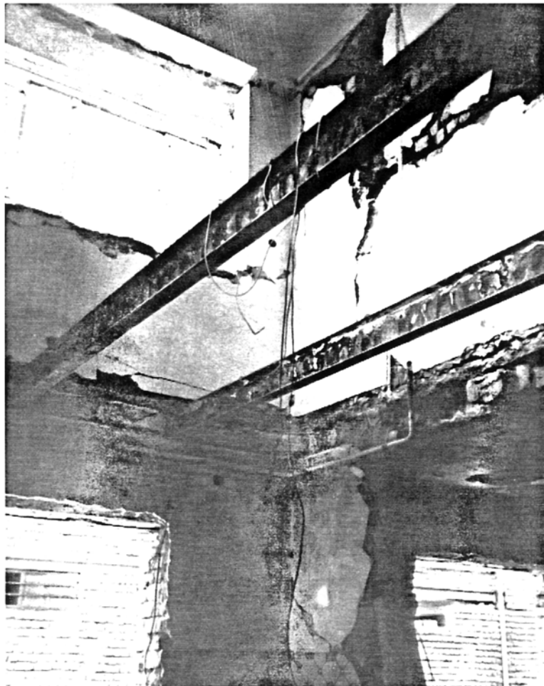
Picture 3.20 Three-storey Building, Manjil First floor jack arches collapsed despite no apparent separation of the supporting I-beams
