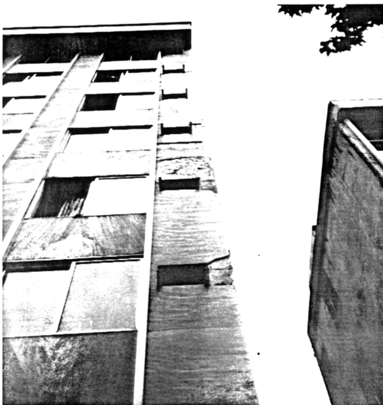
Picture 4.38 Eight-storey Grey Stone Clad Building, Rasht Collapse of sections of stone cladding the only failure in this building
