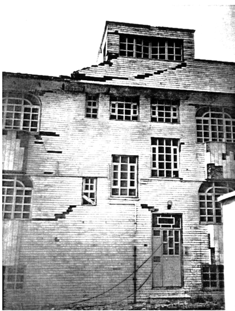
Picture 3.3 3-4 storey House, Manjil Despite many failures due to its complex architectural form the building maintained its integrity
