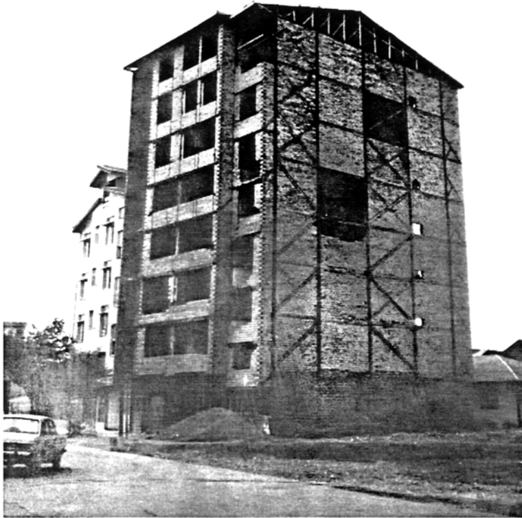
Picture 4.19 Unfinished Steel Frame Building, Rasht Lateral-torsional coupling amplification in response of the building due to its eccentric stiffness
