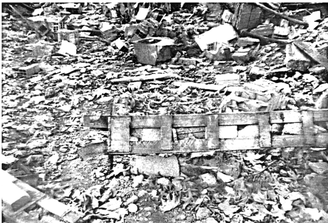
Picture 4.24 Six-storey Steel Frame Building, Rasht Weak steel column consists of two undersize I-beams
