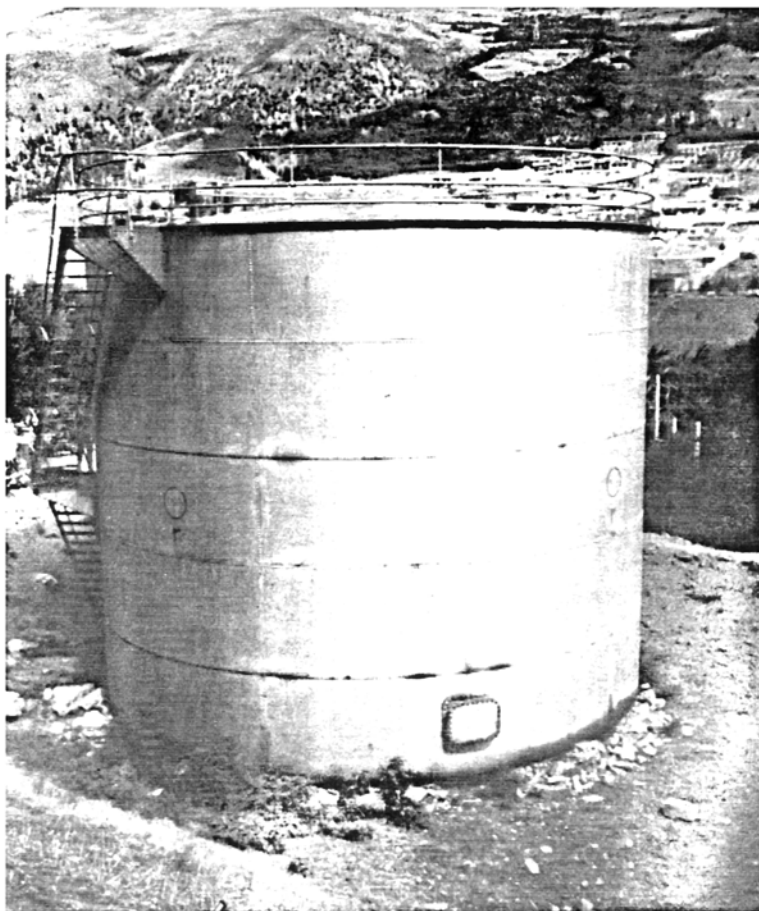
Picture 5.36 Petrol tank No. 3, Rudbar Steel tank survived the quake but the brick footing did not
