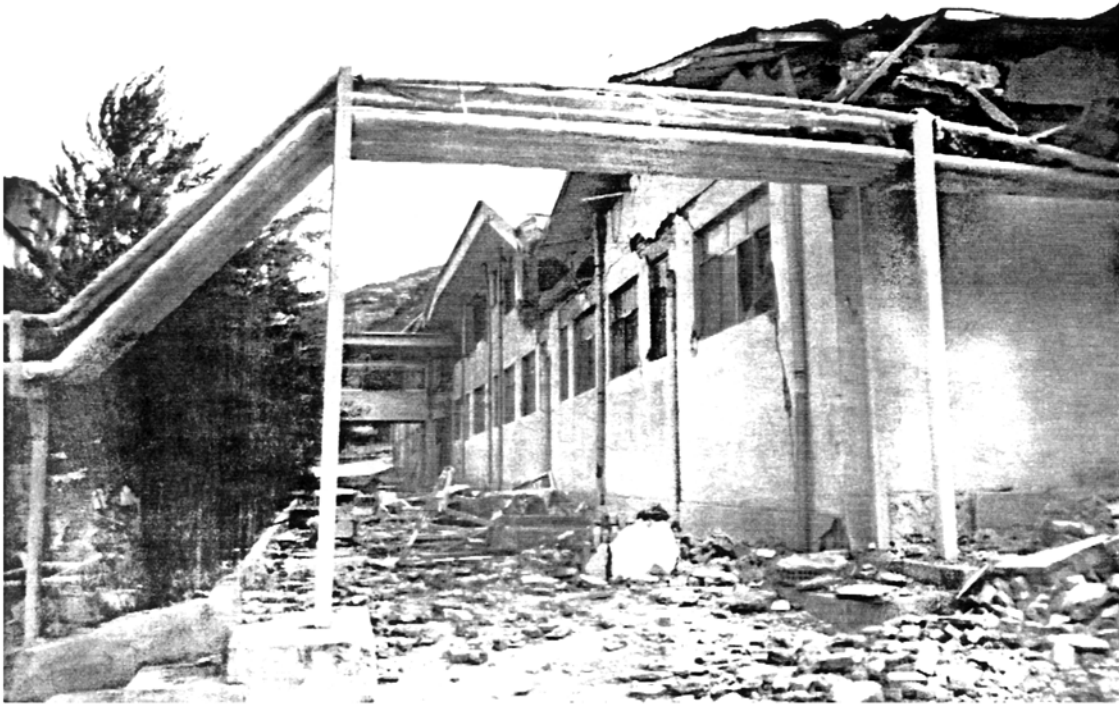
Picture 3.9 Vali-asr Hospital, Rudbar Damage to the middle one-storey building
