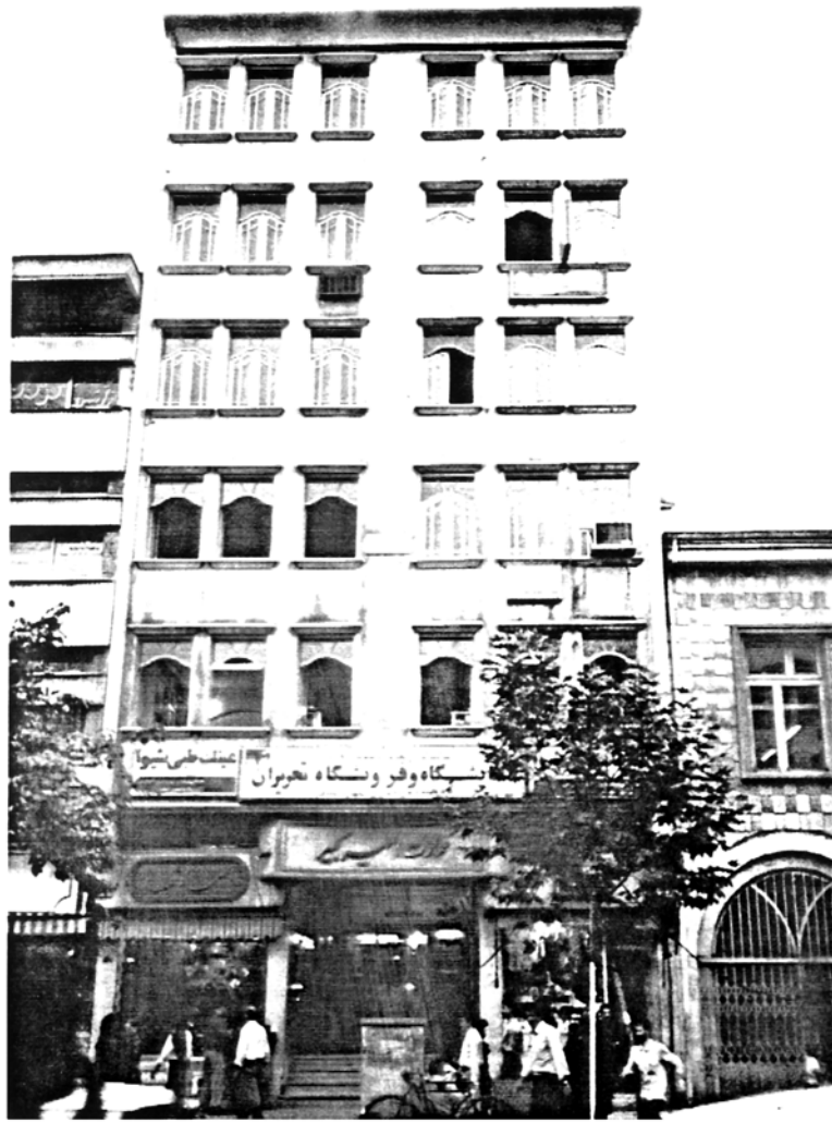
Picture 4.21 Six-storey Shop Store, Rasht Shear failure in the central infill wall
