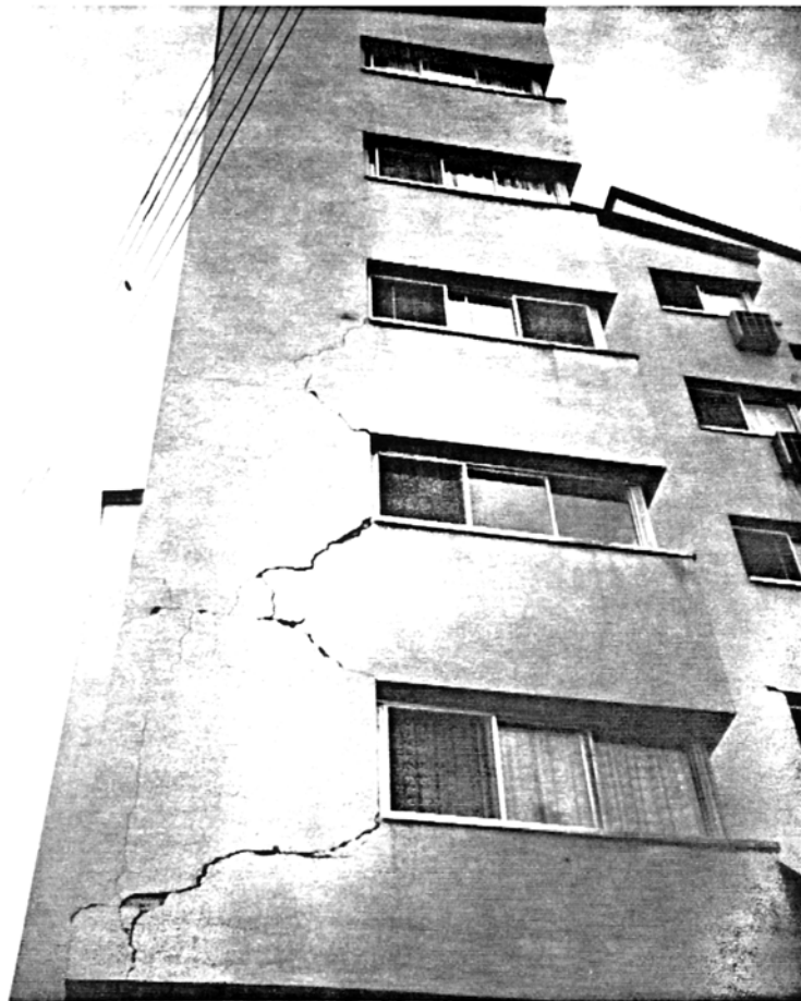
Picture 4.34 Nine-storey Apartment Block, Rasht Shear cracks in the infill walls
