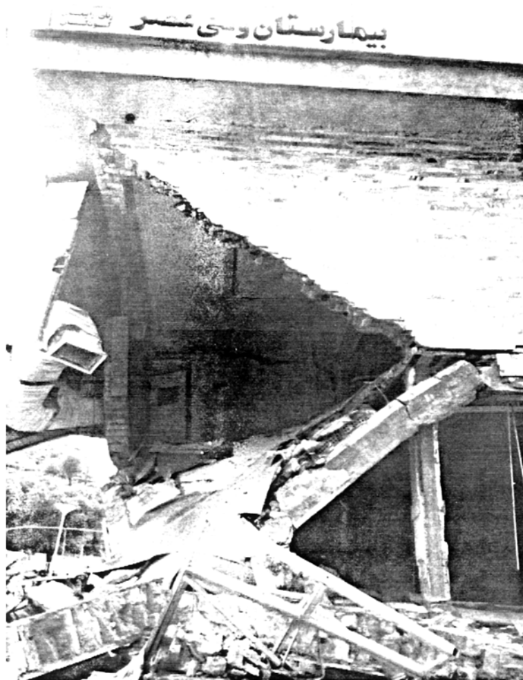
Picture 3.6 Vali-asr Hospital, Rudbar excellent behaviour of roof concrete ring-beam after collapse of main load-bearing elements at this corner
