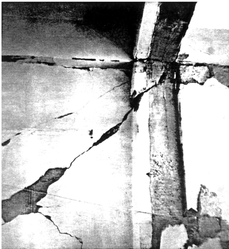
Picture 4.5 Telecom Centre, Manjil Diagonal shear failure in the concrete block masonry wall extending to the reinforced concrete column
