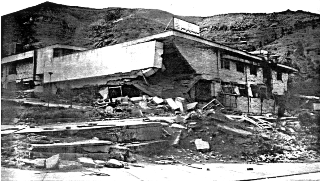
Picture 3.5 Vali-asr Hospital, Rudbar Damage to the entrance of the main building
