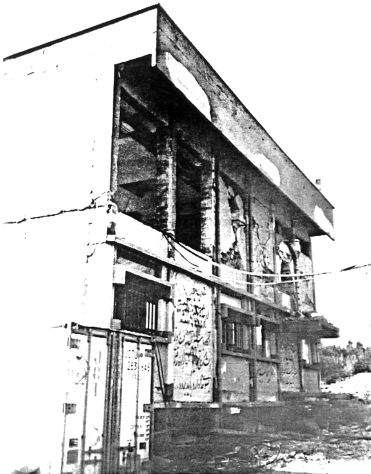
Picture 4.6 Telecom Centre, Manjil View of east face of the building indicating lesser response at the south-east corner
