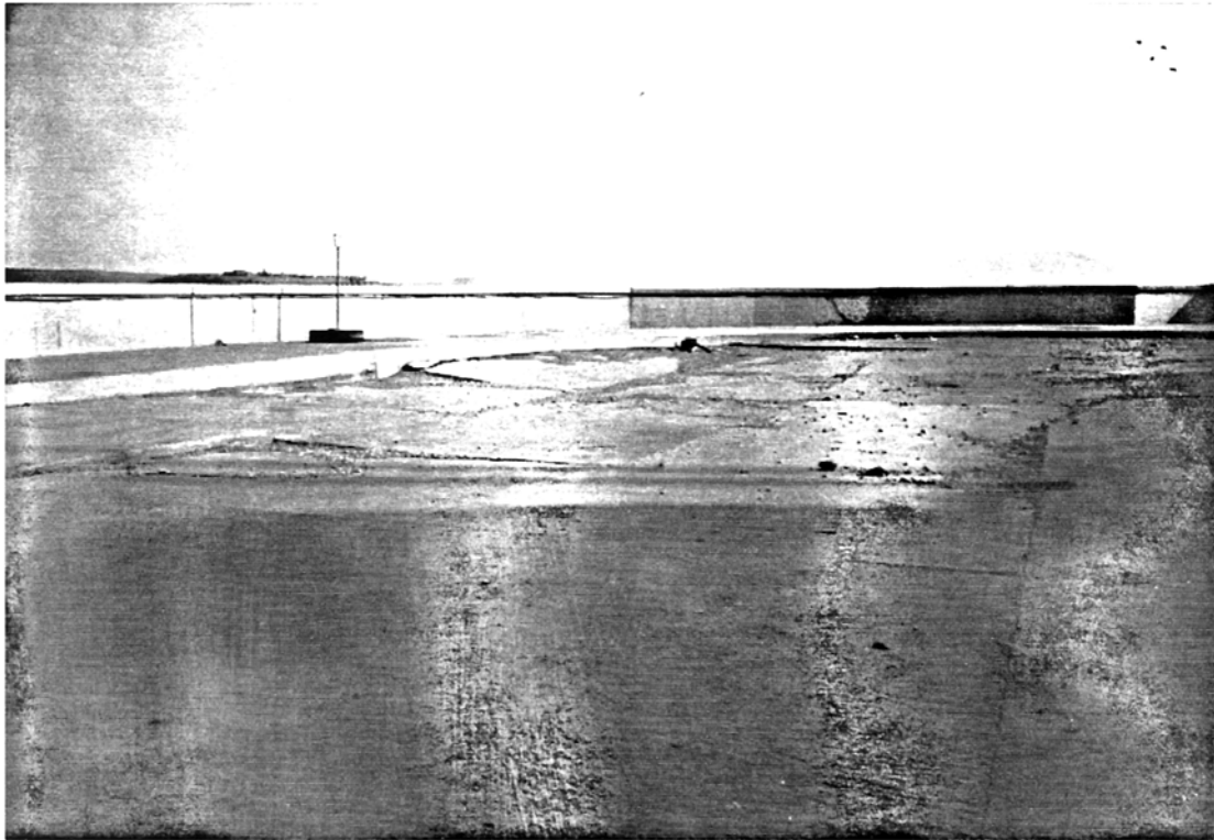
Picture 5.9 Sefid-rud Dam, Manjil Subsidence of the fill at the west end adjoining the concrete section of the dam
