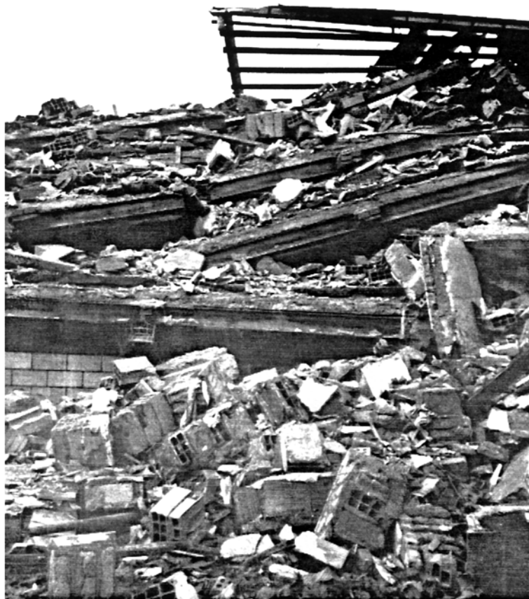
Picture 4.23 Six-storey Steel Frame Building, Rasht Concrete beam-block floor slabs maintaining their integrity after collapse
