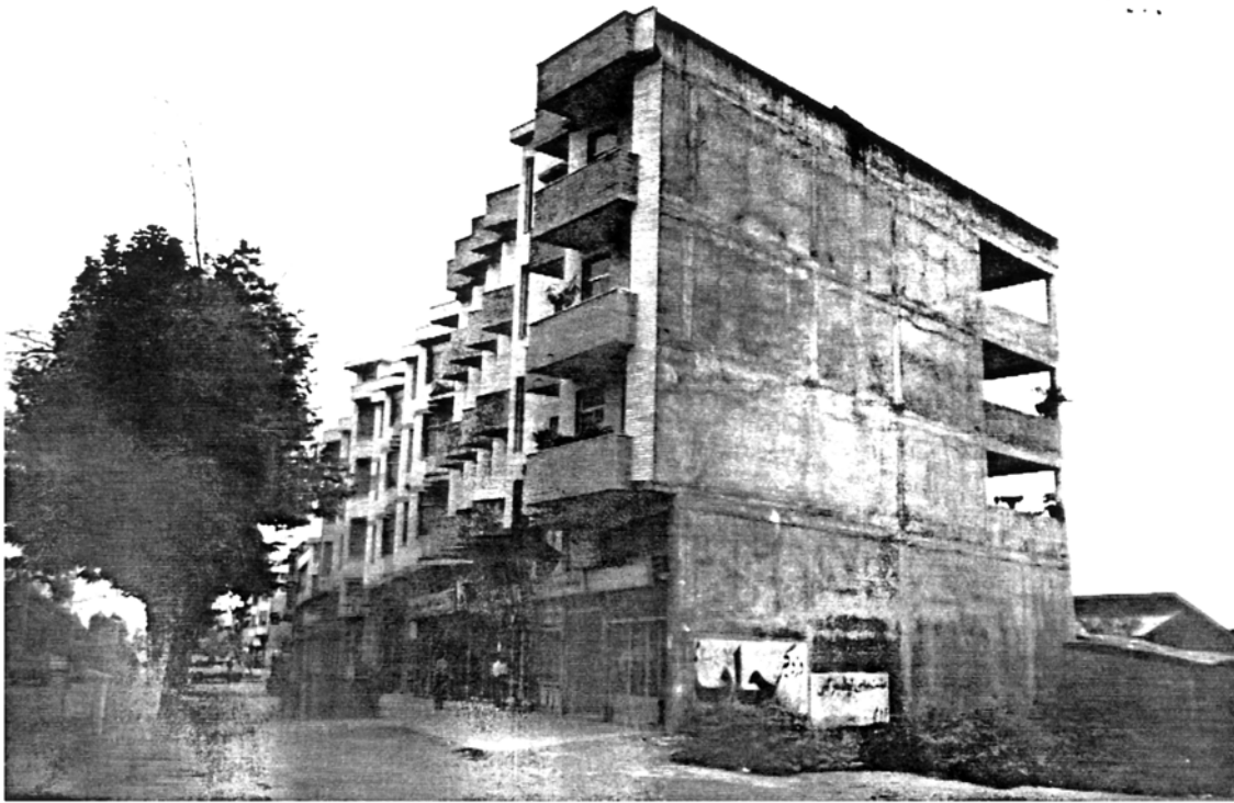
Picture 4.31 4-6 Storey Concrete and Steel Frame Buildings, Rasht The better behaved concrete frame building also supported the weaker neighbouring steel frame buildings
