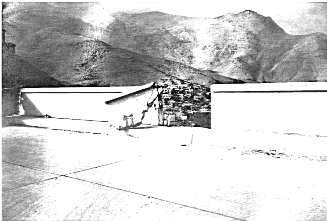
Picture 5.8 Sefid-rud Dam, Manjil Flexural failure in the long, unsupported reinforced concrete parapet wall
