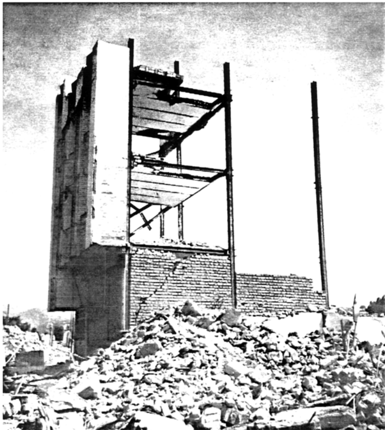
Picture 4.17 Three-four Storey Steel Frame House, Manjil Amplification of response at the back of the building due to lateral-torsional coupling caused by both mass and stiffness eccentricities in the building
