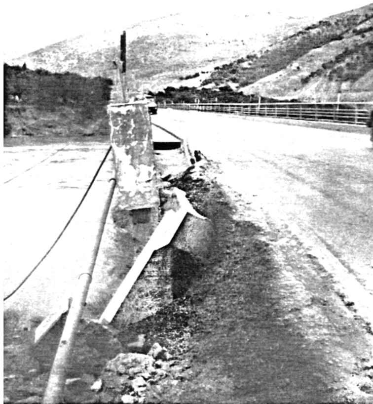
Picture 5.18 Concrete Bridge, Rudbar Failure of the south-west retaining wall
