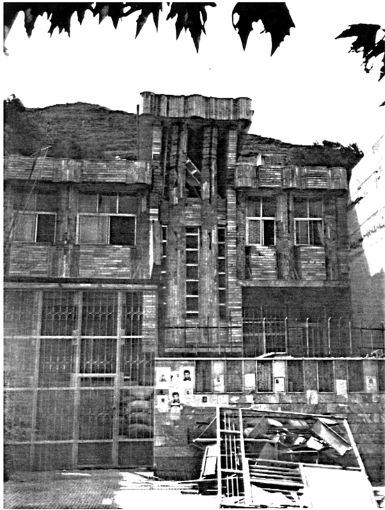
Picture 3.23 Damage to Two-three Storey Steel Frame Residence, Rudbar
