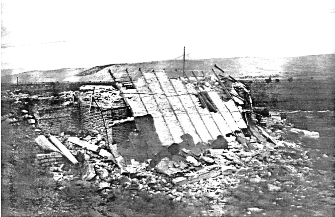
Picture 3.16 Two-storey Jack-arch Brick Building, Near Rudbar Collapse of the roof due to inadequate vertical support but steel bars keeping the I-beams and jack-arches together
