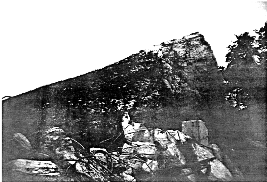
Picture 5.28 Concrete Water Tower No. 1, Rasht Explosive compressive failure of concrete at the lower section of the shaft during collapse
