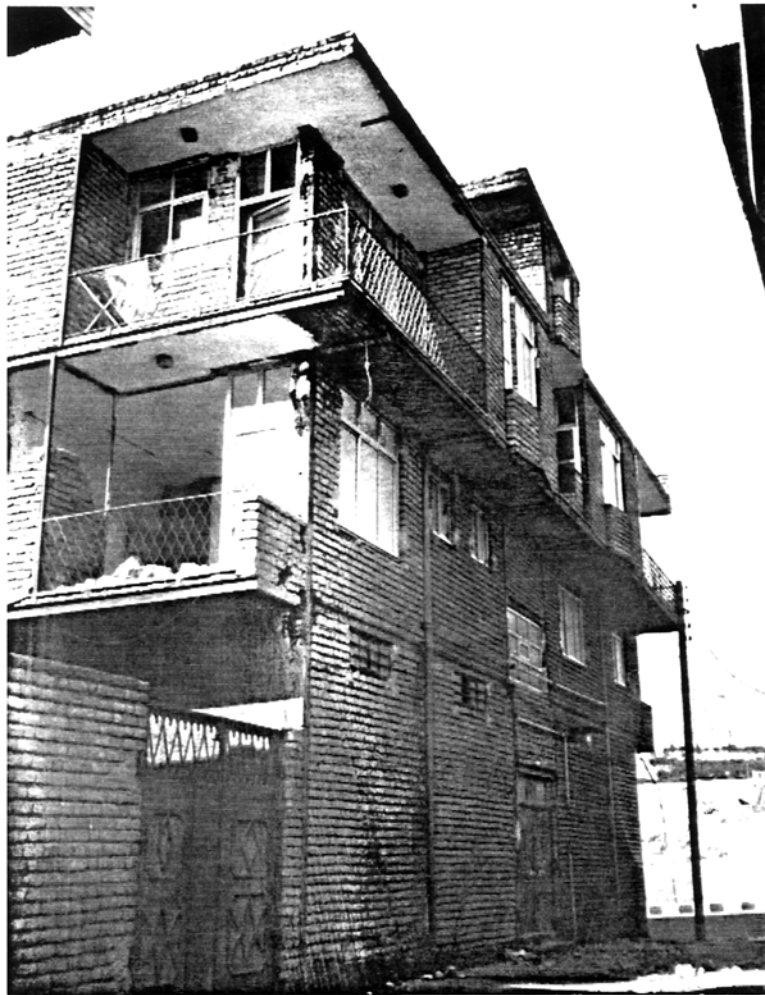
Picture 4.7 3-4 Storey Steel Framed Building, Manjil The good behaviour of this relatively well constructed building was probably due to its flexibility
