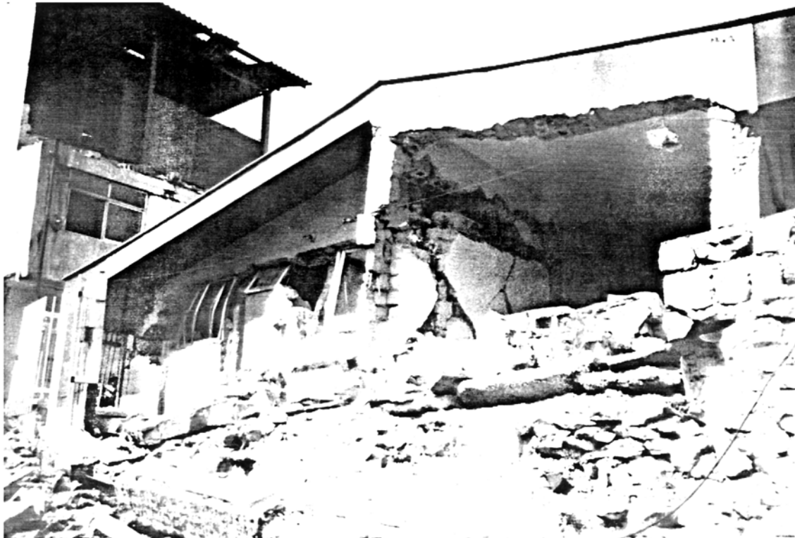
Picture 4.12 One-storey Reinforced Concrete Frame House, Rudbar This relatively stiff house, founded on built ground suffered heavy damage due to high dynamic amplification
