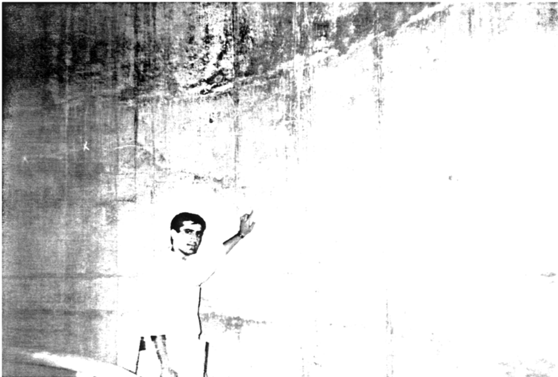
Picture 5.34 Concrete Water Tower No. 3, Rasht Horizontal bending cracks joined by short vertical cracks indicate the path of the weakest section of the shaft in taking bending stresses
