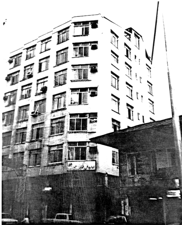
Picture 4.29 Telecom Building, Rasht A well behaved steel frame building with minor damages
