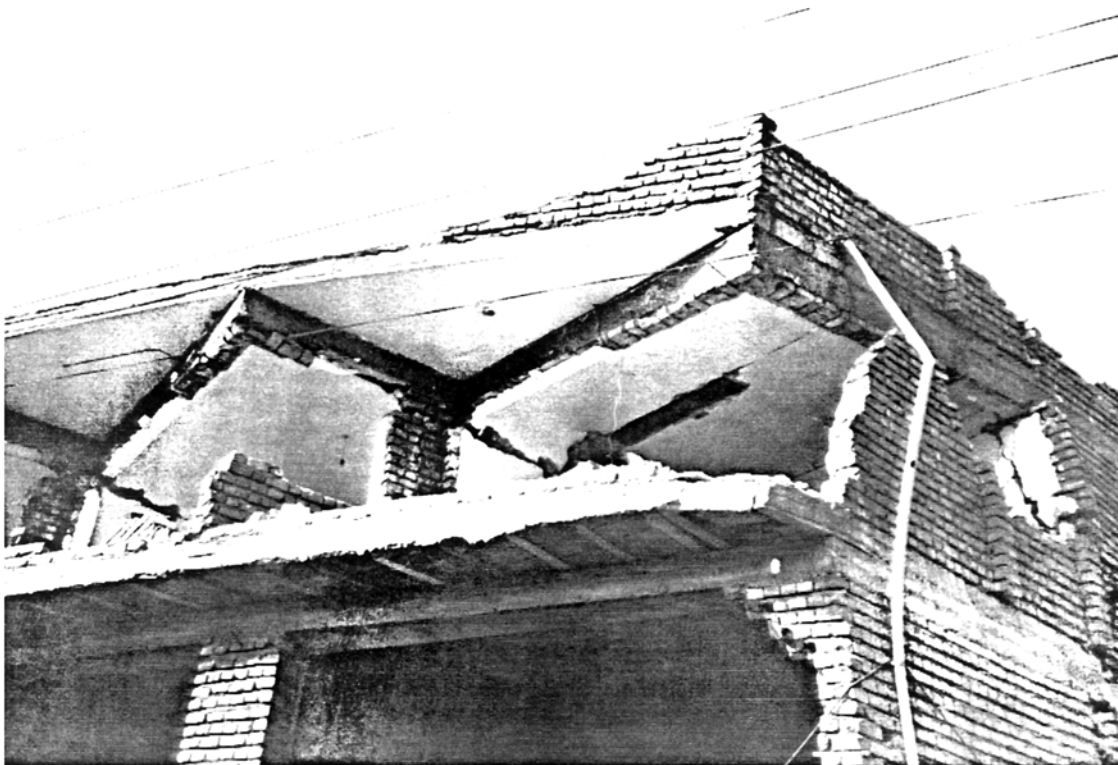
Picture 3.12 Two-storey Brick Building, Manjil Despite loss of load bearing west wall elements the concrete ring beam has kept the roof in place
