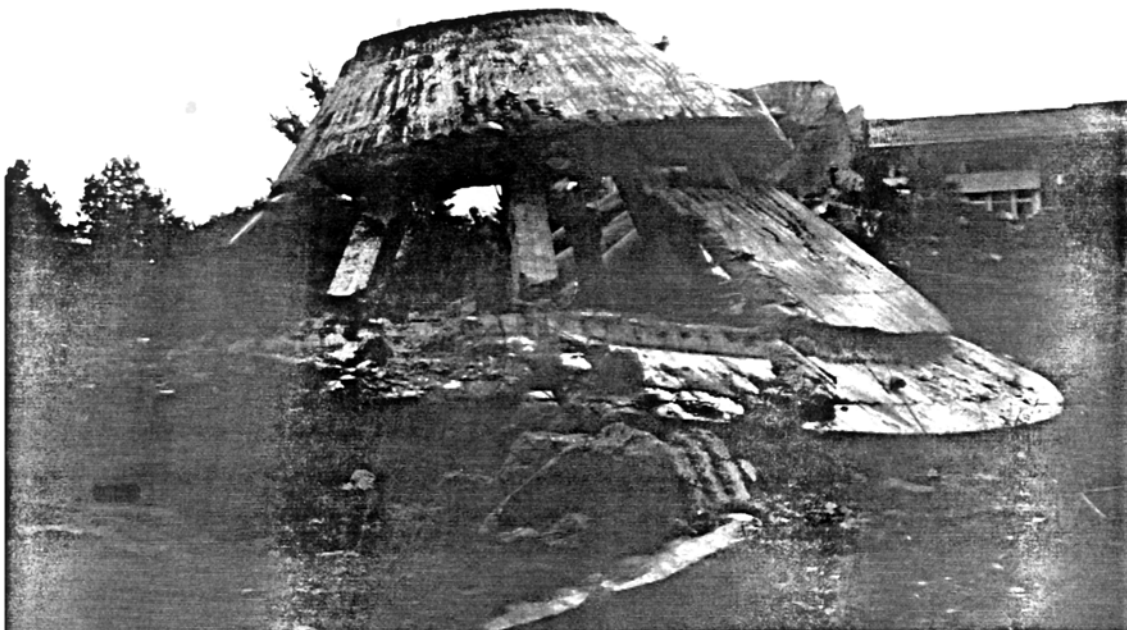
Picture 5.30 Concrete Water Tower No. 1, Rasht Secondary bending and buckling failure of tank columns due to impact
