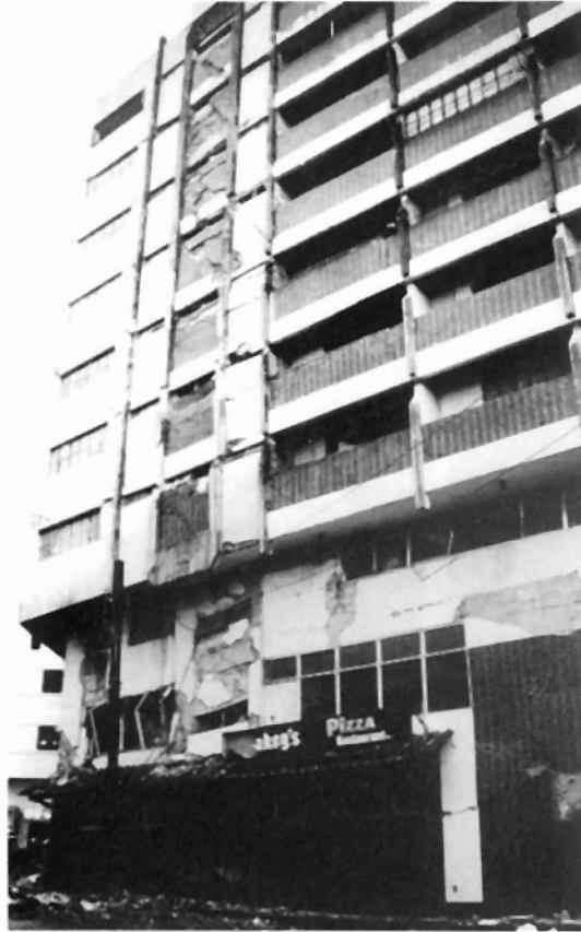
Figure 5.33 Damage to multistorey r.c. building, Baguio
