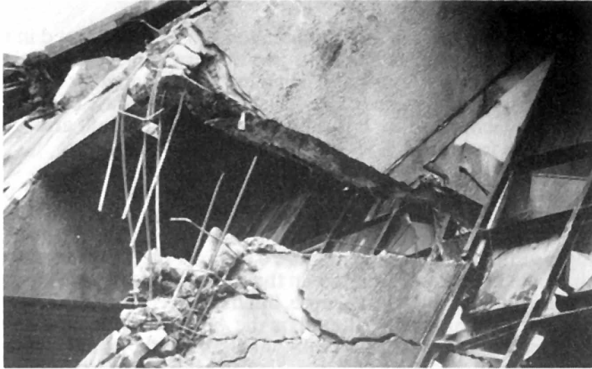
Figure 5.10 Failure of A-frame along construction joint, main hotel
