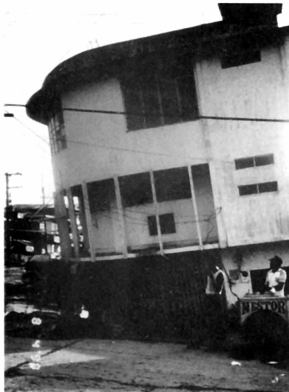
Figure 6.4 Foundation failure of building in Dagupan
