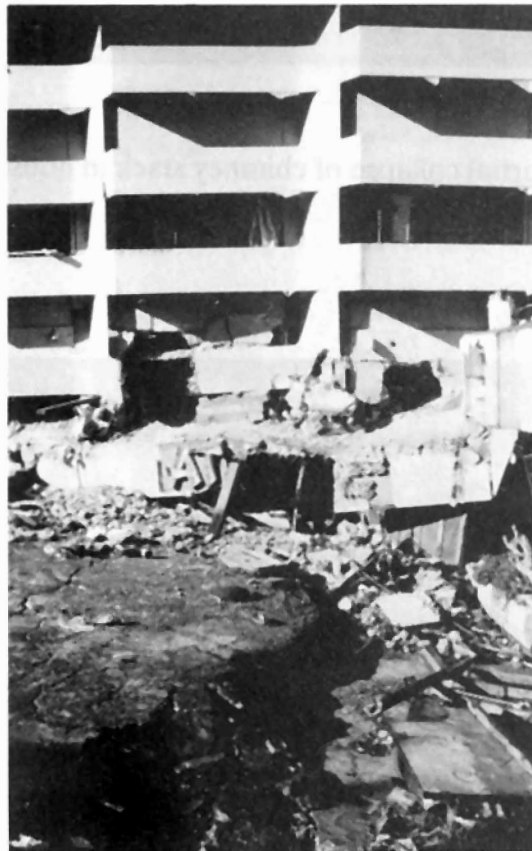
Figure 5.45 Ground settlement near Nevada Hotel, Baguio
