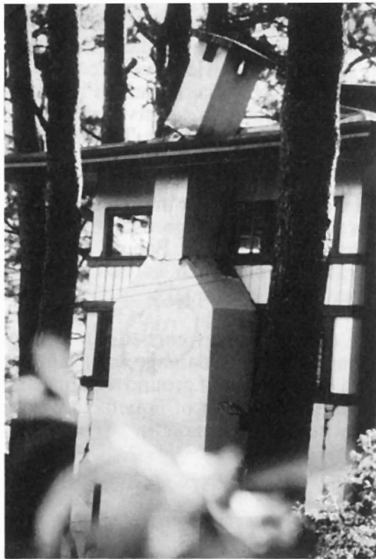
Figure 5.43 Partial collapse of chimney stack in house, Baguio
