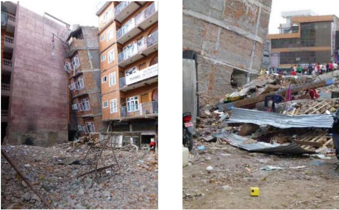
Figure 5-11 Fail at the base of the structure.
