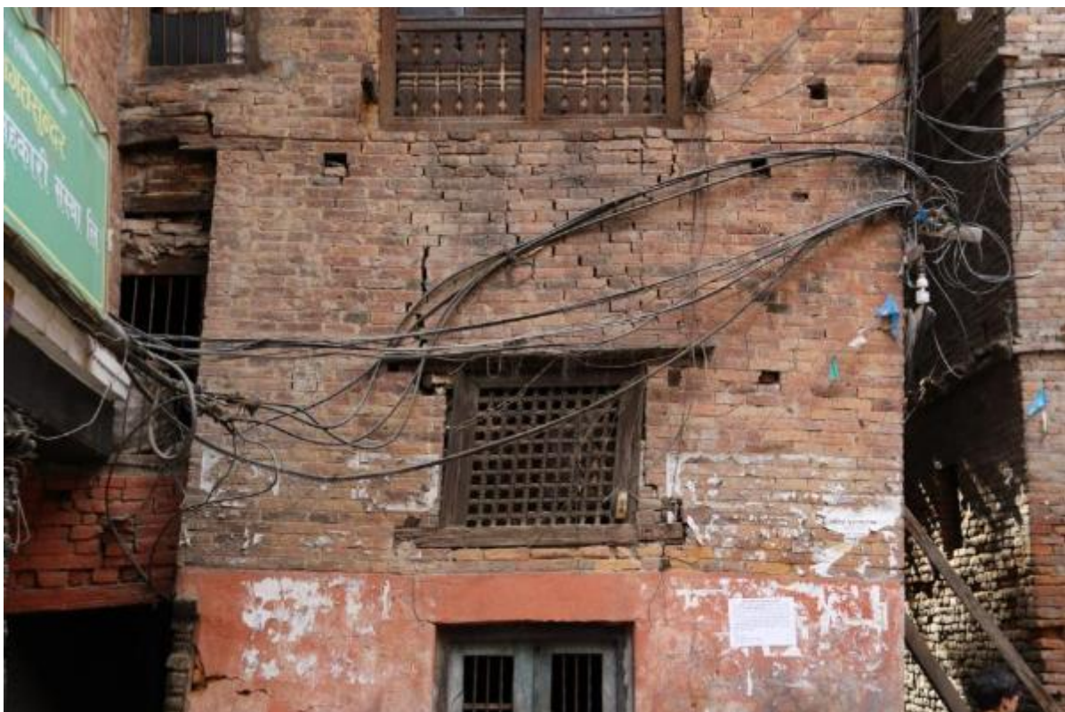
Figure 4-6 Example of In-plane shear failure of a typical Newari residence.
