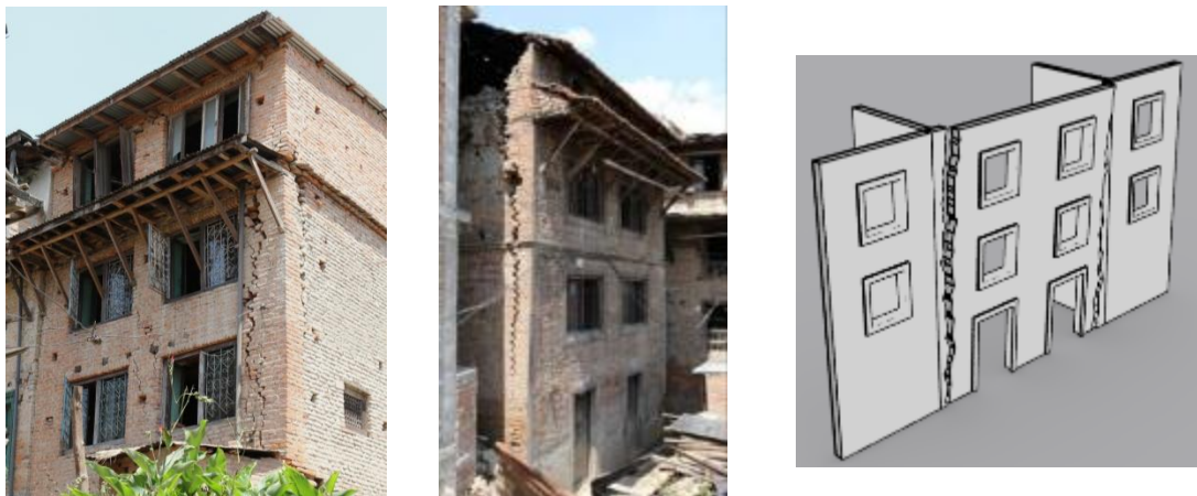
B2) Out of plane: Overturning due to insufficient connections on both sides of the facade
