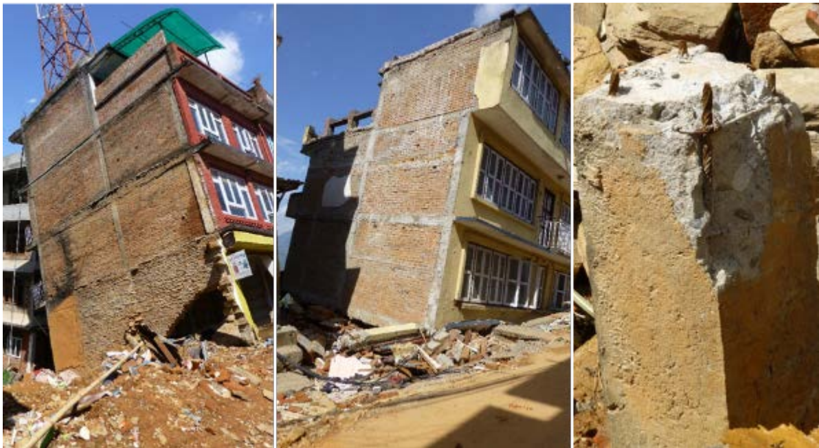
Figure 5-13 Building failures of Dolalghat region.
