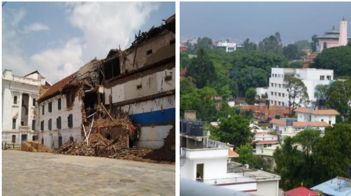
Figure 5-3 Damage in Durbar Square.
