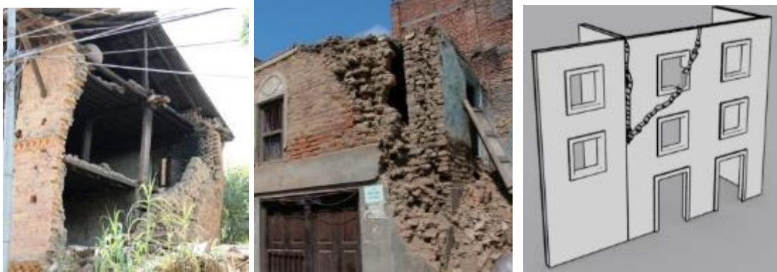
B1) Out of plane: Overturning due to insufficient connection of one side of the facade
