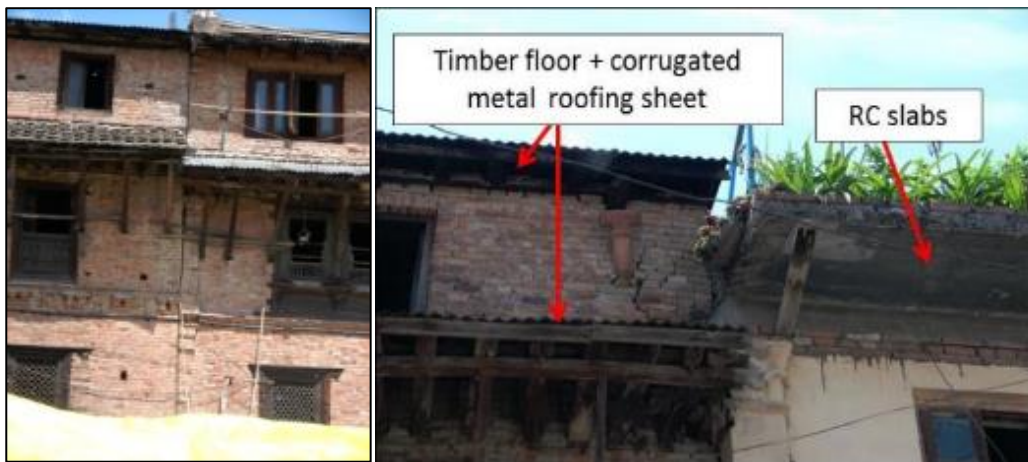
Figure 3-7 Absence of seismic gaps between buildings.
