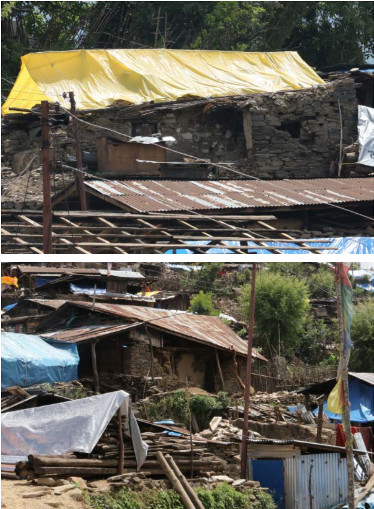
Figure 7-8 Building Damage in Lapsibot
