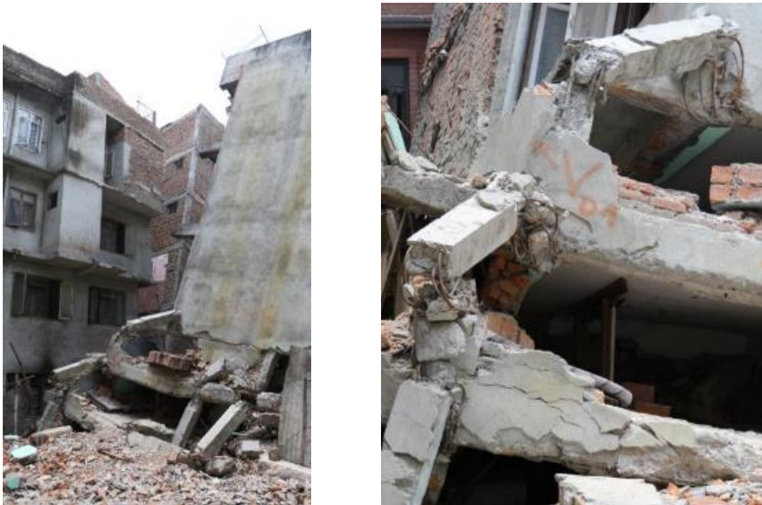
Figure 4-13 exemplifies the observed collapses with complete failure of the bottom storeys.
