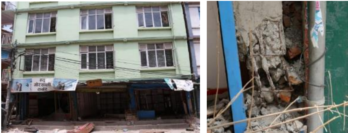
Figure 4-12. Examples of combined foundation bearing capacity failure. Left: Four storey building with soft storey failure. The gap to the right of the building did not exist before the earthquake. Right: Close up view of failure at the base of the right ground floor column.
