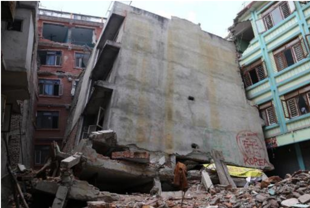
Figure 4-12 Exemplifies severe leaning.
