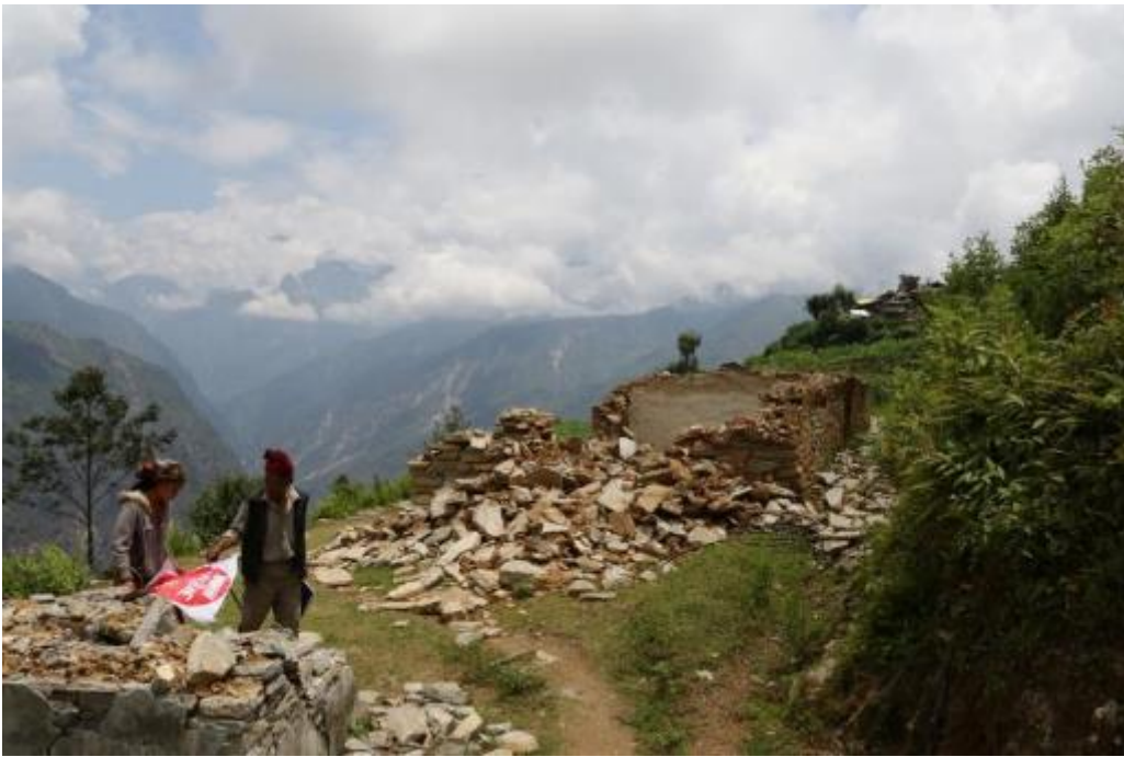
Figure 7-5 School building, showing complete collapse. This building was one of the most poorly constructed in the village with no cement used in the mortar.
