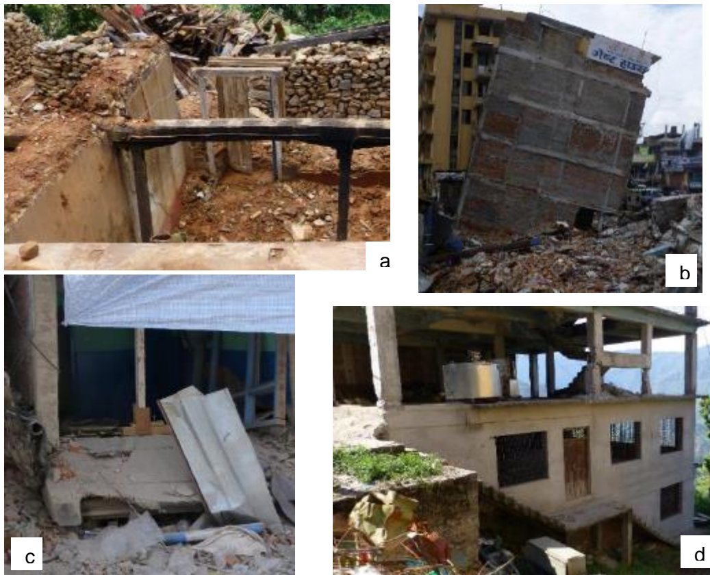
Figure 5-6 Failure of buildings that could be related to the foundation.
