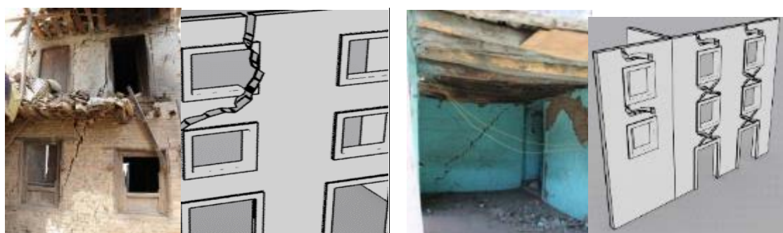
a) In plane failure (right: over multiple storeys; left: single wall beneath extremely heavy floor)
