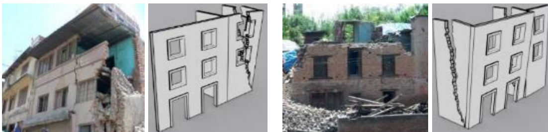
C1) Combined failure: Corner failure overturning of two facades
