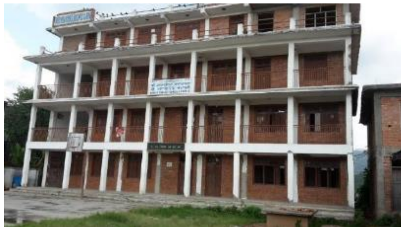
Figure 6-5 A Four storey RC framed building with fired clay masonry infill. Building constructed in 2010 without any seismic consideration. On the same site there is another school building designed with some limited seismic consideration following the 1988 earthquake, illustrating that seismic design awareness apparently reduced as the memory of the last earthquake dimmed. This is also symptomatic of weak enforcement of building regulations.
