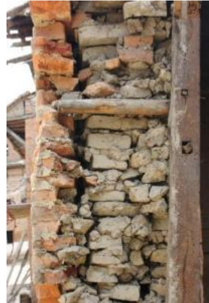
Figure 4-5 Decay and delamination between wall wythes. Examples of sorted timber that showed decay and delamination between wall wythes made from different materials.
