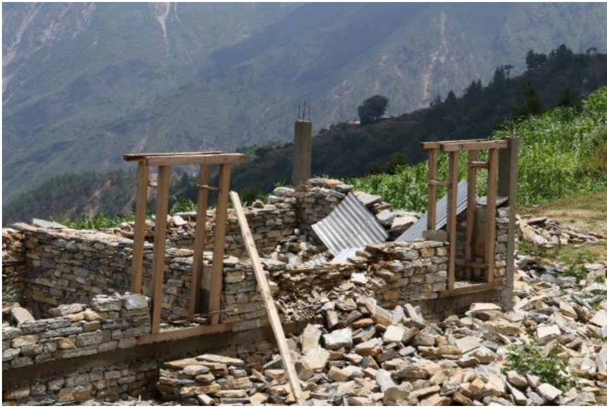
Figure 7-7 School building damaged.
