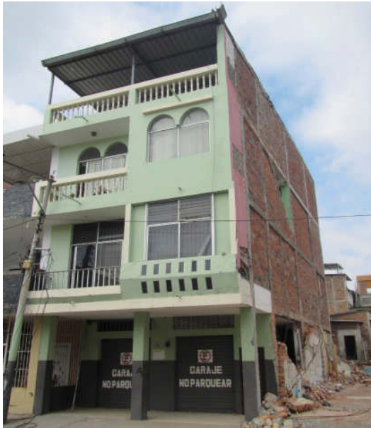
Figure 11 - Light metal roof addition, Manta, Tarqui ©EEFIT
