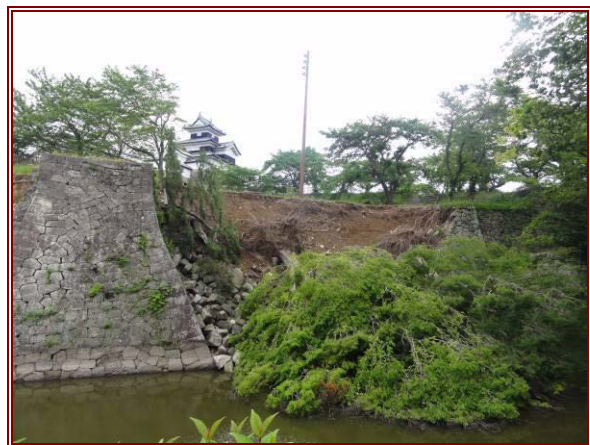
(b) Collapse of stone wall
