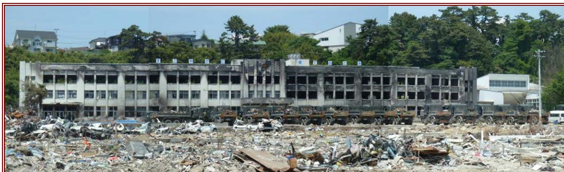
Figure 10.8 Fire damaged school, Ishinomaki City. It is not known whether this building was used as an evacuation refuge during the tsunami.
