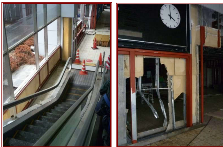
Figure 7.66 (left) View to ground floor showing damaged escalator and glazing, and 3.5 m high watermark on glazing.
