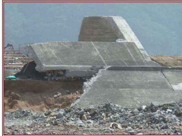
Figure 6.4 Unreinforced concrete interlocking blocks and sand infill of the sea wall at Tarō.
