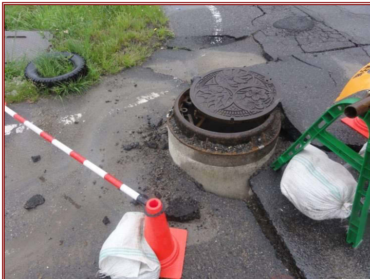
(a) Uplift of manhole
