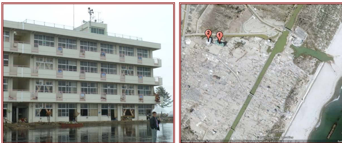
Figure 10.22 (left) The south face of Arahama Elementary School. Sirens and steel bracing are visible (2 instances, in the lower three storey windows), as is damage to the ground floor.
