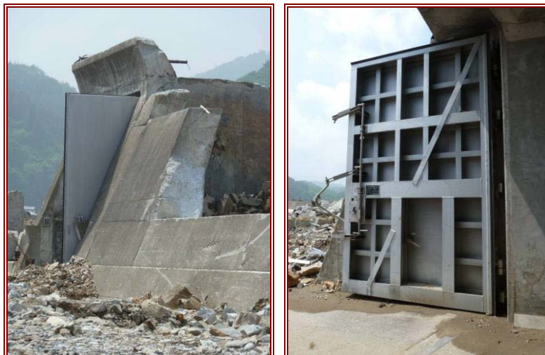
Figure 6.5 (left) Remaining buttress supports around a tsunami gate in the sea wall at Tarō.
