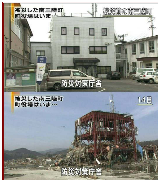
Figure 7.30 Crisis Management Department of Minamisanriku Town, which shows the building before and after the tsunami (Anon., 2011b).
