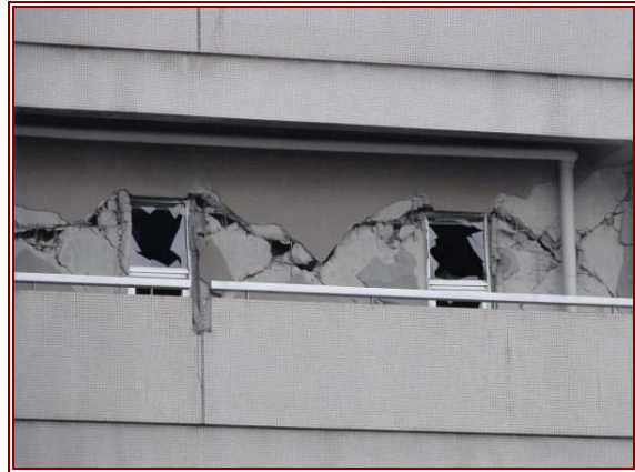
(b) Large diagonal cracks on wall
