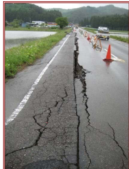
(b) Lateral spreading
