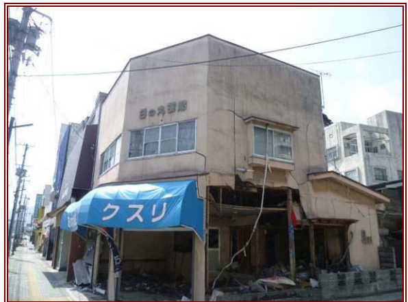
(f) Timber frame, D3, 3 m inundation.
