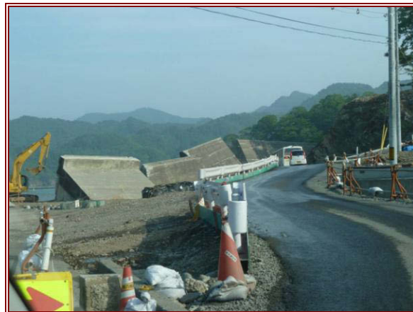
Figure 6.12 Toppled concrete blocks from the seawall in Ryoishi.
