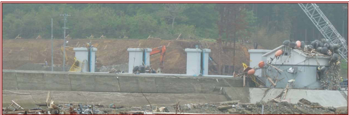
Figure 6.25 Damaged tsunami gates on the Mizushiri River in Minamisanriku.
