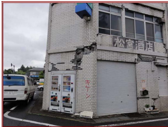
(e) Damaged liquor store
