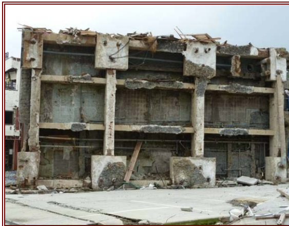
Figure 7.42 (left) Foundations of the overturned building D.
