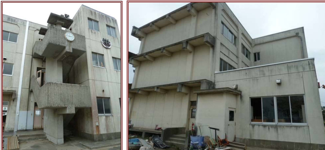
Figure 10.24 (left) Minor earthquake damage at seismic detailing of Yuriage Junior High School: the staircase moved independently of the main building, and horizontal movement was accommodated in the separation joint shown by the vertical silver strip from ground to roof level.
