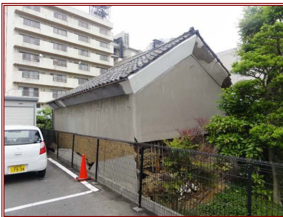
(a) Damage to traditional warehouse
