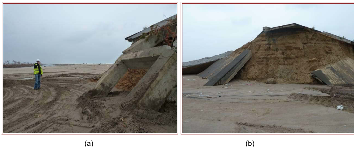
Figure 6.15 Catastrophic failure of the concrete block revetment at Yamamoto-cho.
