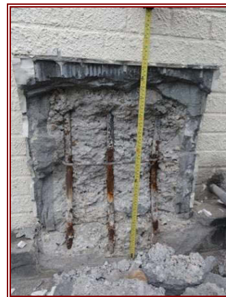
(f) Falling of concrete cover
