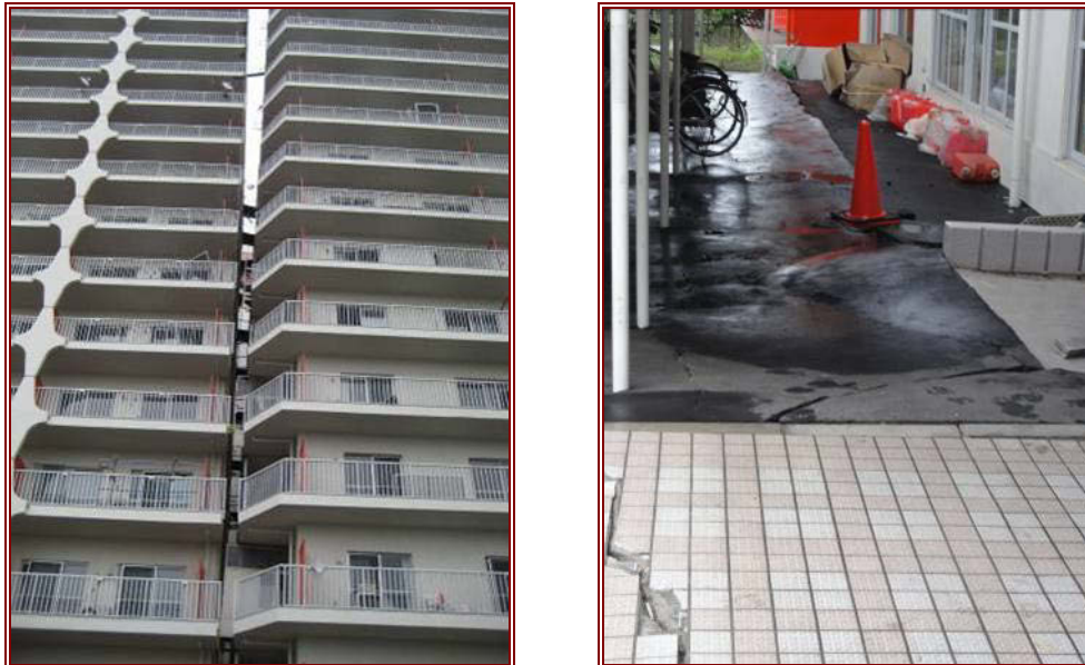
(a) Left block has tilted due to differential settlement (b) Ground settlement adjacent to building
