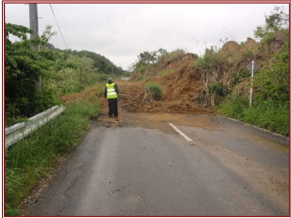
(b) Road buried by landslide debris
