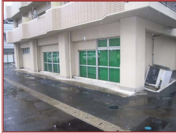
Figure 8.2 Settlement of a 6-storey building in Yamoto-machi, Sendai City.
