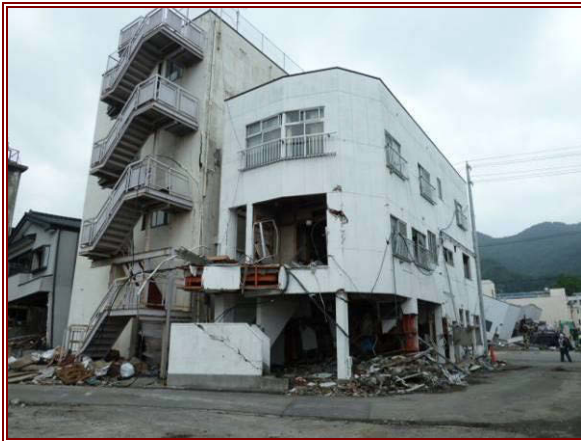
(c) Steel frame, D2, 7 m inundation.
