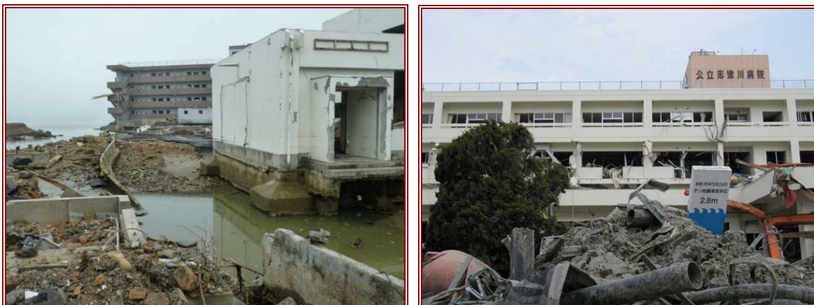
Figure 7.33 (left) Significant scour in Shiomi-cho, adjacent to the former gymnasium building, 100 m from the sea. Significant scour also occurred at the apartment block (a designated vertical evacuation structure) visible in the background. This structure is discussed further in section 10.3.3.
