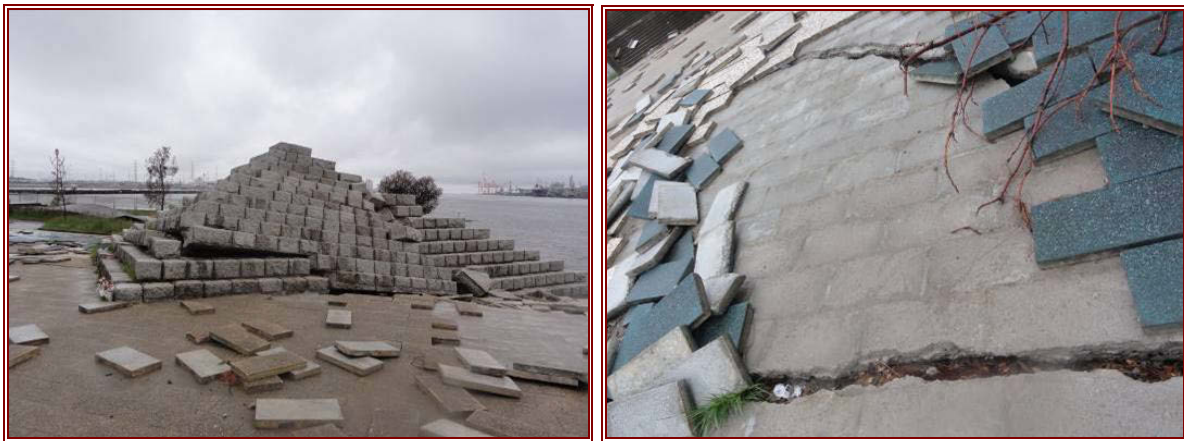
(a) Lateral spreading at the port edge
