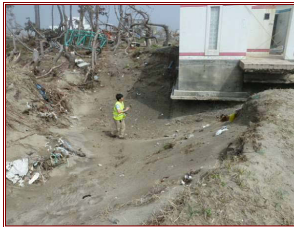
Figure 7.55 Extreme scour of approximately 86 m 2 around a toilet block constructed on sandy soil with shallow foundations. This building is 40 m landward of sea defences at Wakabayashi-ku.
