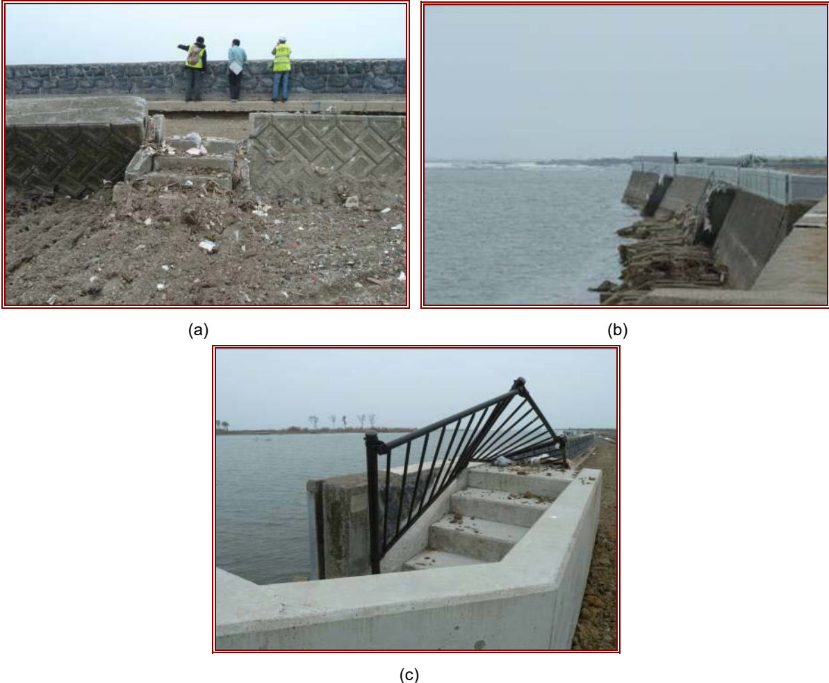
Figure 6.28 Damage to river defences on the south side of the Natori River in Yuriage.
