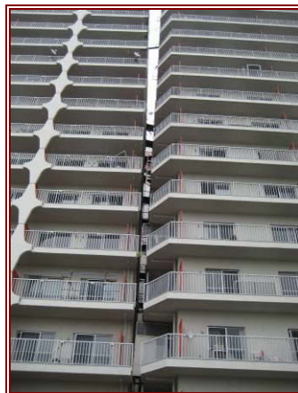
(f) Gap between two buildings
