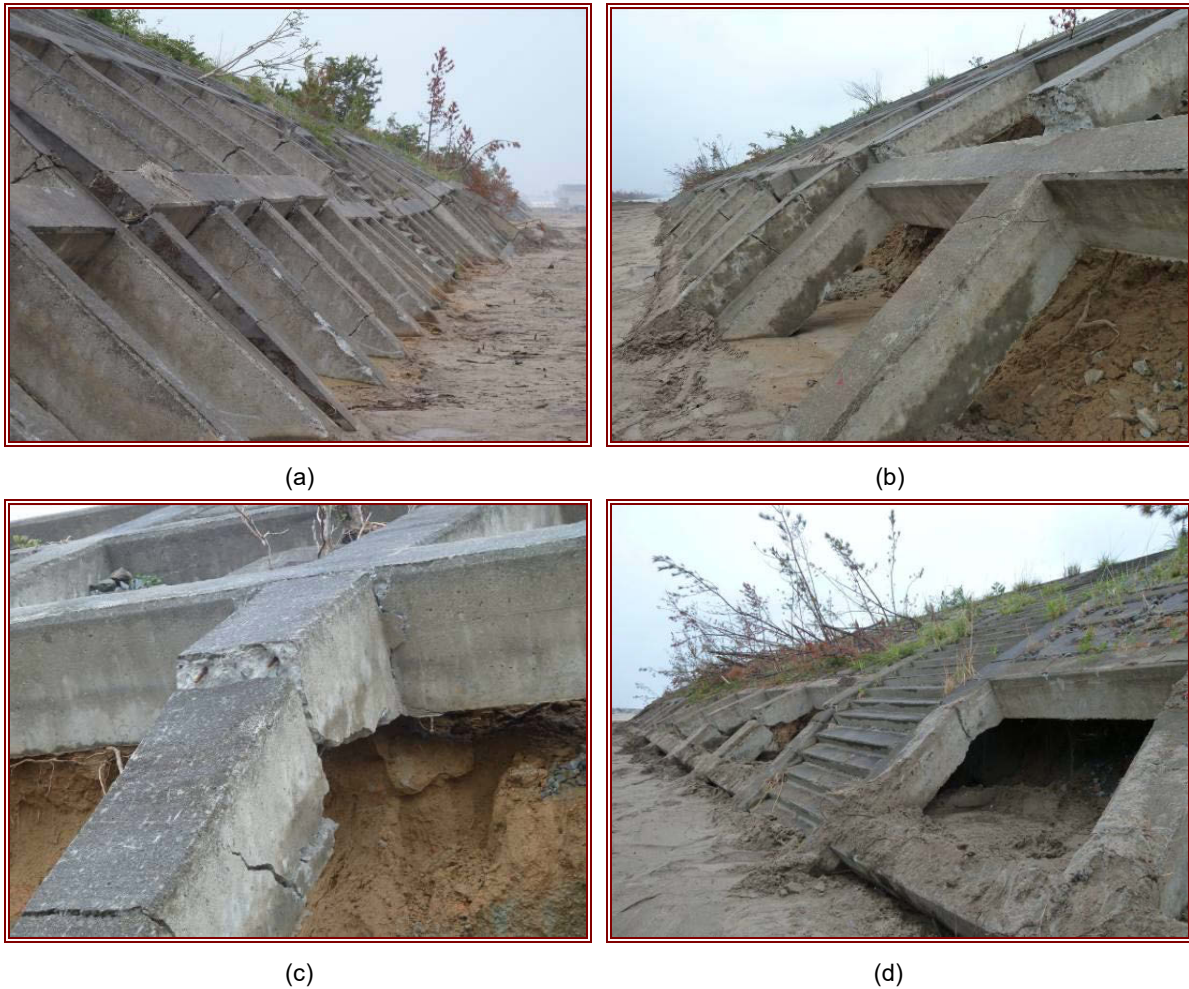
Figure 6.14 Inland side of concrete block revetment at Yamamoto-cho. (a) to (c): Breaks in the lattice revetment. (d): Sand in-fill wash-out.
