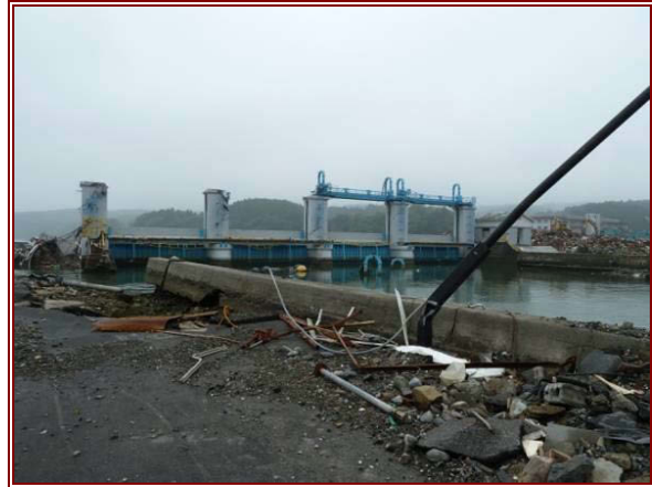
Figure 6.24 (right) Damaged tsunami gates at the mouth of the Hachiman River, Minamisanriku.
