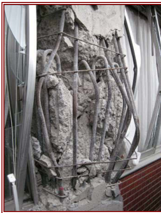
(c) Shear failure of a column
