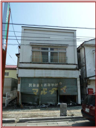
(a) Timber frame structure, damage D1, 3 m inundation.
