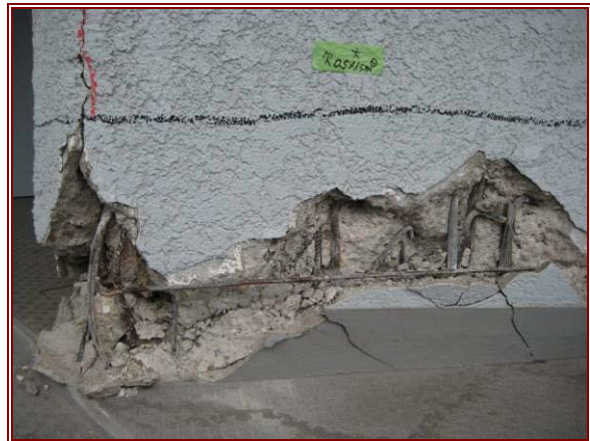
(b) Column-floor joint failure
