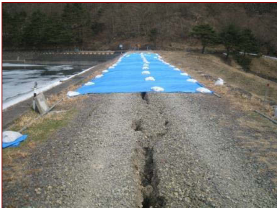
Figure 4.18 Covering the cracks on the crest of Nishigo Dam to prevent water intrusion (Matsumoto, 2013).
