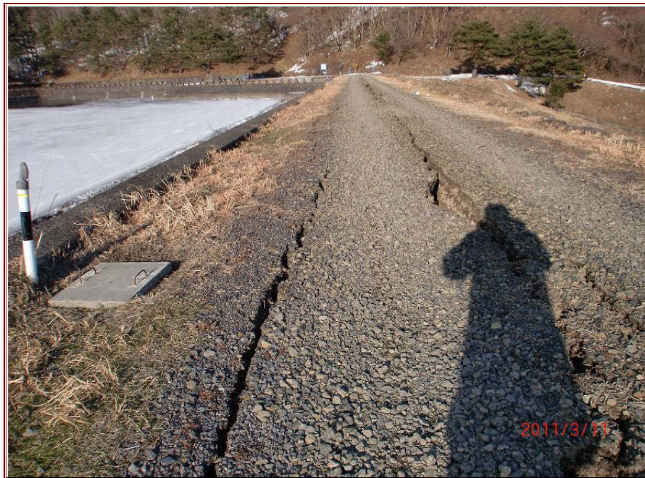
Figure 4.17 Cracks in the crest of Nishigo Dam observed immediately after the earthquake on March 11, 2011 (Matsumoto, 2011).
