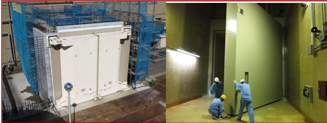
Figure 4.13 External and internal reinforced doors for reactor buildings at Hamaoka NPP (reproduced from Hamaoka, 2013).
