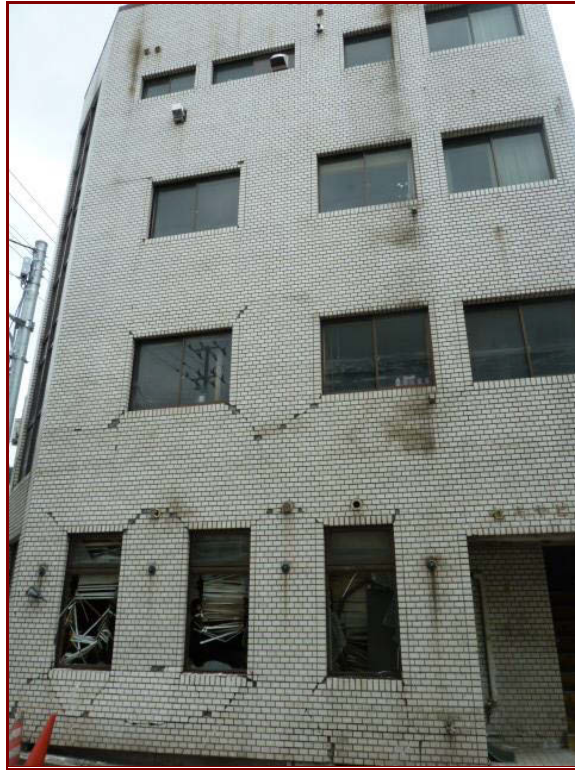
Figure 2.11 Additional seismic damage indicated by conjugate shear cracking of facade in Kamaishi.
