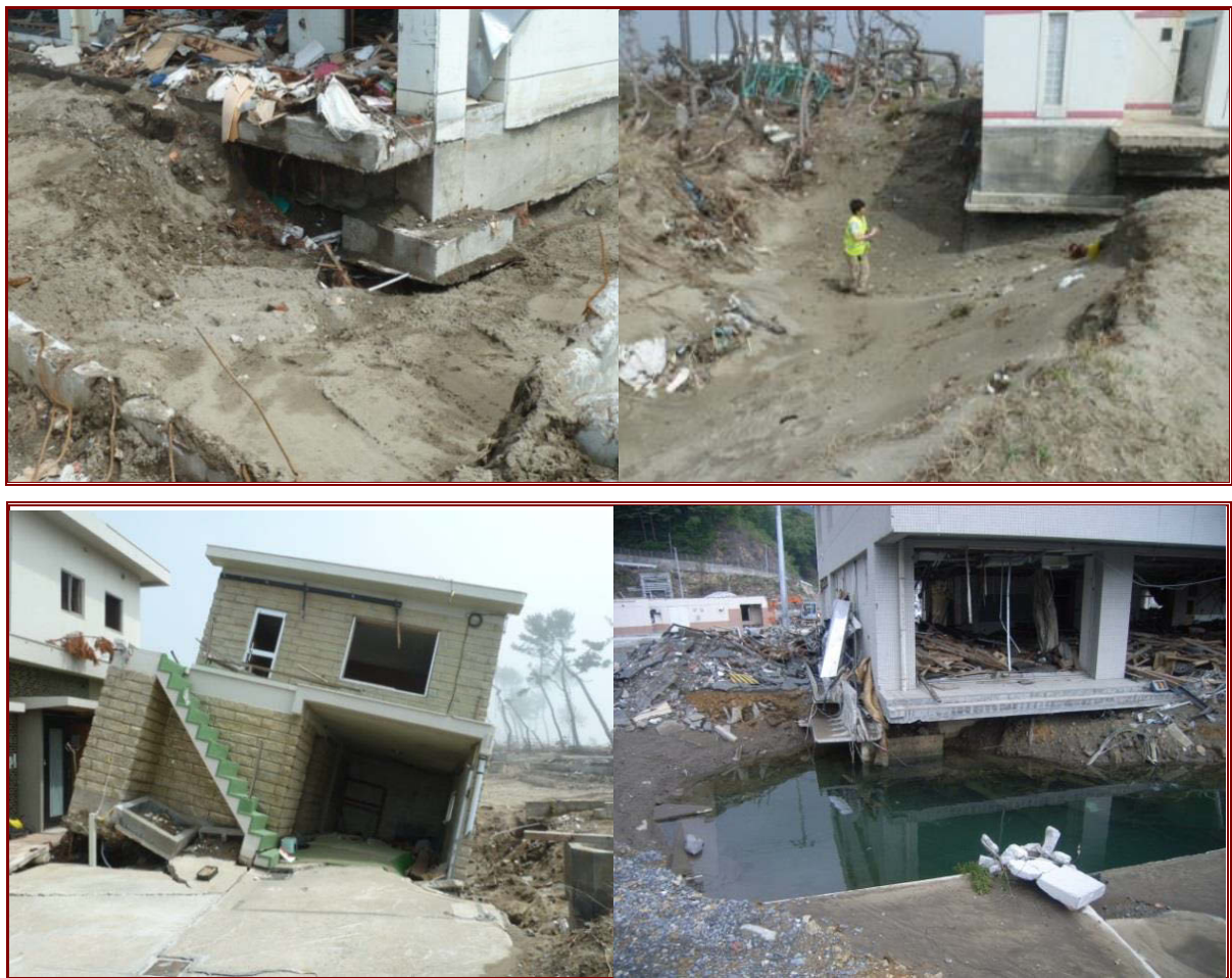
Figure 2.9 Scour undermining foundations building corners.
