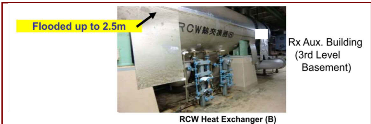
Figure 4.6 Internal Flooding on the Heat Exchanger of Unit 2 (extracted from (Kato, 2013)).
