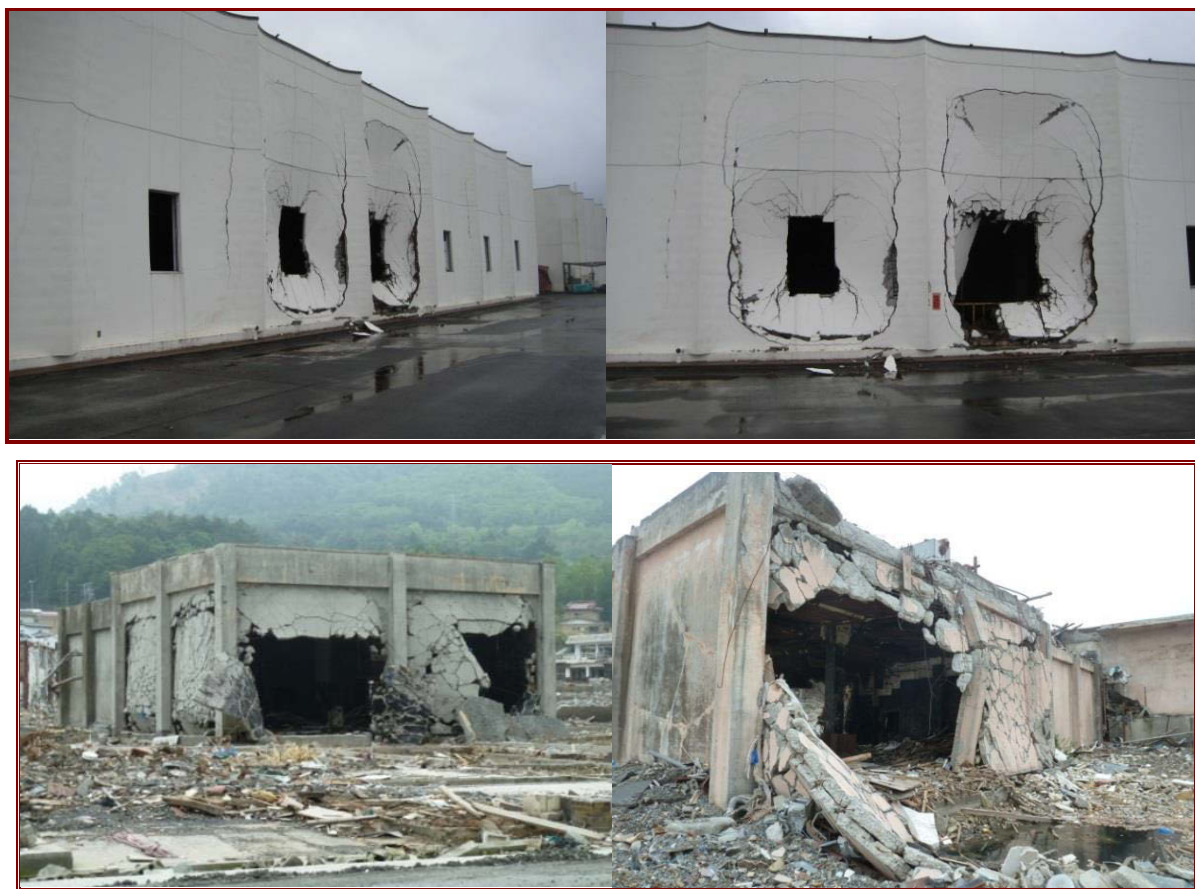
Figure 2.4 Out-of-plane failure of walls due to lateral fluid load (hydrostatic and hydrodynamic).
