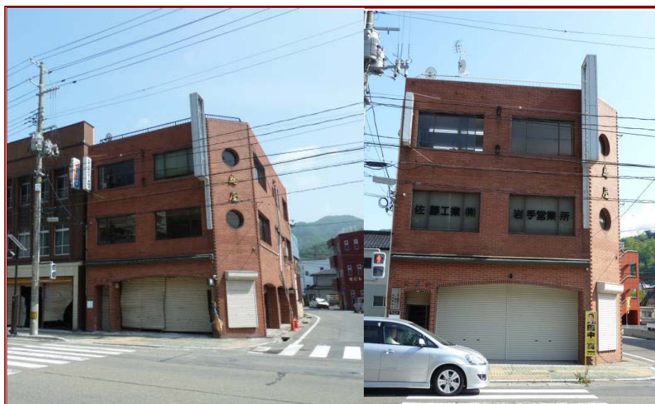
Figure 2.17 Retained building where inundation did not reach the 2nd floor, in 2011 (left) and 2013 (right). Note the adjacent building (which experienced the same inundation) has been demolished.
