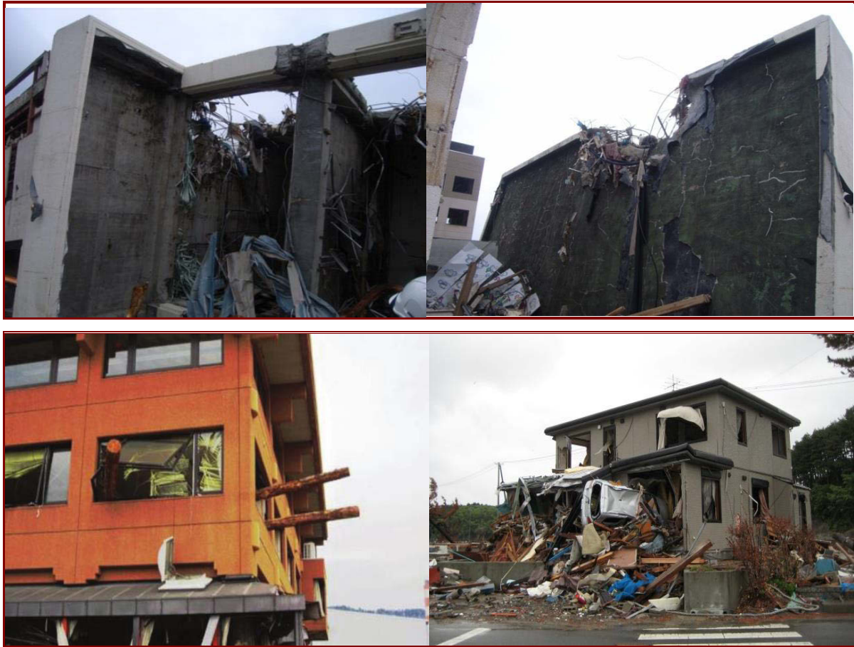
Figure 2.6 Damage due to debris impact and damming.
