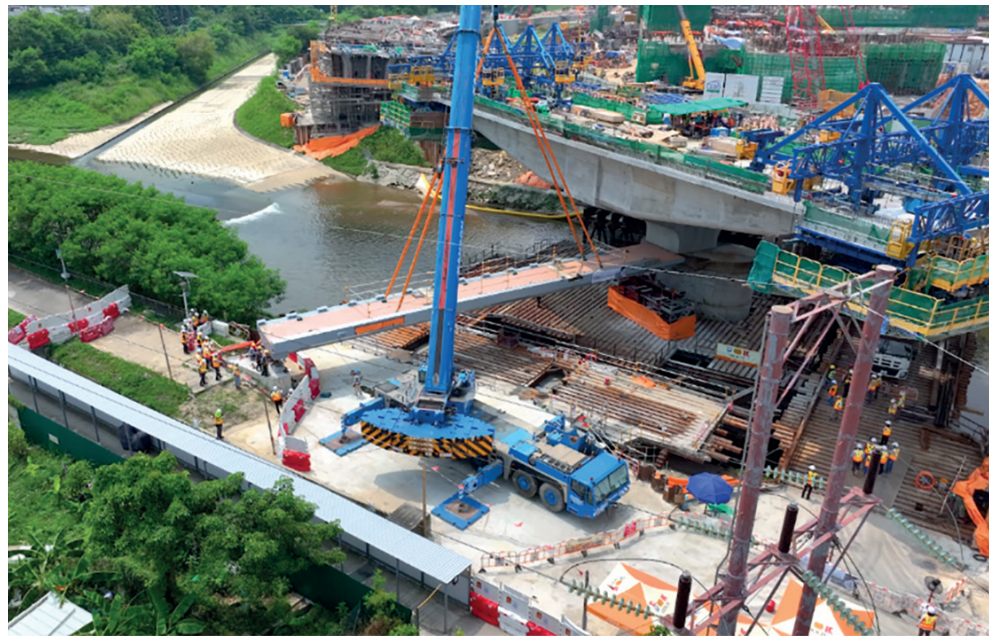
➤ FIGURE 13: Lifting and installation of segment of Footbridge F4 with length of 34.1m
