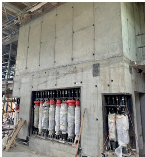
↑ Resistant slip friction joint damping devices were used to convert original design to rocking wall structure
