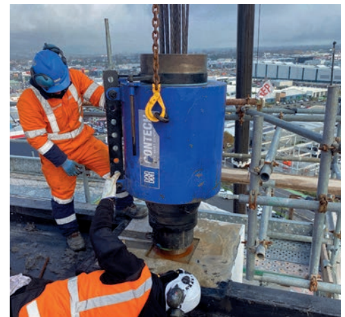
↑ Anchor strands were inserted from top of column core holes and anchored at base above rocking plane
