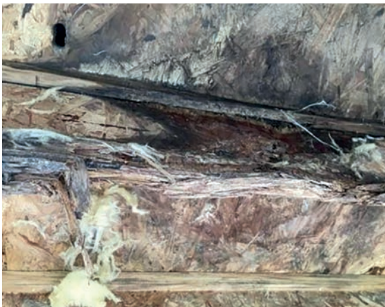
↑ FIGURE 1: An example of OSB board deterioration
