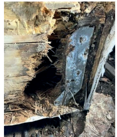
↑ FIGURE 3: Engineered timber joist deterioration
