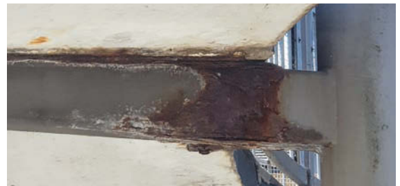
↑ FIGURE 1: Corroded cantilever deck support
