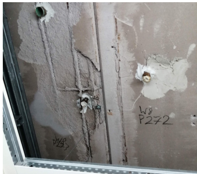
Damage caused by drilled holes for services penetrations.
