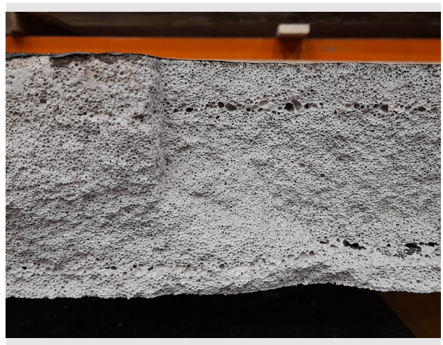
Photo showing bubble formation on reinforcement
