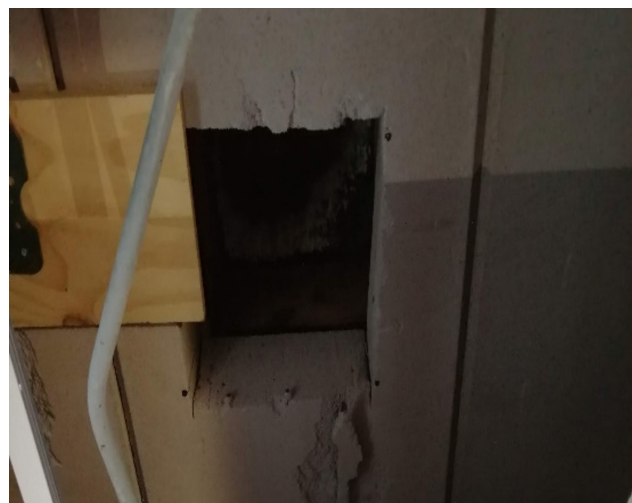
Damage caused by roof vent installation
