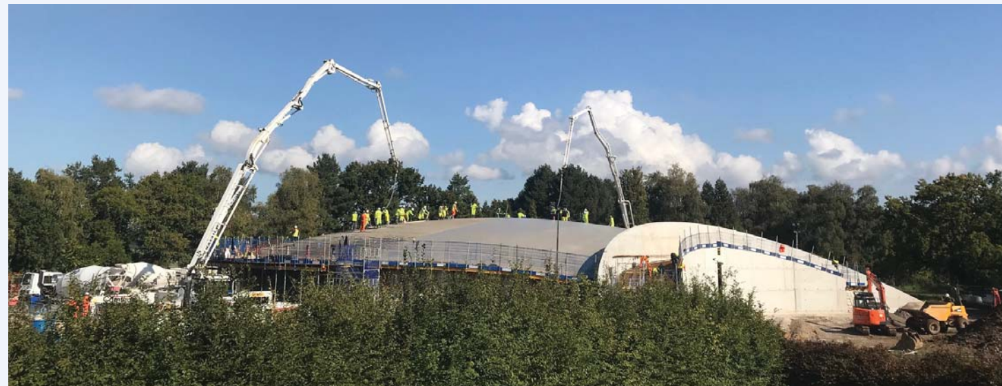
Figure 3. Photo from site
