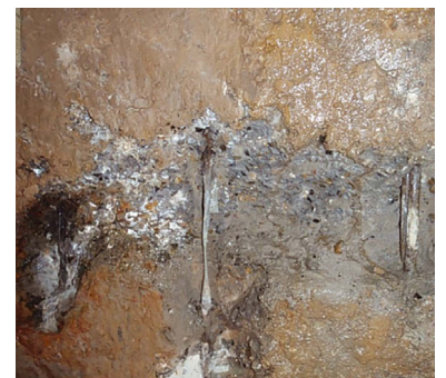
FIGURE 3: Exposed pile cap indicating potentially serious durability issue to steel reinforcement
