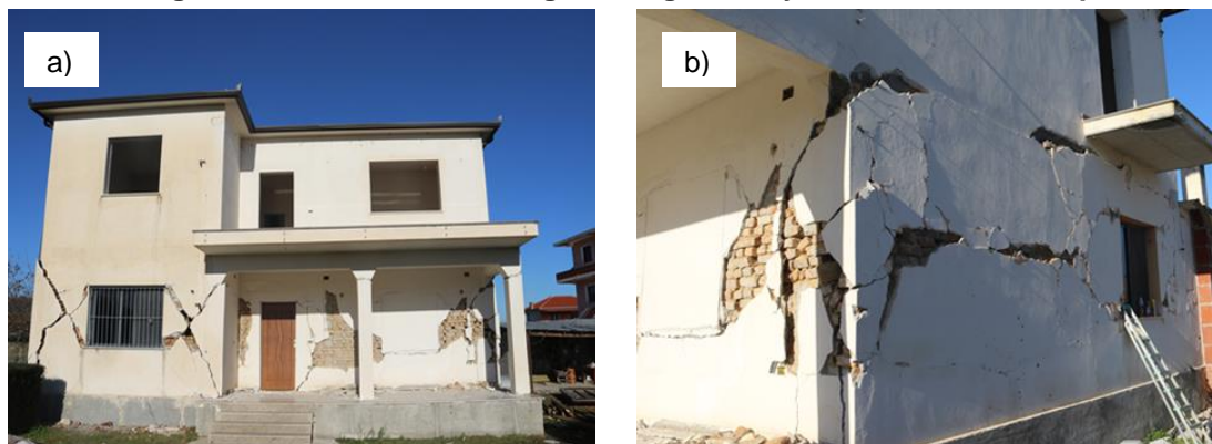
Figure 7.32: Extensive damage in single-family rural house in Bubq
