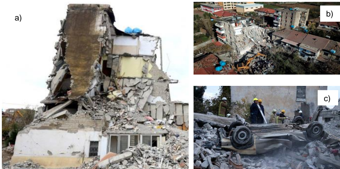
Figure 7.6: a) Collapsed 5-storey URM building in Thumanë; b) view from the air of the collapsed building in Thumanë; c) destruction in the town of Thumanë, one of the worst affected areas
