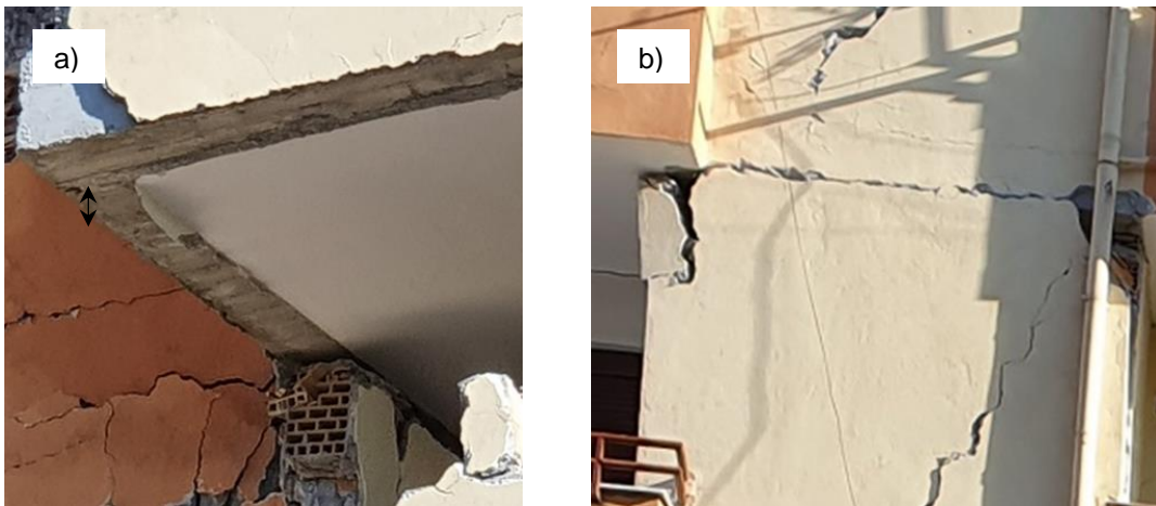
Figure 7.21: Typical 2000s multi-storey RC building compliant with KTP-N.2-89: a) collapse of the infill panel; b) detachment of the infill panel and formation of horizontal cracks
