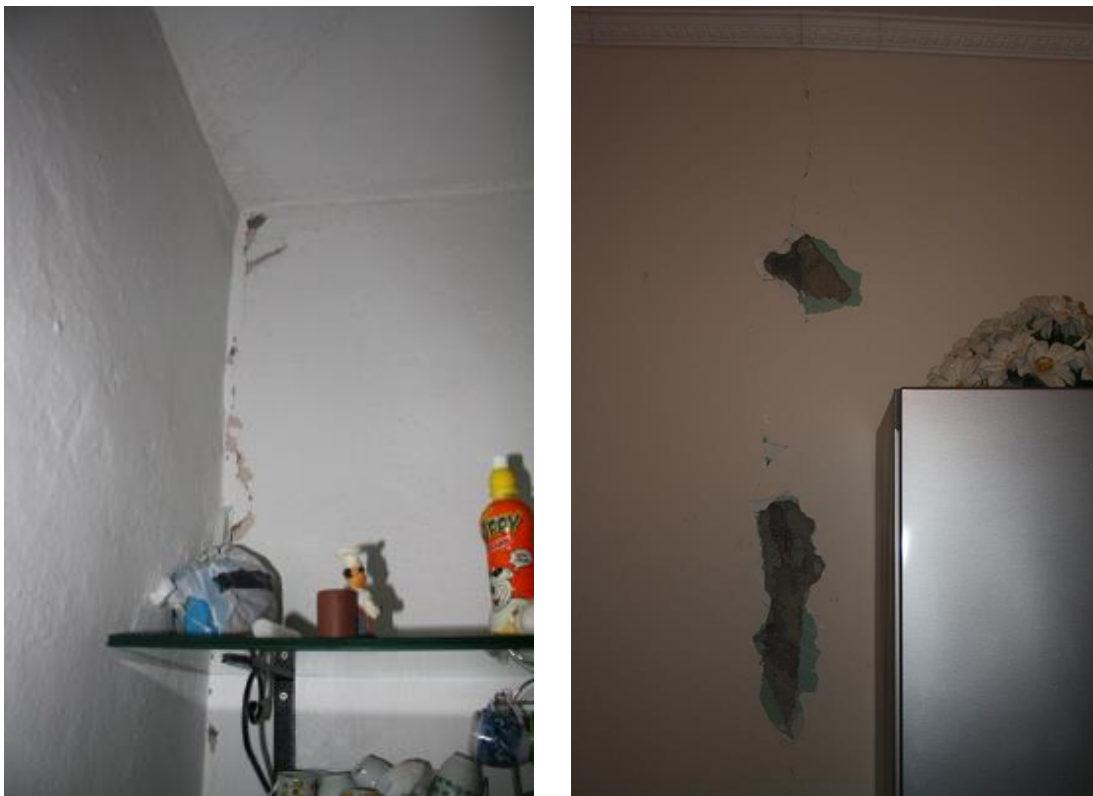
Figure 7.14: LPBs in Laç (Module 1, two sections): Vertical cracks formed in the interface between wall panels
