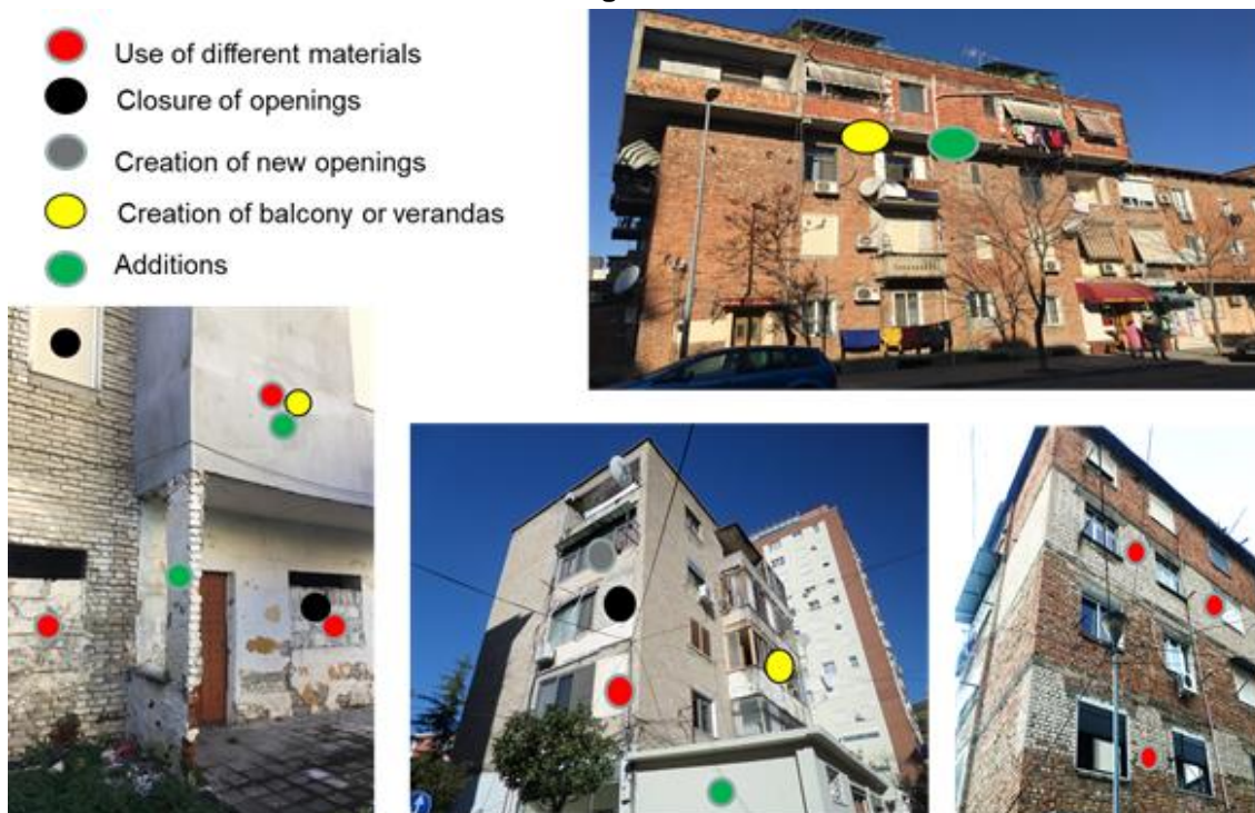
Figure 7.5: Irregularities in elevations due to unauthorised interventions on URM buildings in Durrës
