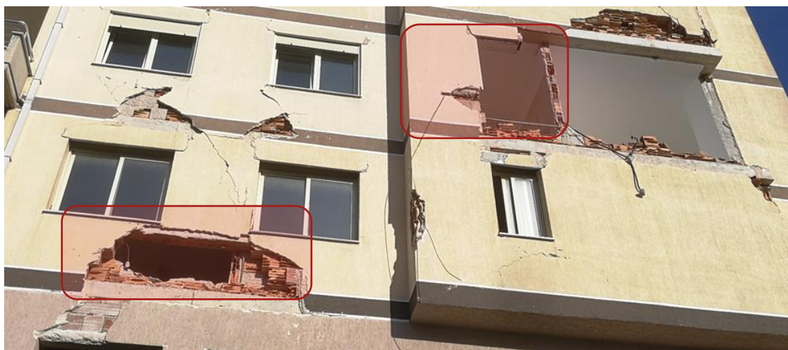
Figure 7.28: Typical post-2010 multi-storey RC building compliant with KTP-N.2-89 with integrated aspects of Eurocode 8. Effects of the belt beams in confined and unconfined infills.
