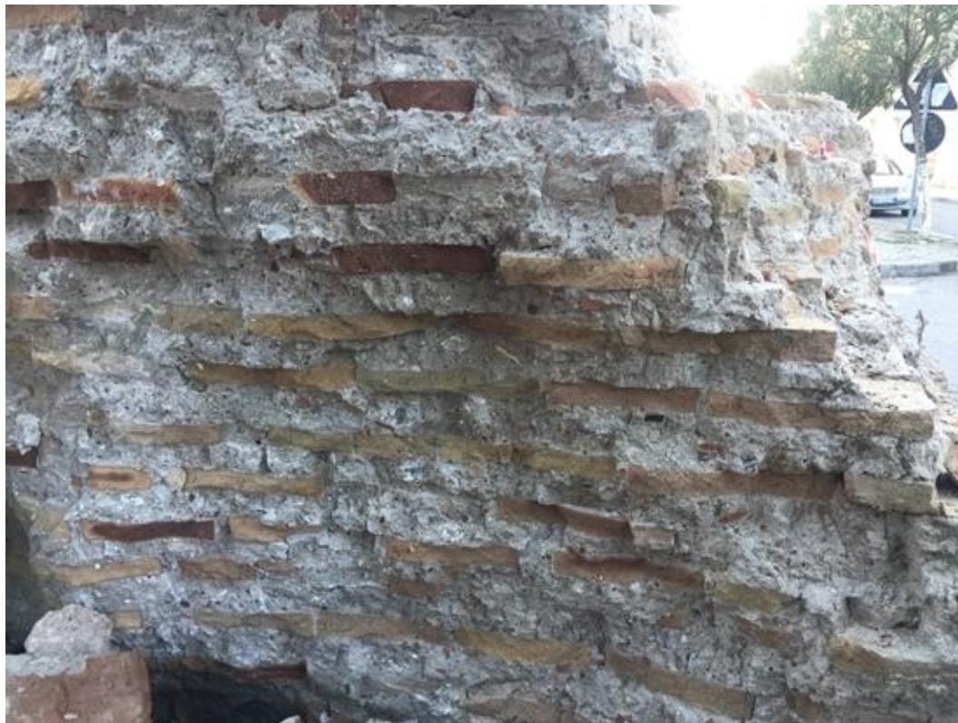
Figure 7.37: Close view of the collapsed masonry in Durres
