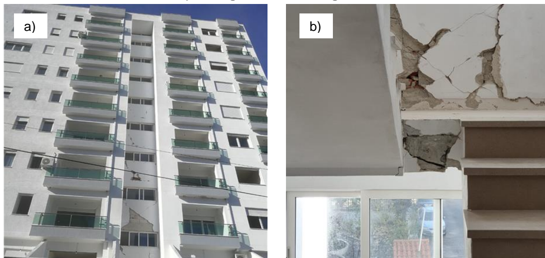
Figure 7.25: Typical post-2010 multi-storey RC building compliant with KTP-N.2-89 with integrated aspects of Eurocode 8: a) exterior damage related to the interaction with the stairs; b) damage on the landing of the stairs
