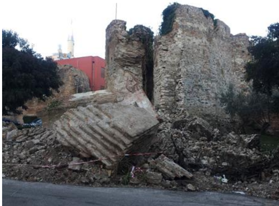
Figure 7.36: View of the surfaces of rupture of the gate tower
