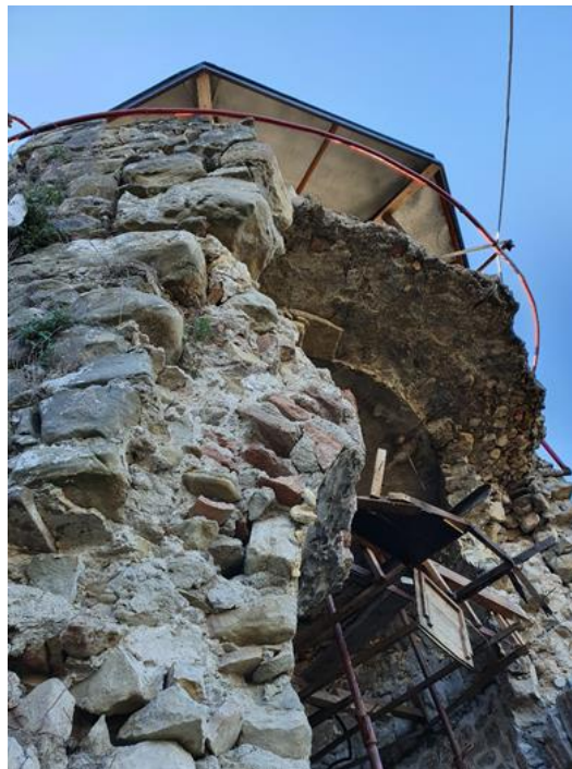
Figure 7.51: View of the damage to the Prezë clock tower
