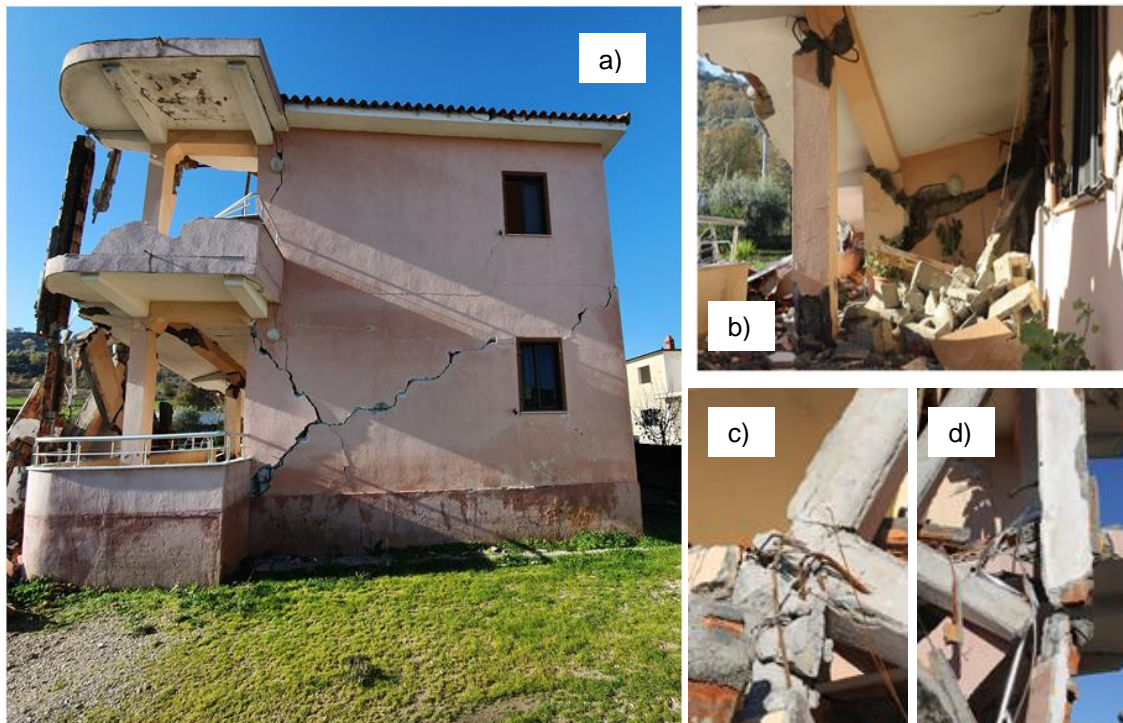
Figure 7.31: Collapsed single family rural house in Bubq: a) severely damaged side façade b) internal view of the failed portico, c) and d) details of the poor reinforced columns of the portico at the joint connections.
