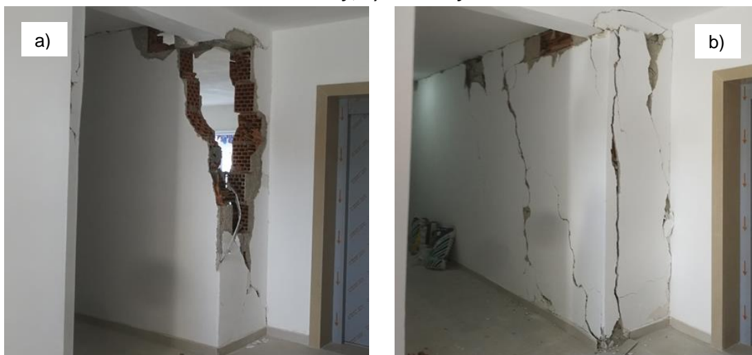
Figure 7.26: Typical post-2010 multi-storey RC building compliant with KTP-N.2-89 with integrated aspects of Eurocode 8. Unconfined internal infill showing damage at the a) 2 nd storey; b) 5 th storey
