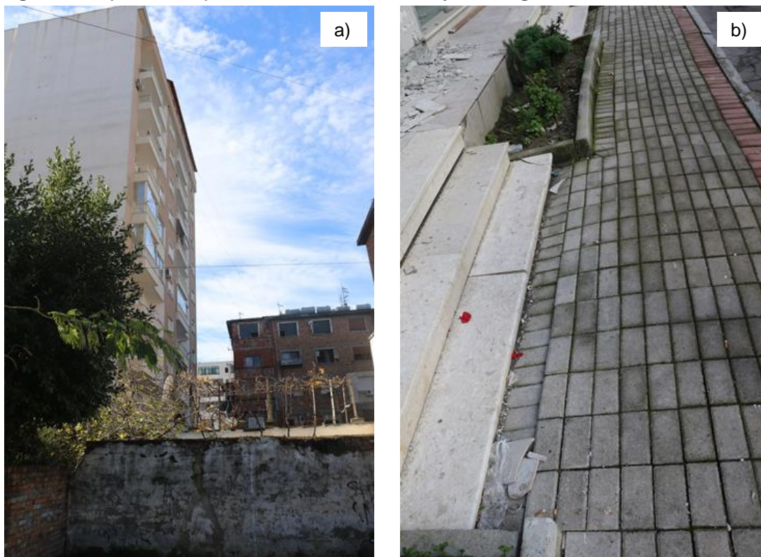
Figure 2.9: a) Tilt and b) subsidence of multi-storey building due to soil reconsolidation
