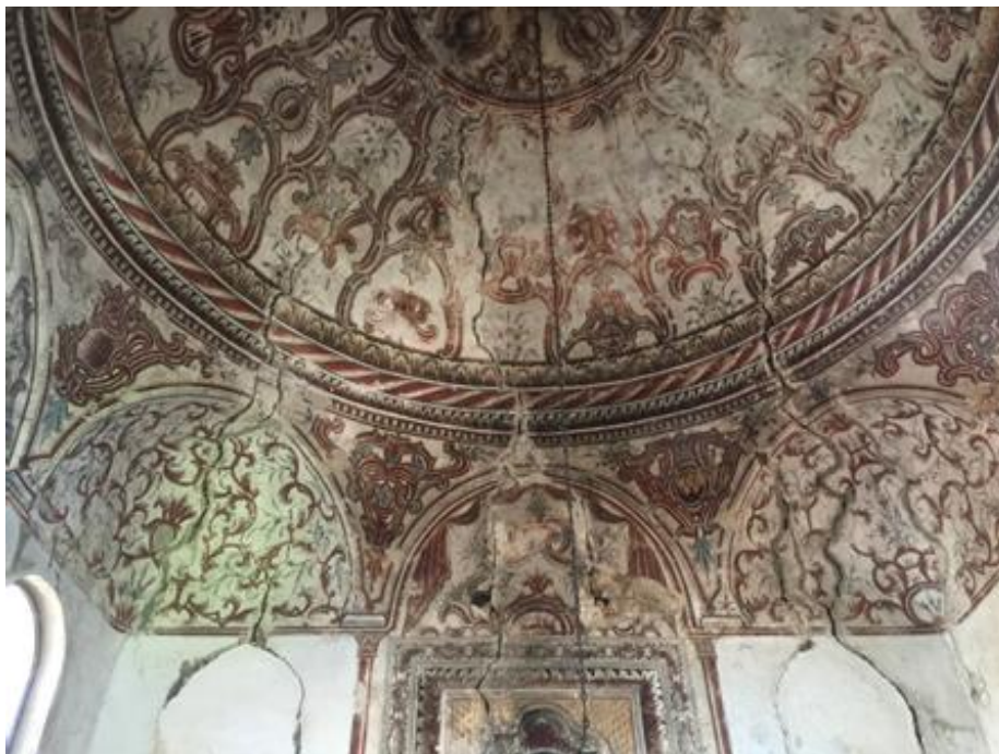
Figure 7.43: View of the cracking of Tekke of Dollma dome
