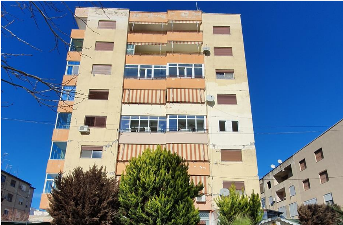
Figure 7.22: Typical 2000s multi-storey RC building compliant with KTP-N.2-89: damage layout on the eastern façade of the building
