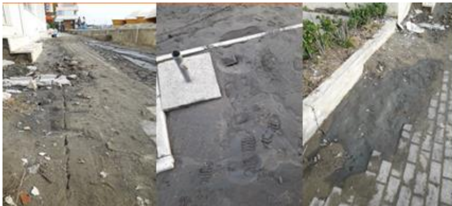
Figure 2.8: Surface manifestation of liquefaction along Durrës beach
