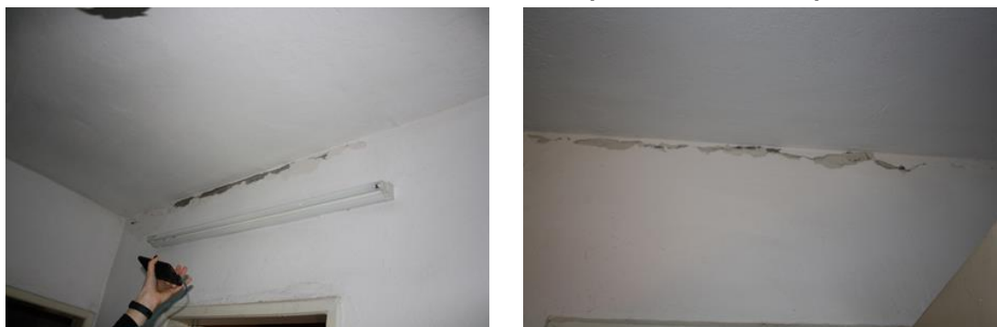
Figure 7.16: LPBs in Durrës (Module 2 with one, two & three sections): horizontal cracks formed in the interface between the wall panel and the floor panels
