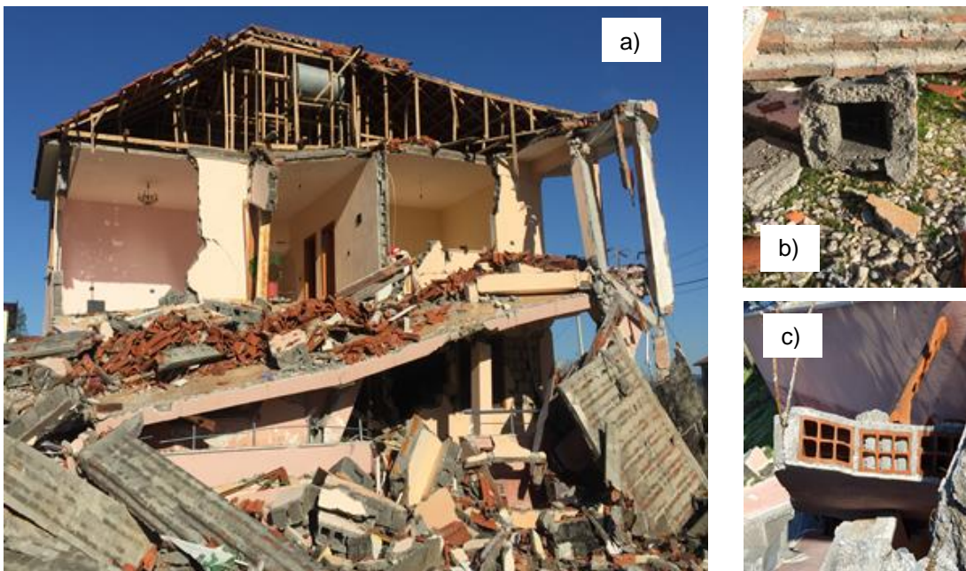
Figure 7.30: Collapsed single-family rural houses in Bubq. URM building with hollow concrete blocks and RC slab at the 1 st level and hollow brick waffle concrete slab at the 2 nd level
