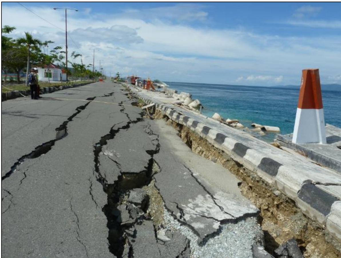
Figure 5.17 - Cracks parallel to coastline, consistent with lateral spreading of the ground.
