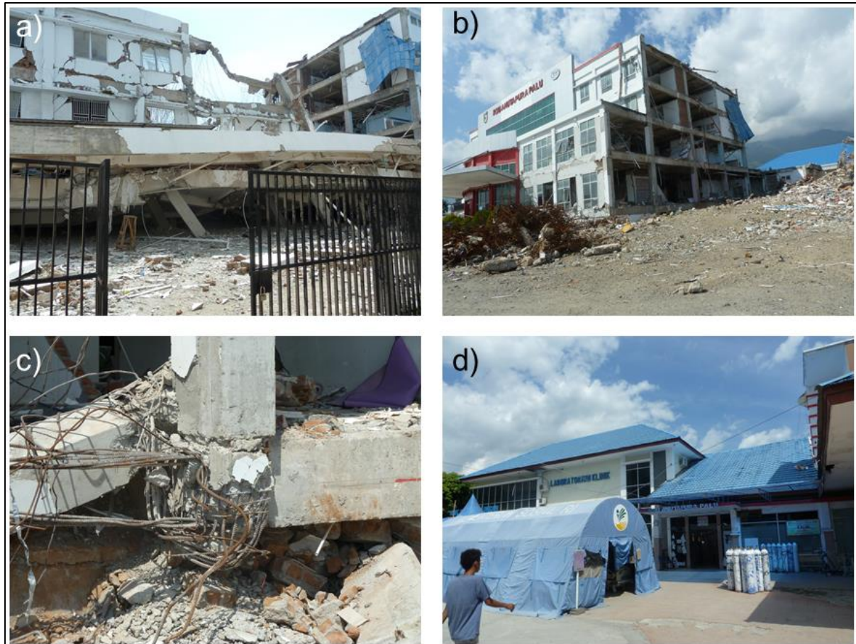
Figure 7.40 - Damage at Anutapura Hospital a) soft story collapse of four story RC frame structure; b) RC frame of remaining structure visible following removal of collapsed debris; c) column=beam joint reinforcement exposed in collapsed structure; d) low-rise hospital structures were relatively undamaged and remained operational.
