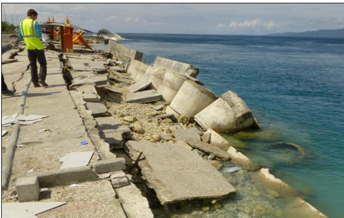
Figure 5.18 - Failure of piled sea wall at Donggala Koto Wisata
