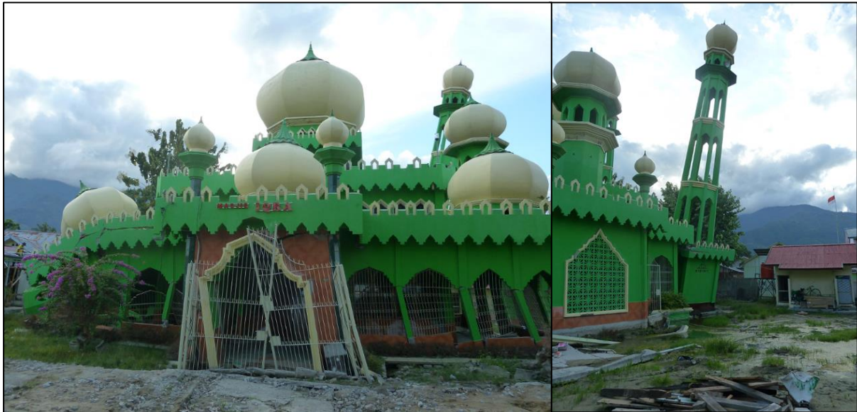
Figure 5.6 – Left: Front of Masjid Iqra. Right: Masjid Iqra in Lasoso. Severe liquefaction-induced damage and tilting of minaret due to liquefaction beneath base.
