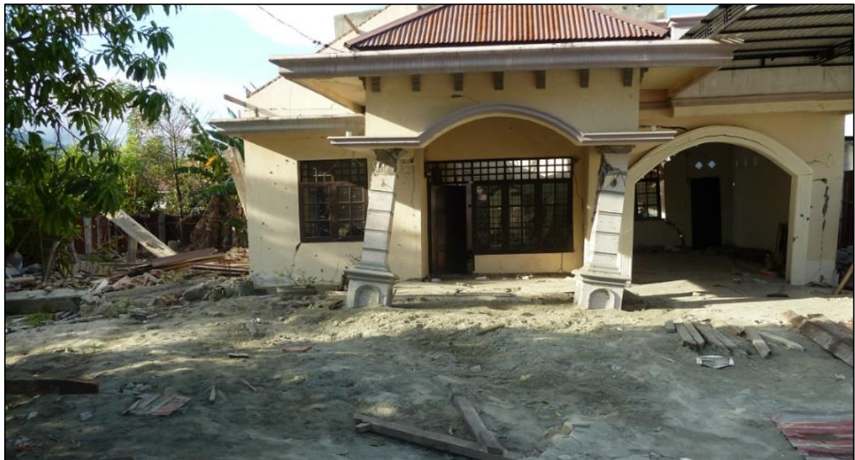
Figure 5.5. - Damage to a one-storey building in Lasoso due to differential settlement induced by liquefaction. Sandy ejecta in garden.
