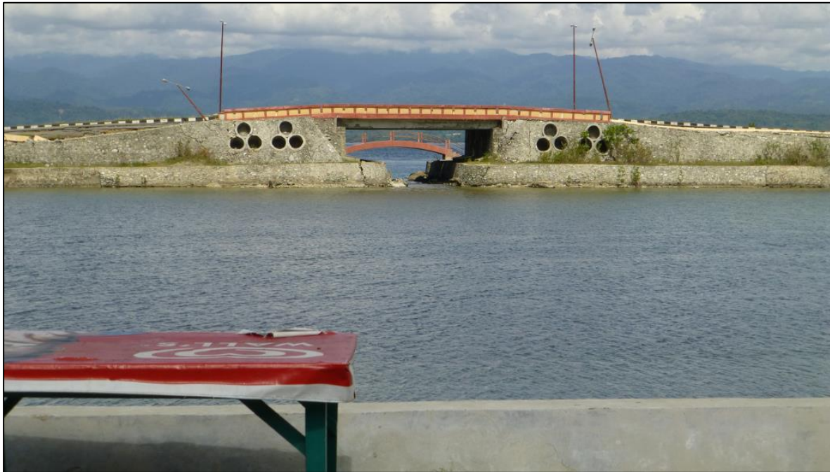
Figure 5.16 - View across dolphin enclosure to sea road. Slight damage to bridge abutments consistent with soil displacements, though bridge remains operational.
