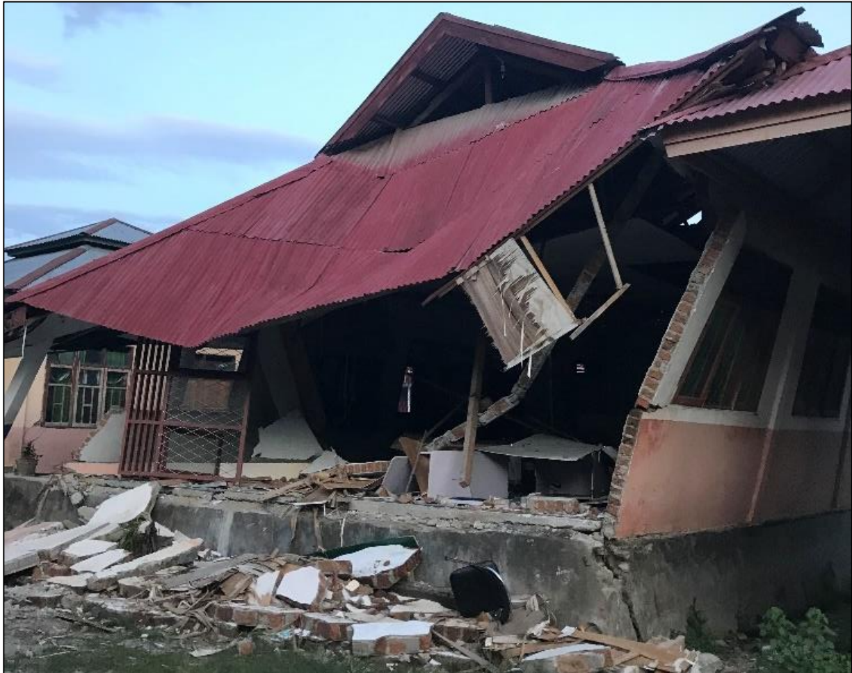
Figure 7.25 - Collapse of a CM school building in SMP Negeri 1 Biromaru School, Sigi.
