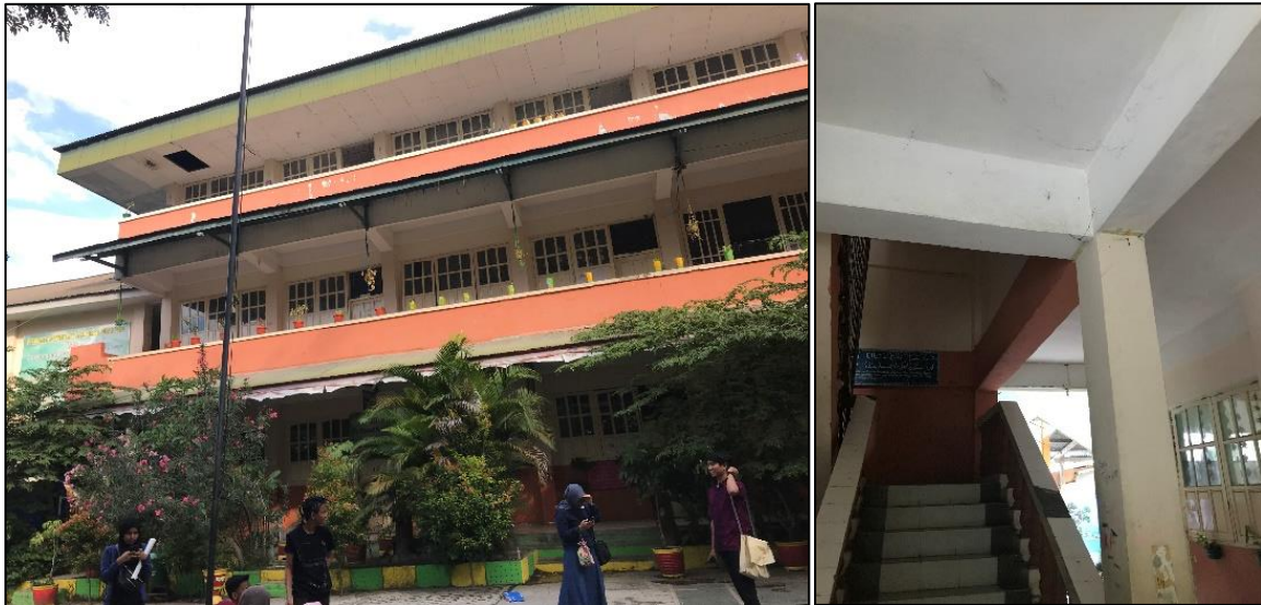
Figure 7.32 - MTS Alkhairaat Pusa Palu School. Left – 3-storey RC frame building that sustained minor damage to infill panels. Right – Typical sizes of beams and columns in RC frame schools.
