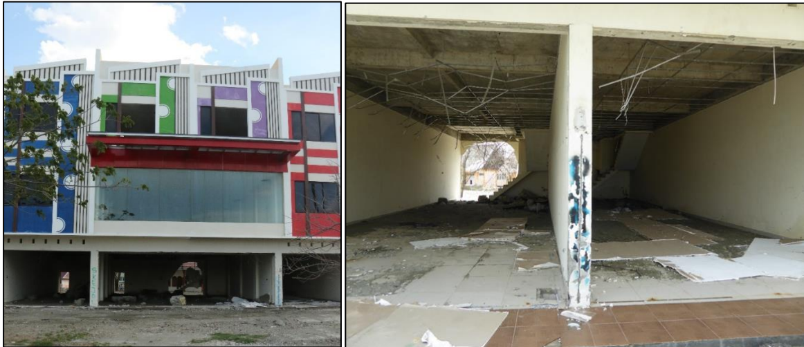
Figure 7.44 – Three –storey RC building near the Grand Duta Hotel. This structure was inundated by the tsunami at its ground floor, but sustained no structural damage, just non-structural damage to sea front windows and to back walls and to fittings at ground-floor level.
