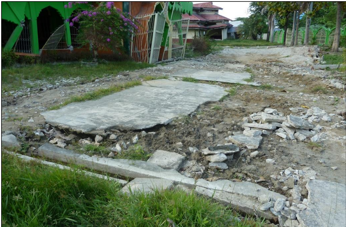
Figure 5.7 -. Masjid Iqra. Failure of garden paving above sandy soil, and ejecta in background.
