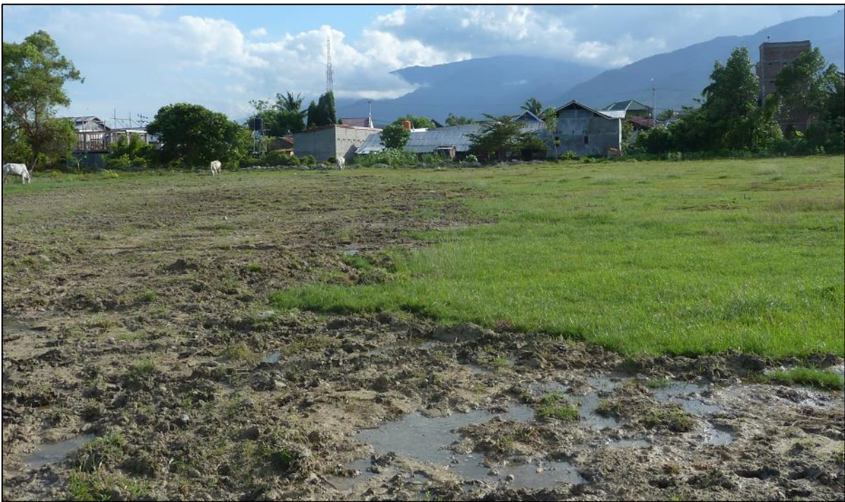
Figure 5.3.- Liquefaction ejecta in a field at Gelanggang Mahasiswa, Kabonena. The ejecta, is seen to follow the path of the fault across the field, although the soil on both sides appears to have settled by a similar distance.
