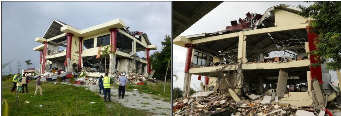
Figure 7.20 - Tadulako Univerity collapsed 3-storey building of the Faculty of Social and Political Sciences. Left – front view. Right – back view.
