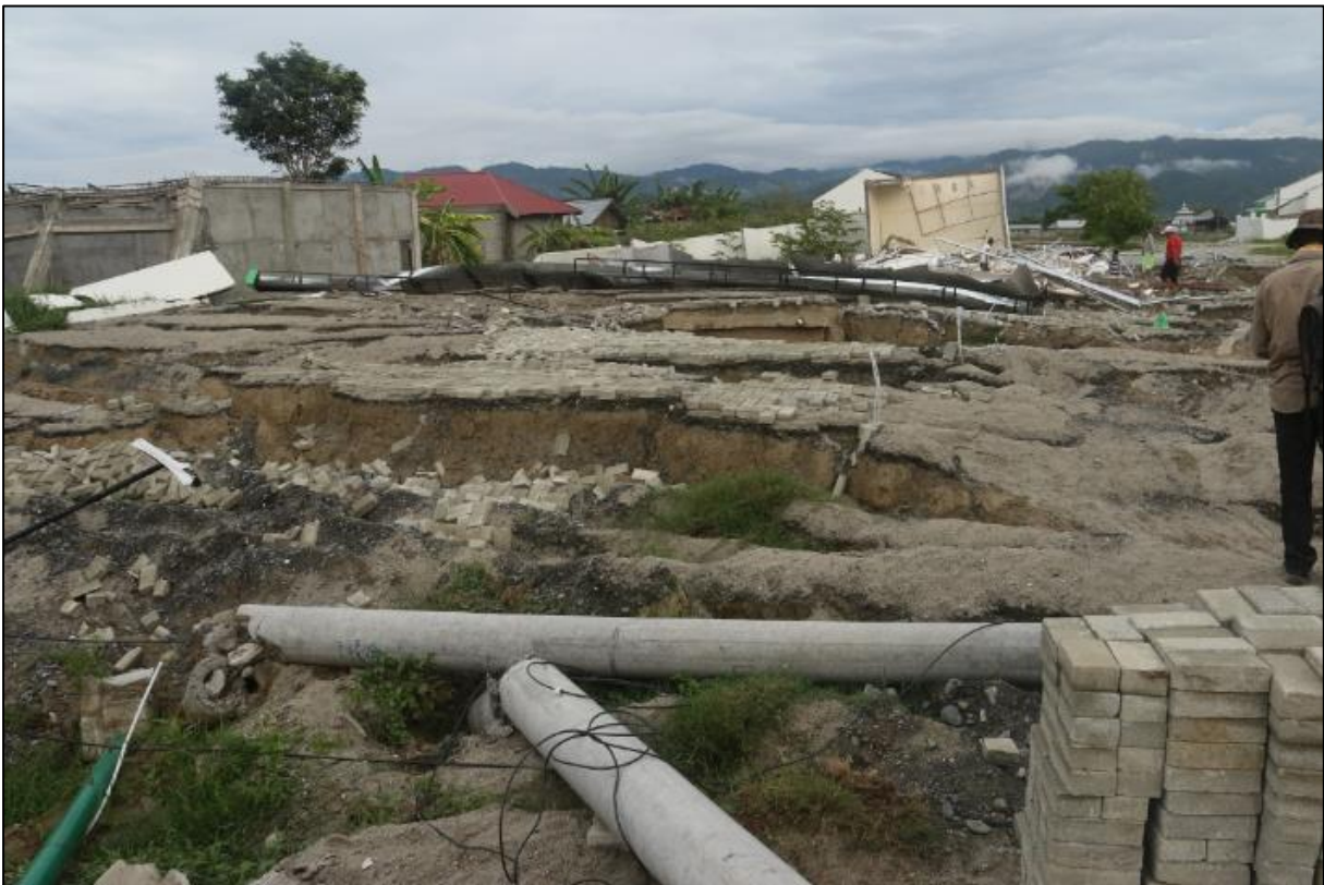
Figure 5.12 - Differential settlement and ground disturbance in Sigi. Pipework in foreground appears to be new rather than uplifted.
