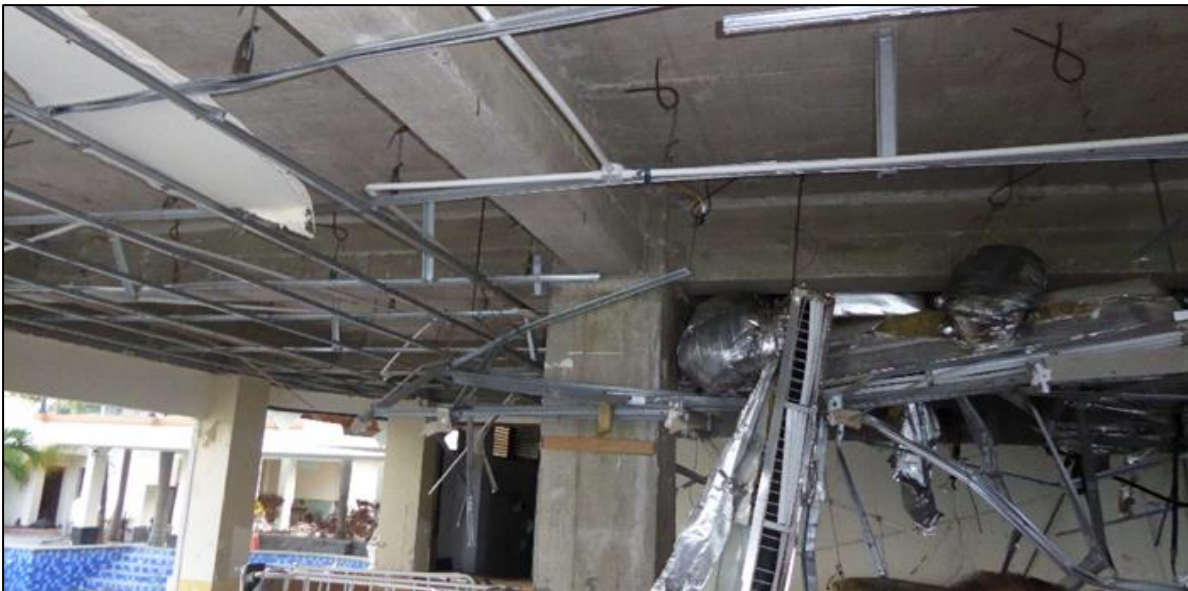
Figure 7.49 - Swiss Belhotel - damage to internal fittings at the ground storey of the shoreward side of the hotel. No structural damage observed in the main RC structure.
