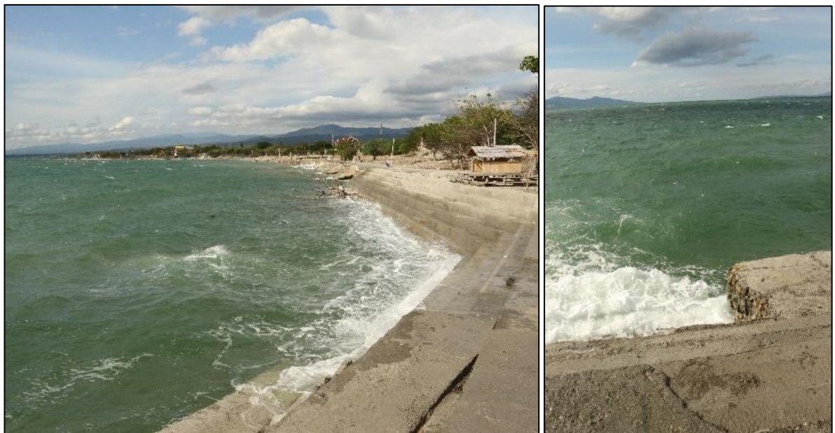
Figure 7.56 - Stepped revetment South of Mamboro missing its crest.
