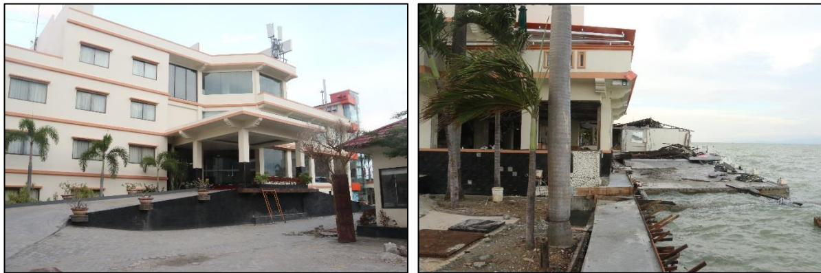
Figure 7.48 - Swiss Belhotel (Left) Undamaged front facade facing away from the bay (Right) Loss of confined masonry one-storey buildings to the shoreward side of the hotel
