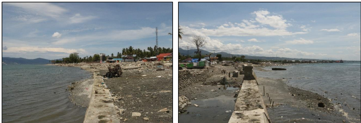
Figure 7.55 - Mamboro seawall showing loss of the crest of the structure
