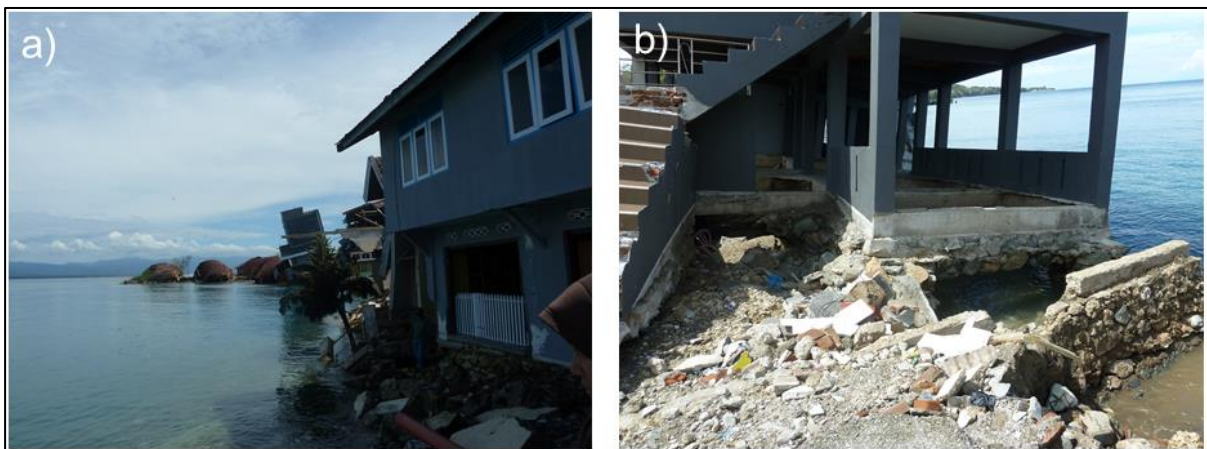
Figure 5.23.- Photographs of Donggala Port, looking a) South East across the estuary towards the partially collapsed metal rooved storage houses b) detail beneath the concrete structure seen tilted on the South edge of the bay, showing evidence of soil having been displaced from beneath the structure.
