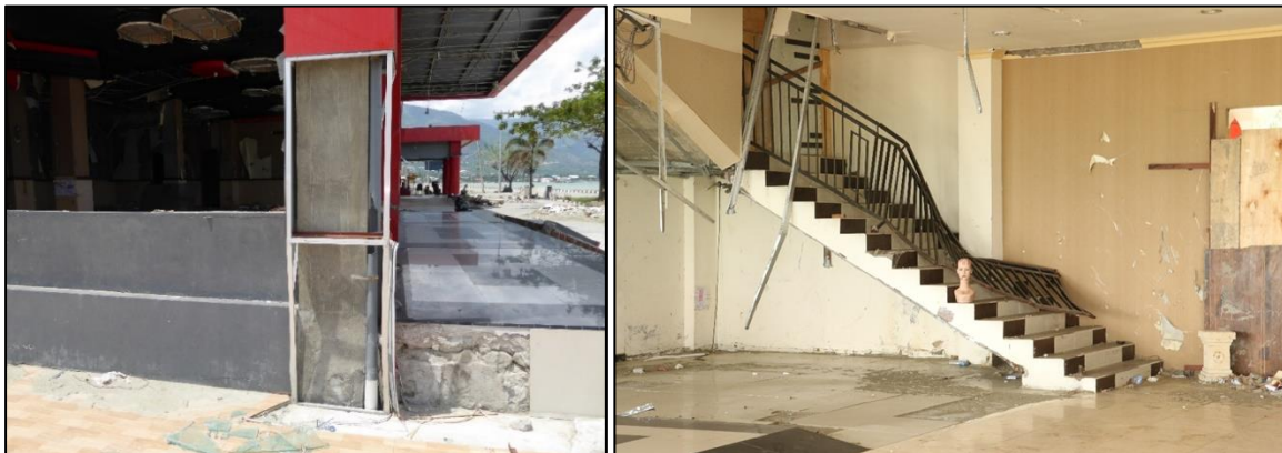
Figure 7.43 – Grand Duta Hotel, Left – image of intact column at ground floor. Right – Image of staircase inside the ground floor of the hotel. The staircase railing was damaged when it was hit by a large desk moved by the tsunami inundation.
