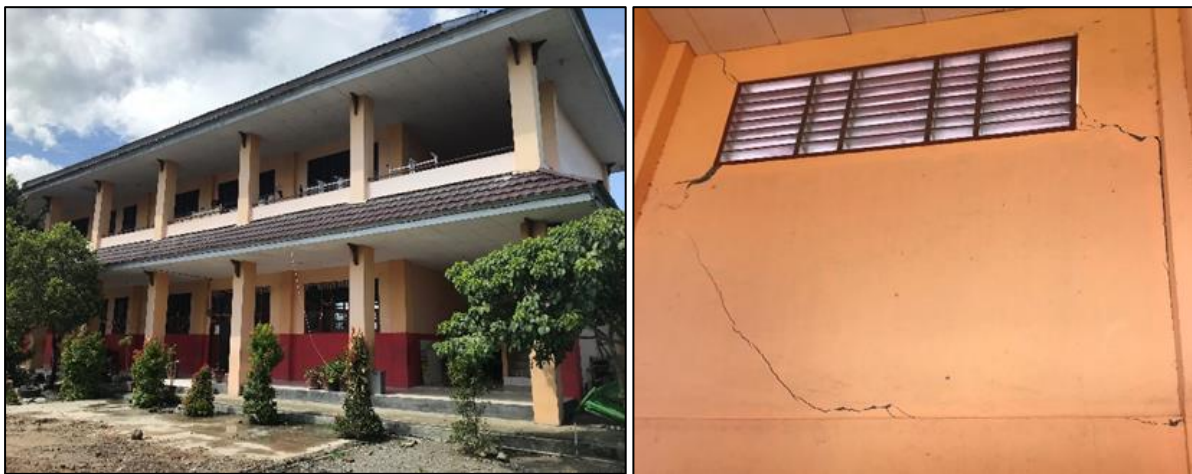
Figure 7.33 - SD Negeri Pengawu School in Palu (Building A in Fig. 7.24c). Left – 2-storey RC school building that sustained moderate damage to infill panels. Right – Damage to the infill walls
