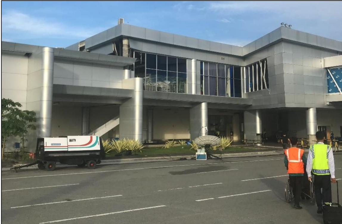
Figure 7.50 - View of Palu Airport passenger building from the runway. Damage to the infill walls at the ground floor is observed. A stack of fallen ceiling cladding can be seen in upper storey window.
