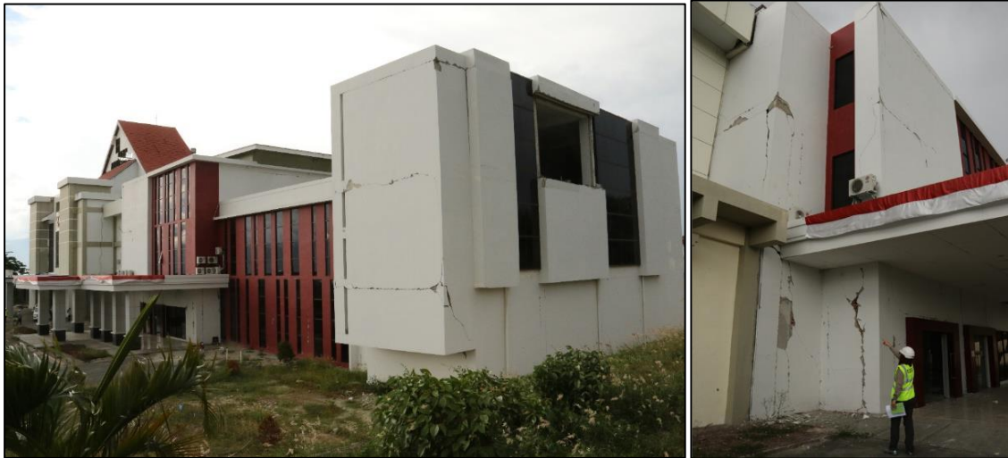
Figure 7.38 - Tadulako University Hospital Building B. Left – Side view of Building B, showing out of plane failure of infill wall at second floor (n.b. plane of infill wall is E-W). Right – location of damage due to pounding between Buildings A and B.
