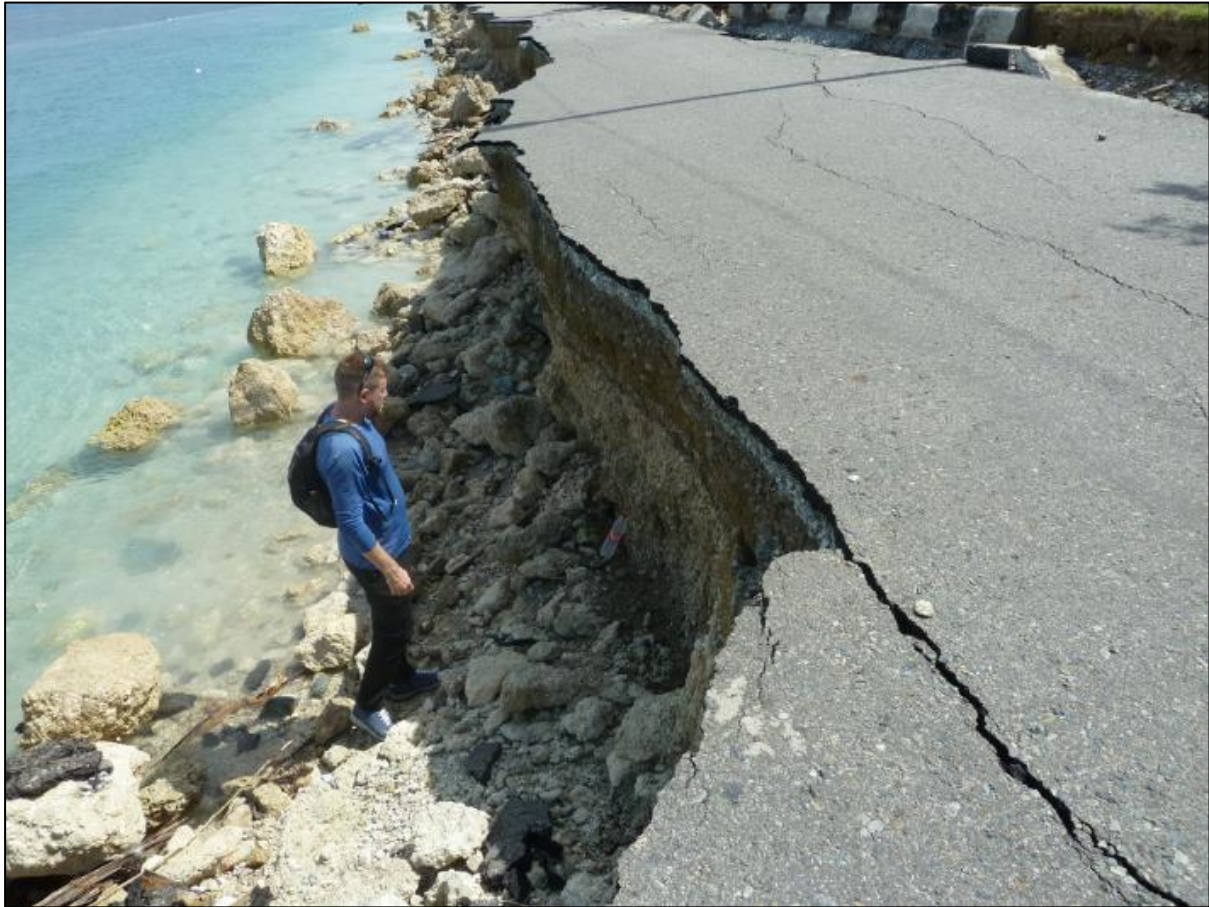
Figure 5.19.- Soil layers exposed by lateral spreading at Donggala Koto Wisata.
