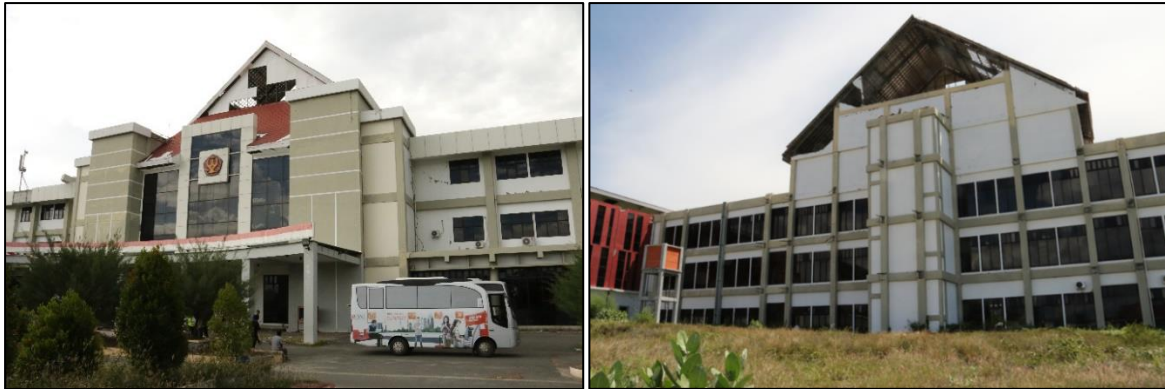
Figure 7.36 - Tadulako University Hospital Building A. Left – Front view. Right – rear view, showing damage to gable.
