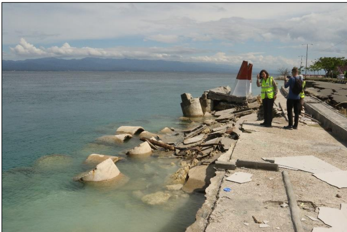
Figure 7.58 - Collapse of quay wall at ‘Dolphin Park’ at Donggala Koto Wisata.
