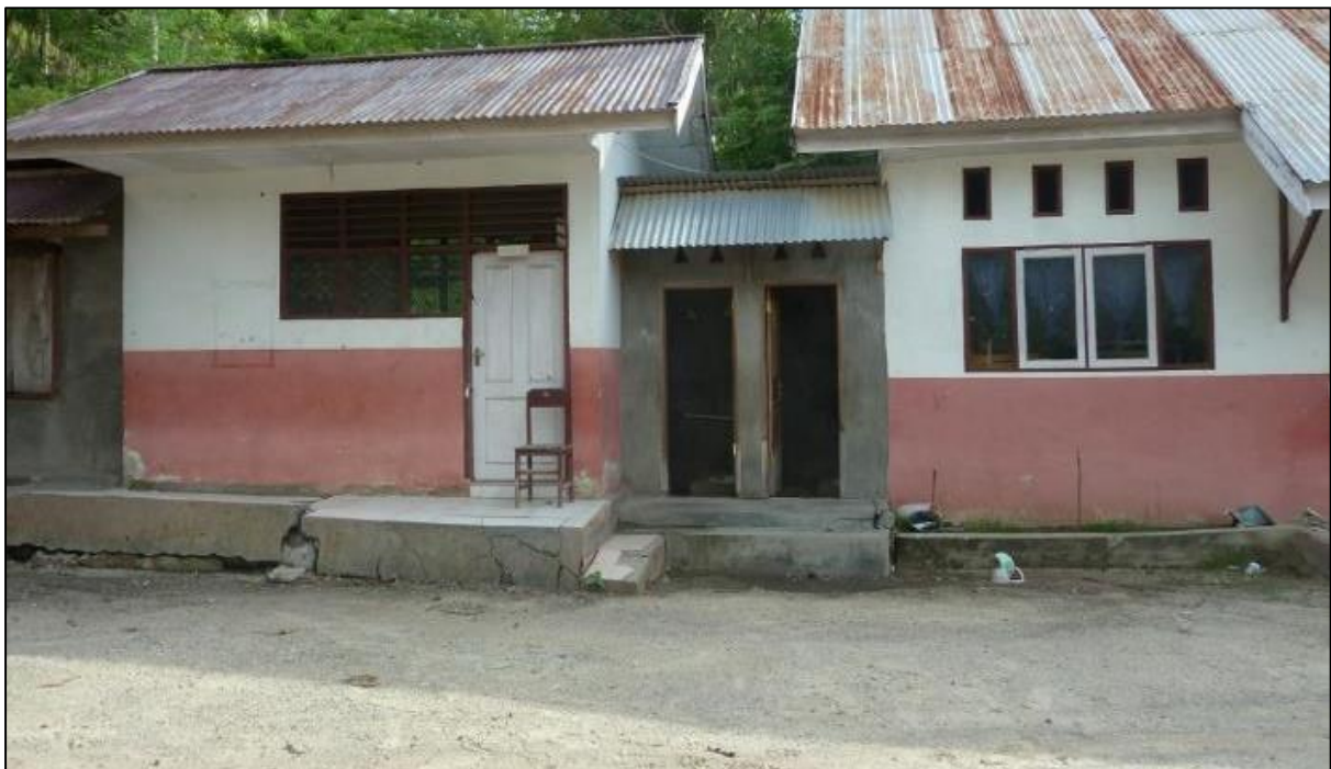
Figure 5.25 – Differential settlement of School in Lero, with liquefaction ejecta in the yard
