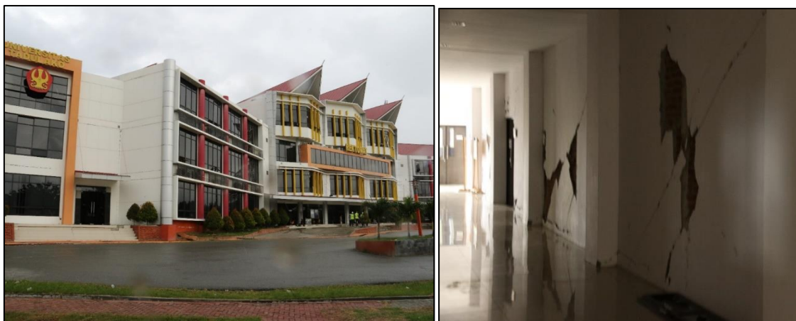
Figure 7.19 - Tadulako University Rektorat (DET2): exterior view (left); damage to internal infill panels (right)
