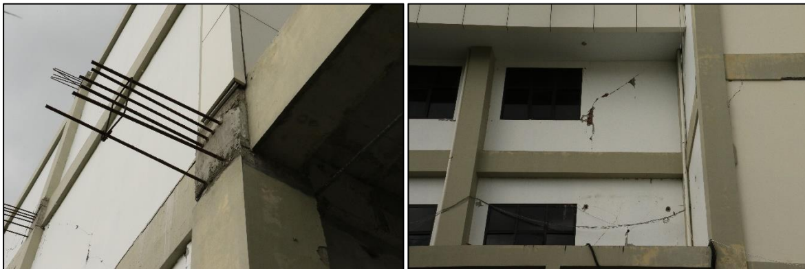
Figure 7.37 - Tadulako University Hospital Building A. Left – Beam reinforcement detailing. Right – damage to brick masonry infills.
