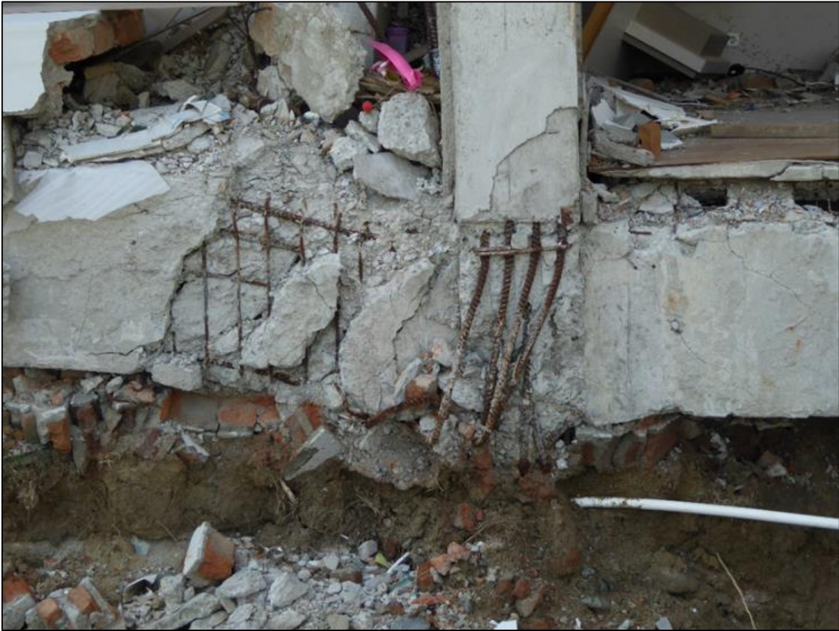
Figure 7.47 – Mercure Hotel – Detail of a joint within the first floor of the building (now at ground level following soft-storey collapse of ground floor).
