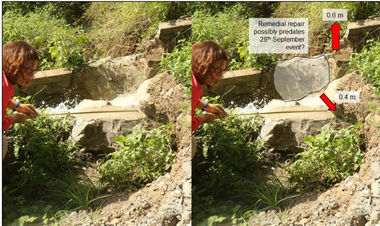
Figure 3.8 – Damage to water channel on North side of large rupture at Labua indicates observed total displacement may be only partly due to 28 th September event
