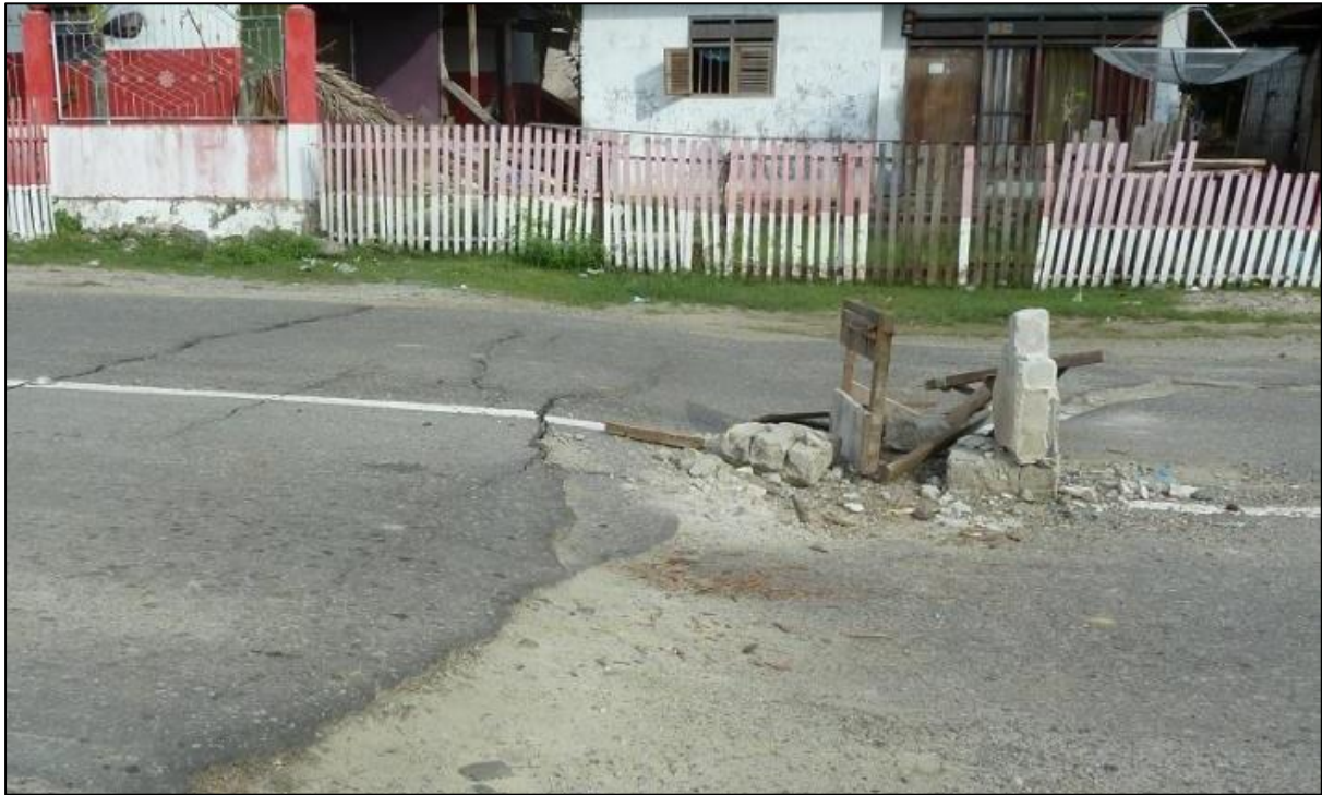
Figure 5.24 – Settlement in the road with sandy soil ejected through cracks.
