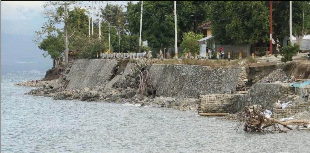
Figure 7.57 - Damaged masonry seawall just to the south of Tasiburi
