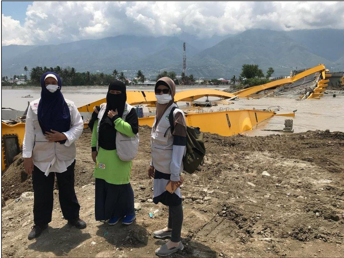
Figure 7.53 - Picture of Ponulele bridge showing the failed deck. Source: Tripadvisor.
