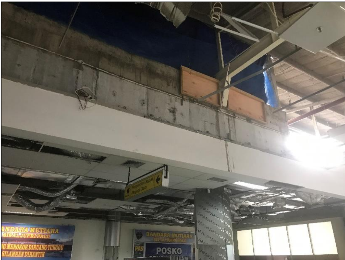
Figure 7.51 - Picture of missing ceiling cladding and damaged fixtures, inside Palu Airport passenger building.
