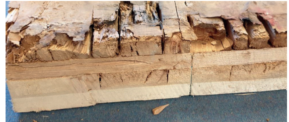
↑ Figure 1 Rotting of CLT panel
