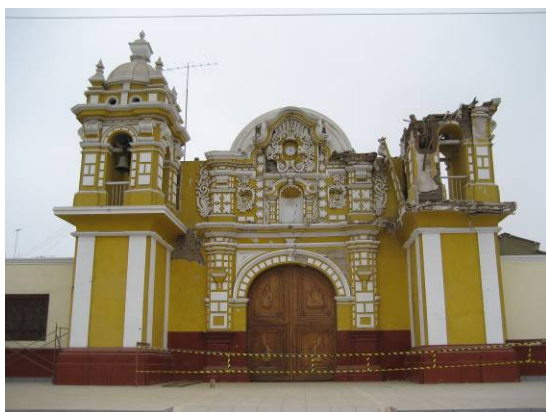
Figure 12.9 XVII century chapel in Hacienda San José near El Carmen with damaged bell tower.
