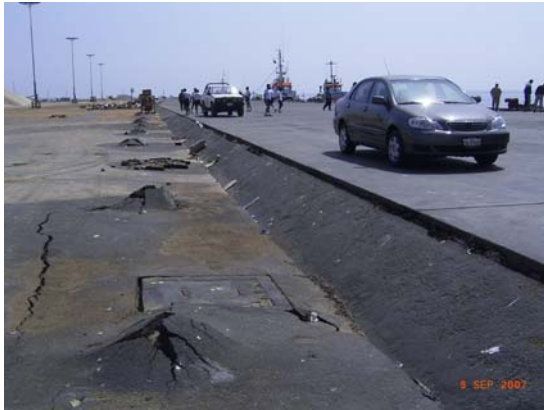
Figure 7.7 Port of San Martín: pile caps punching through the paved access (looking north)
