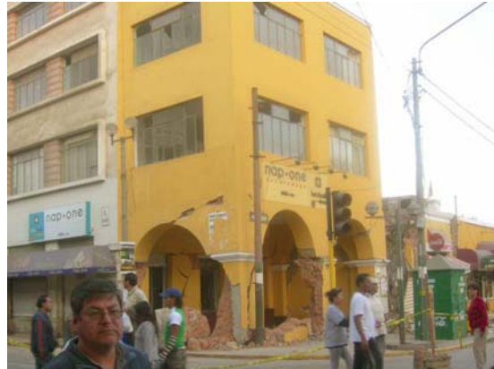
Figure 5.15 Severely damaged masonry structure in Plaza de Armas, Ica, at corner next to a RC building (Photo: Dr. Ing. Jorge E. Alva Hurtado, Universidad Nacional de Ingeniería, Peru )
