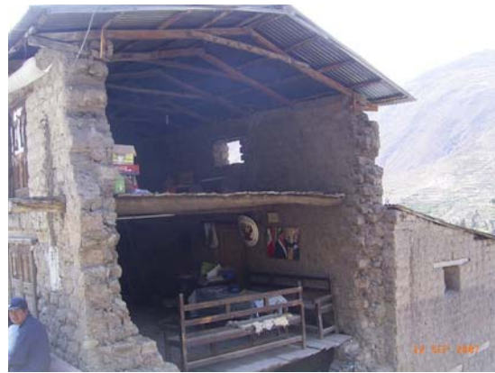
Figure 5.9 Two storey adobe house damaged in Huangáscar
