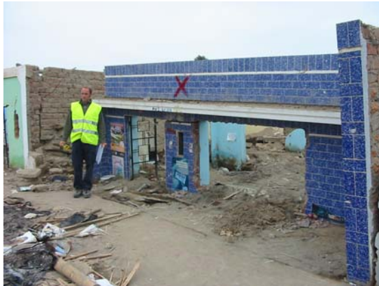
Figure 3.3 Large settlements reached values of approximately 1.0 metre
