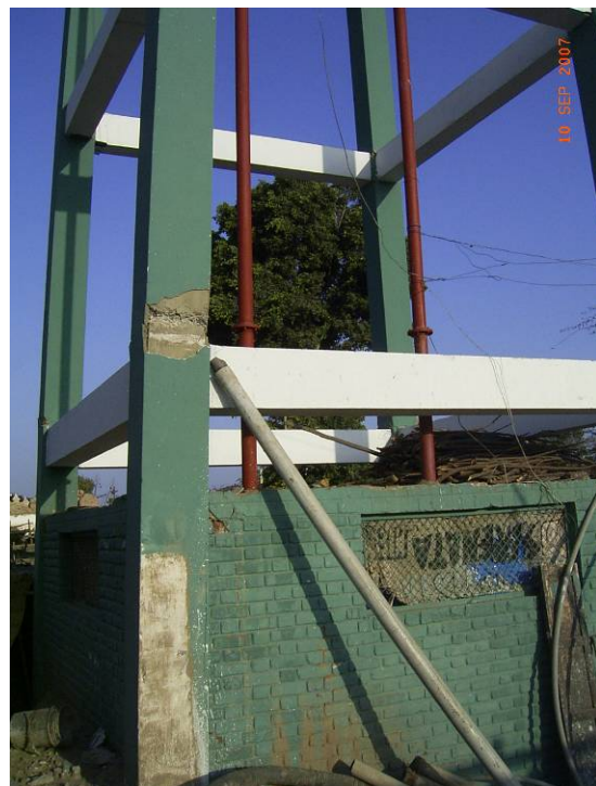
Figure 8.4 Damaged column next to infill wall, joint showing insufficient reinforcement.
