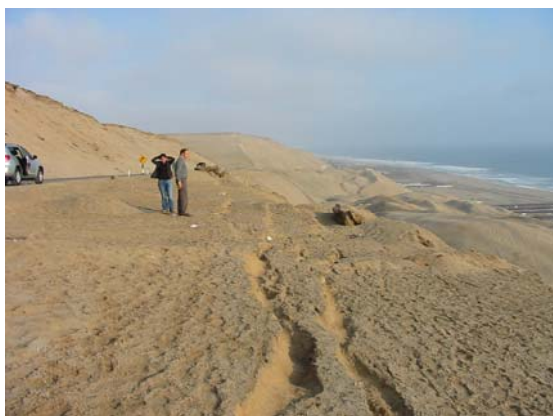
Figure 3.8 Scarp of landslide on the Pan-American Highway; two tension cracks are observed at the bottom of the picture
