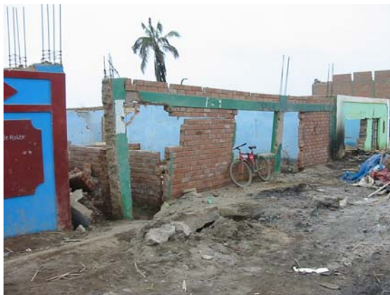
Figure 3.5 Large settlements reached values of approximately 1.0 metre
