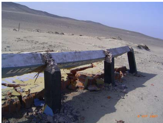
Figure 5.35 Overall view of the collapsed billboard at Pozo Santo, showing four 250x250 mm 1.05 m RC columns
