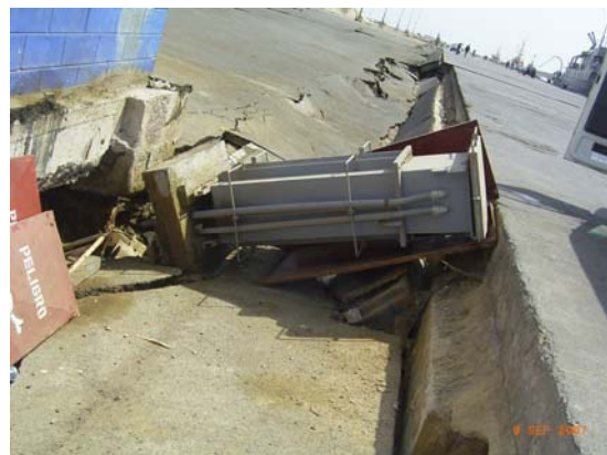
Figure 7.6 Port of San Martín: toppled electric transformer
