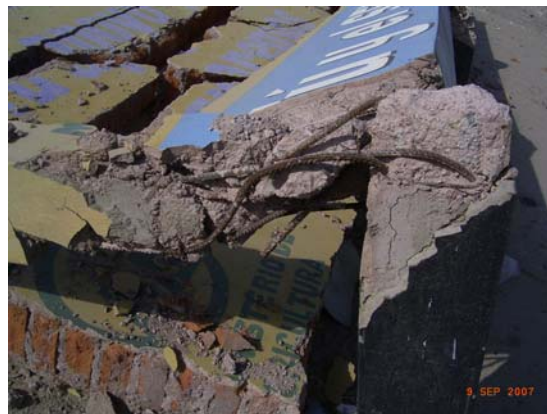
Figure 5.36 Detail of the RC columns of the Pozo Santo billboard, showing 12 mm diameter steel rebars with practically no confinement
