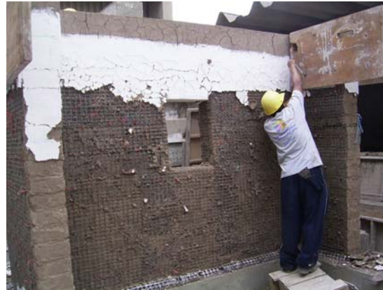
Figure 5.20 Reinforcement of adobe walls with nylon net at the laboratory of PUCP
