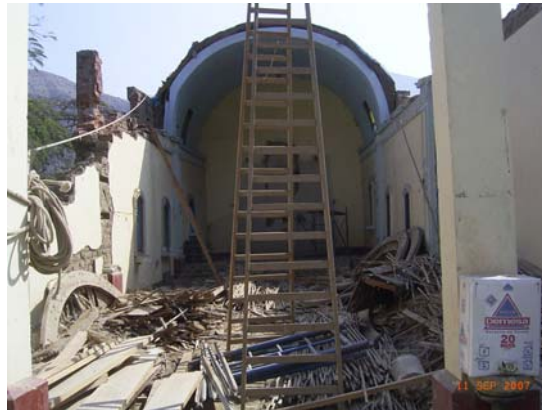
Figure 5.39 Typical collapse of a quincha vaulted roof of a church in Zúñiga
