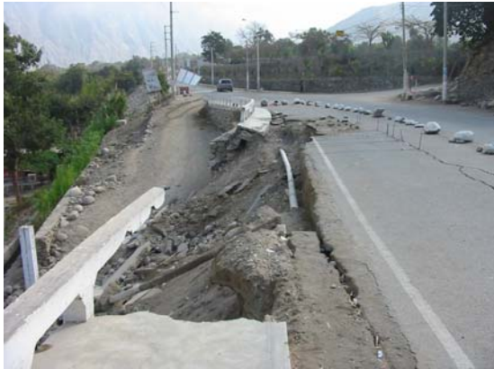
Figure 3.10 Stone retaining wall failure close to Lunahuaná
