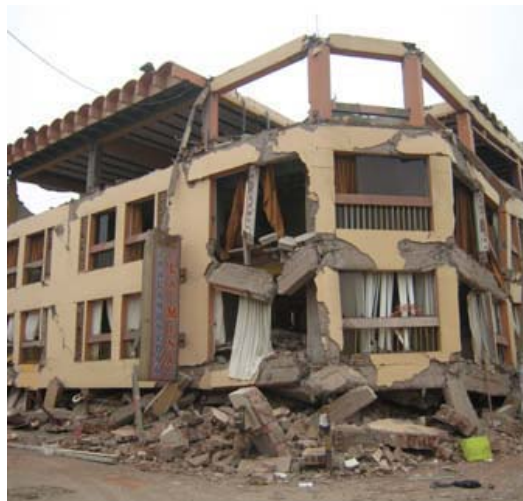
Figure 5.26 Collapsed Embassy Hotel in Pisco (Photo Prof. M. Blondet, PUCP, www.eeri.org/lfe/images/peru_coast_photos )
