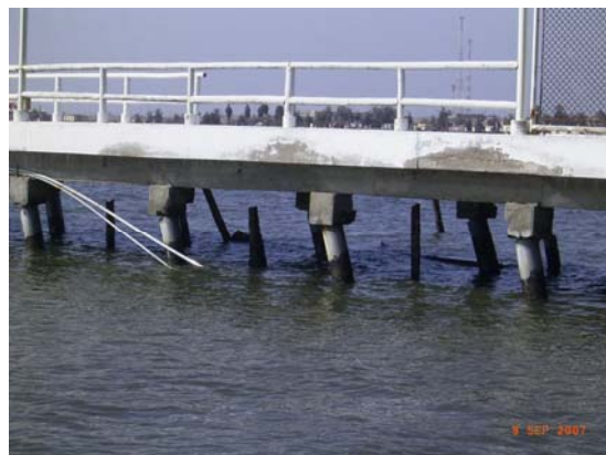
Figure 7.12 Jetty structure at Yacht Club in Paracas: top hinging of steel piles
