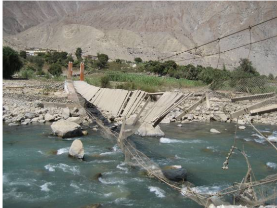
Figure 6.10 Pedestrian bridge crossing the Cañete river damaged by rock fall.
