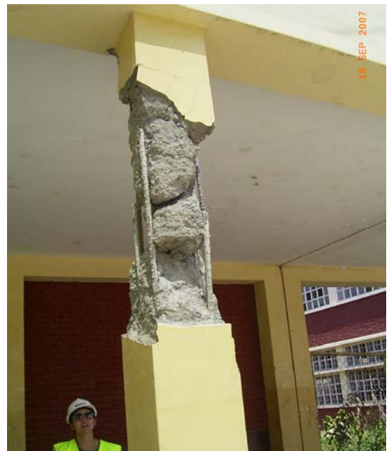
Figure 10.8 Gran Unidad Escolar San Luis Gonzaga : column failure in shear due to insufficient shear reinforcement and low quality of concrete
