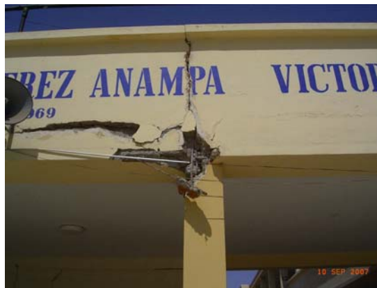
Figure 10.4 Gran Unidad Escolar San Luís Gonzaga : column failure at top end; roof parapet activated a strong-beam-weak-column mechanism
