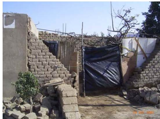
Figure 5.18 Collapsed right corner of the adobe house shown in Figure 5.17 (not upgraded due to insufficient funds)
