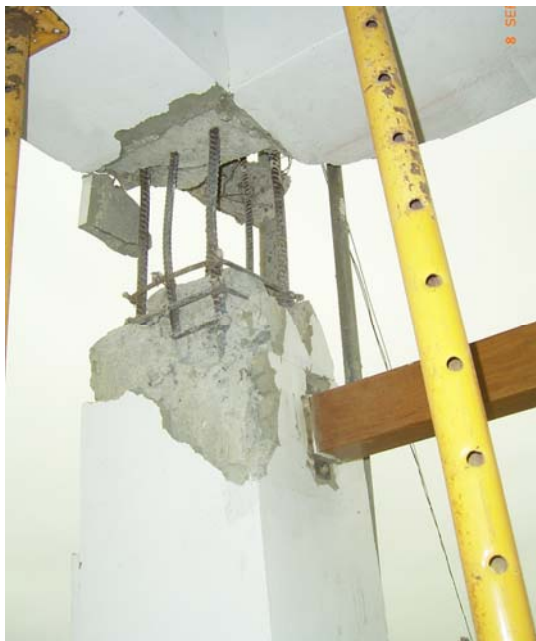
Figure 10.7 Pisco: School building showing failure of column at top end at the second storey, due to insufficient shear reinforcement and activation of a strong-beam-weak-column mechanism
