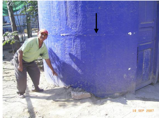
Figure 8.2 Flexural crack running around the perimeter at the base.
