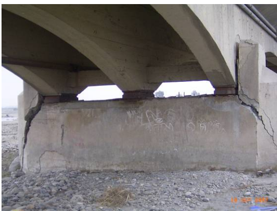
Figure 6.8 Huamaní Bridge: damage of parapets at the second northernmost pier.
