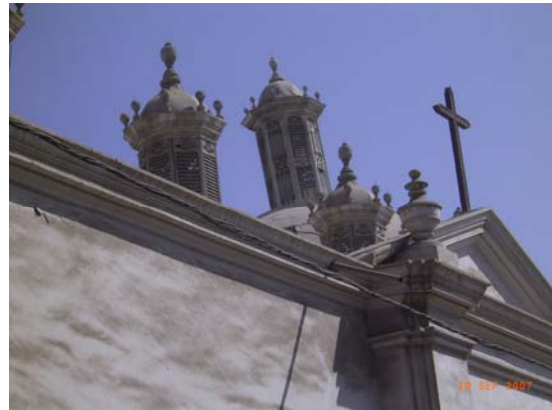
Figure 5.41 Tilted bell towers of a church next to Plaza de Armas in Ica
