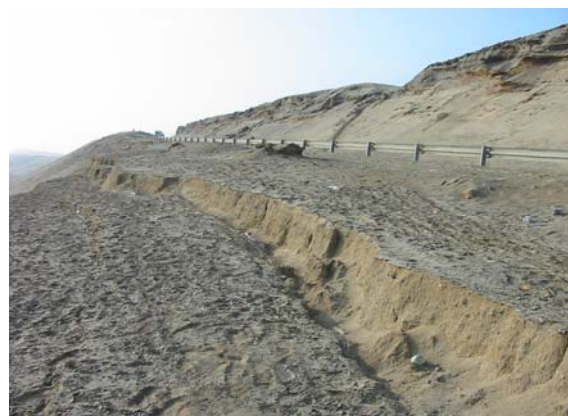
Figure 3.9 Detail of landslide scarp; the largest vertical displacement was measured at 0.4 m
