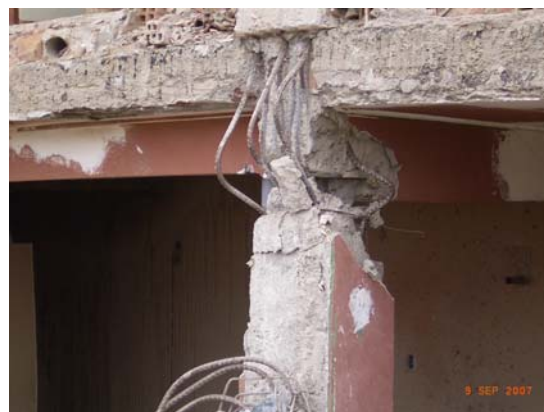
Figure 5.28 Detail of column failure in shear of the building structure of Figure 5.27
