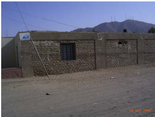
Figure 5.17 Adobe house in Guadalupe upgraded with steel net reinforcement plastered to the exterior and interior surface and showing good performance
