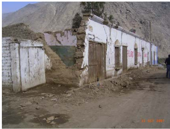
Figure 5.8 Sturdier walls up the Cañete river valley in Zúñiga close to collapse
