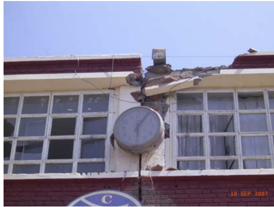
Figure 10.10 Gran Unidad Escolar San Luis Gonzaga : damage due to pounding at ceiling level
