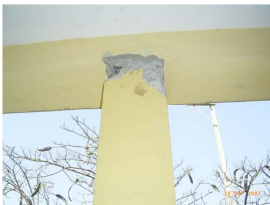
Figure 10.3 Gran Unidad Escolar San Luís Gonzaga : column failure at top end
