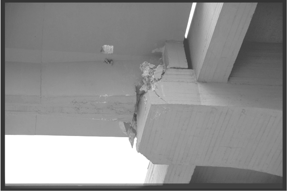
Figure 7.15: Detail of footbridge shear key damage – longitudinal displacement
