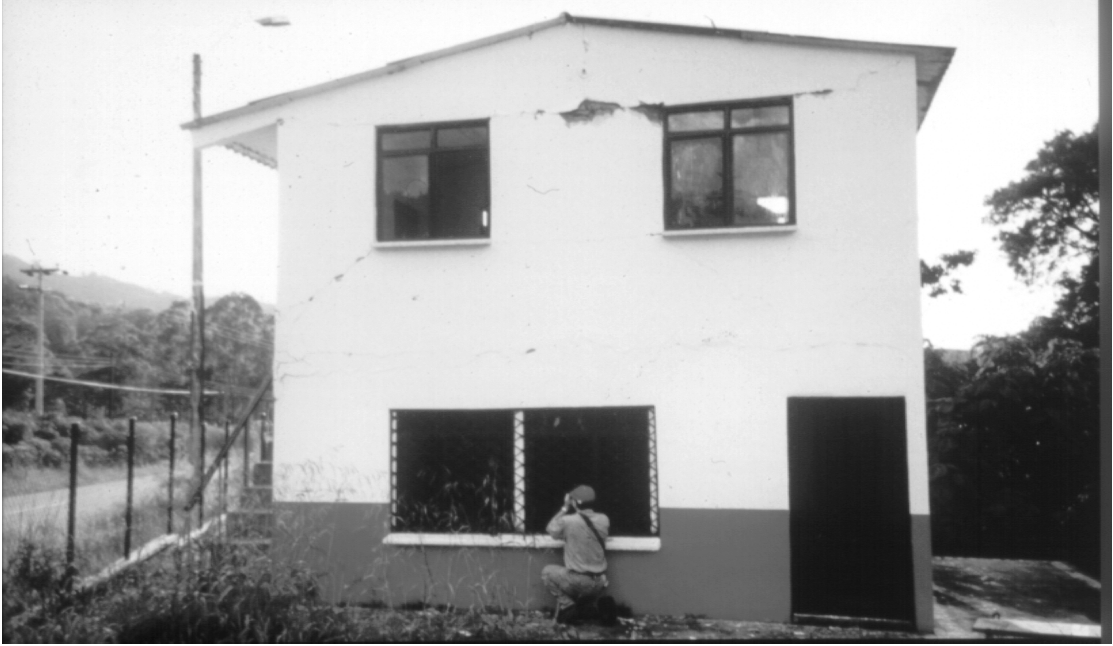
Figure 5.19: Damage to a masonry building at the bamboo centre
