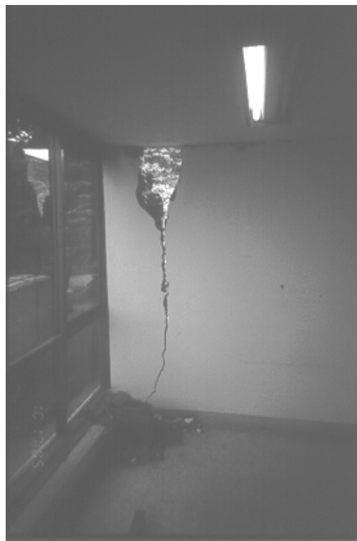
Figure 4.20: Cracking to external infill wall panel
