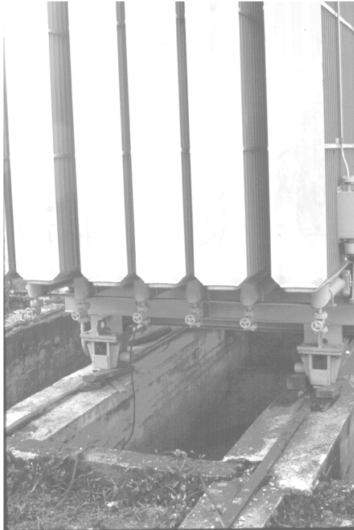
Figure 7.17: Replacement of damaged electric transformer of Regivit substation in Armenia, with damaged concrete wall shown on the lower right
