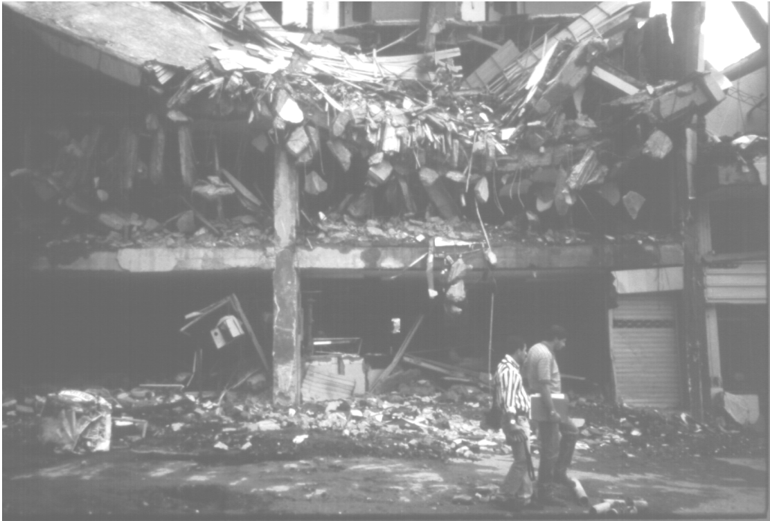
Figure 5.11: The fate of many concrete framed buildings
