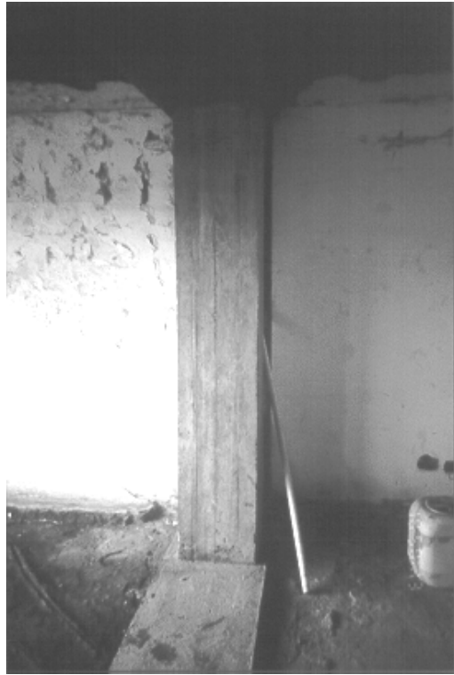
Figure 4.27: Retrofitted beam and column, with beam only providing additional restraint to column in one direction
