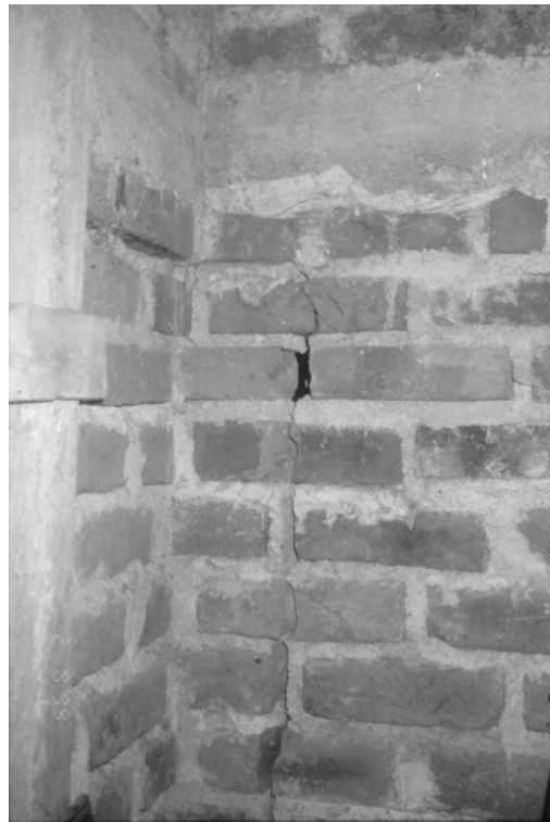
Figure 5.8: Ring beam at roof level, successful in halting the propagation of cracking in the corner of the masonry wall
