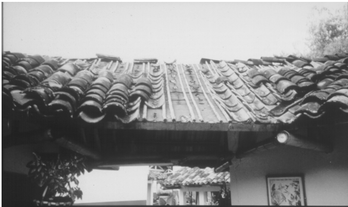
Figure 5.18: Displaced tiles from the roof of a house at the bamboo centre
