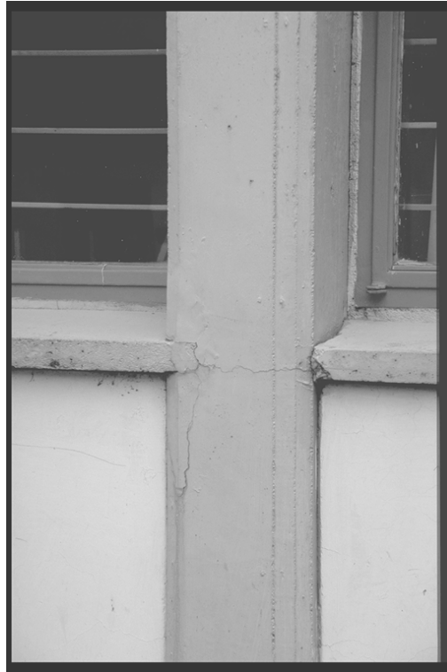
Figure 7.27: School in Pijao: Shear cracks in columns at top of infill
