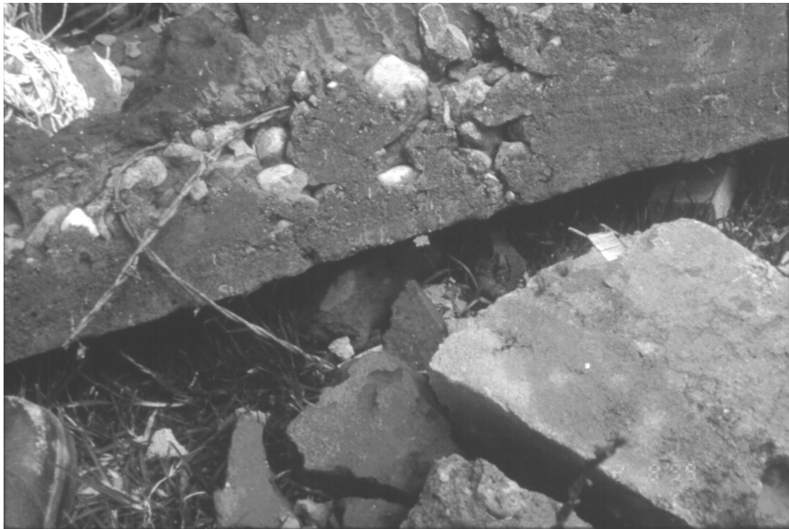
Figure 5.10: Example of poor quality control. Concrete lintel with barbed wire being used as the main tension reinforcement.
