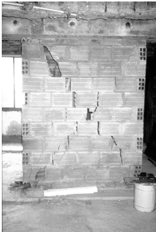
Figure 4.28: Shear cracking to internal non-loadbearing wall
