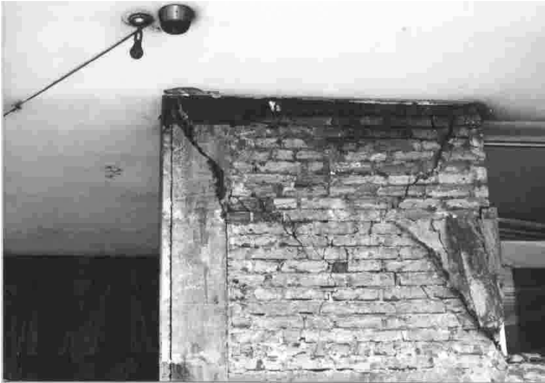
Figure 4.5: Shear failure of column
