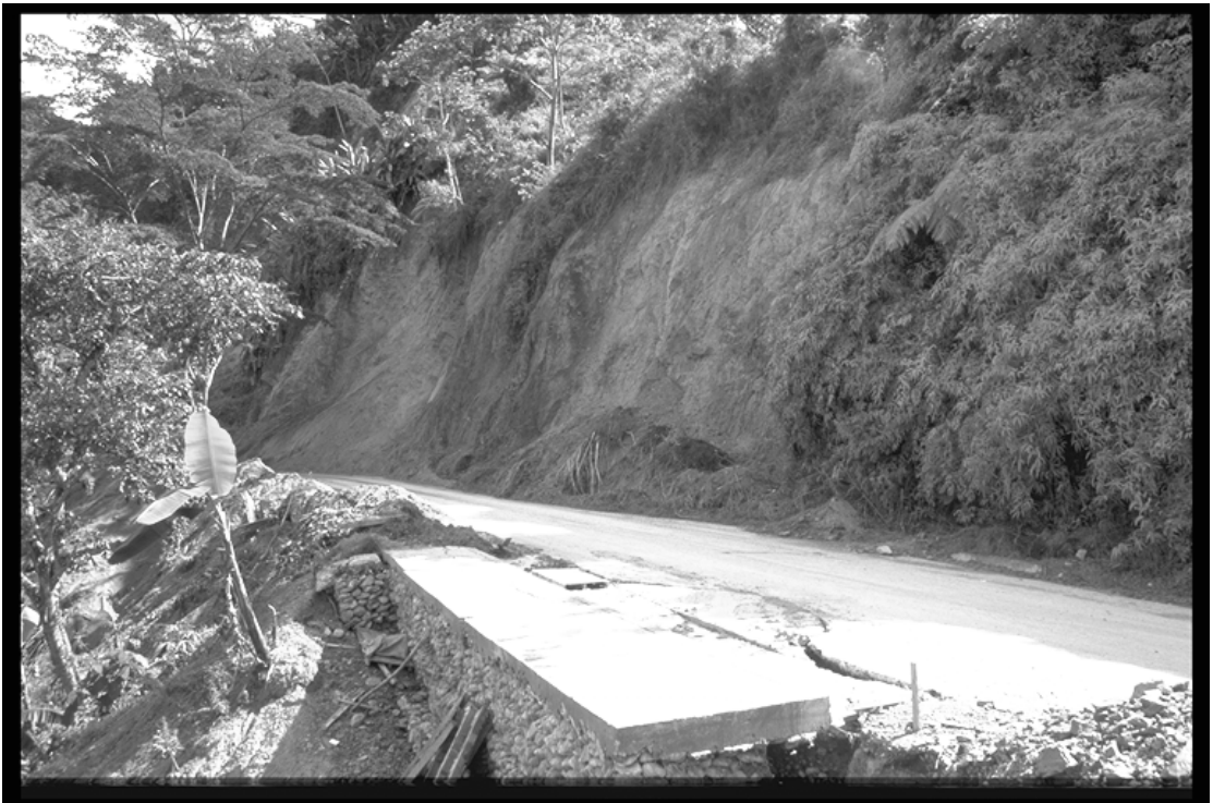
Figure 7.20: Partial failure of gabion retaining wall on the road to Pijao
