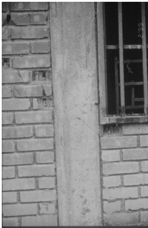
Figure 5.14: 'Short column' shear failure
