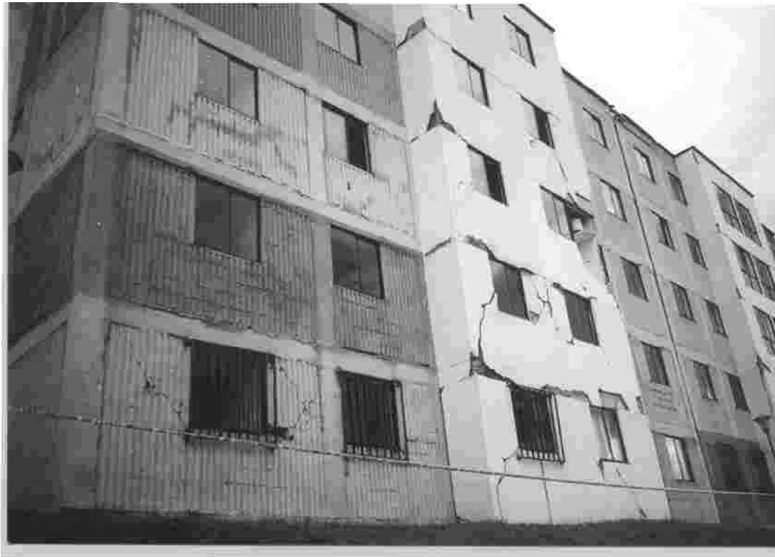
Figure 4.14: Non-structural damage of recent structure
