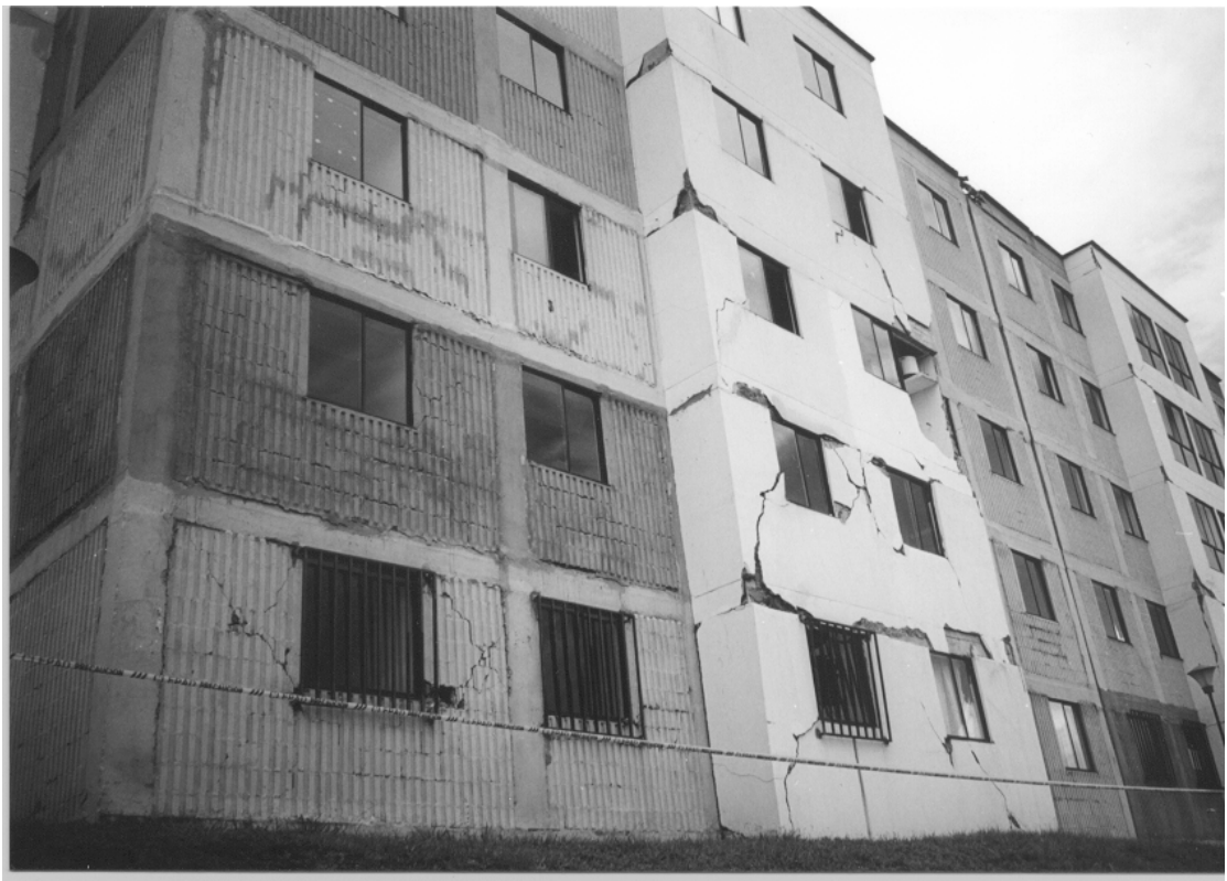
Figure 3.6: Non-structural damage – Pereira
