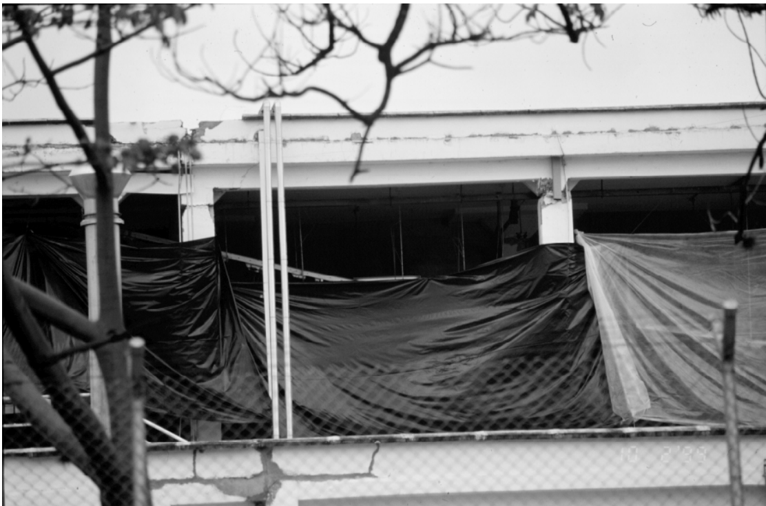
Figure 7.28: Failure of columns at the top of the second storey of a Dosquebradas industrial facility
