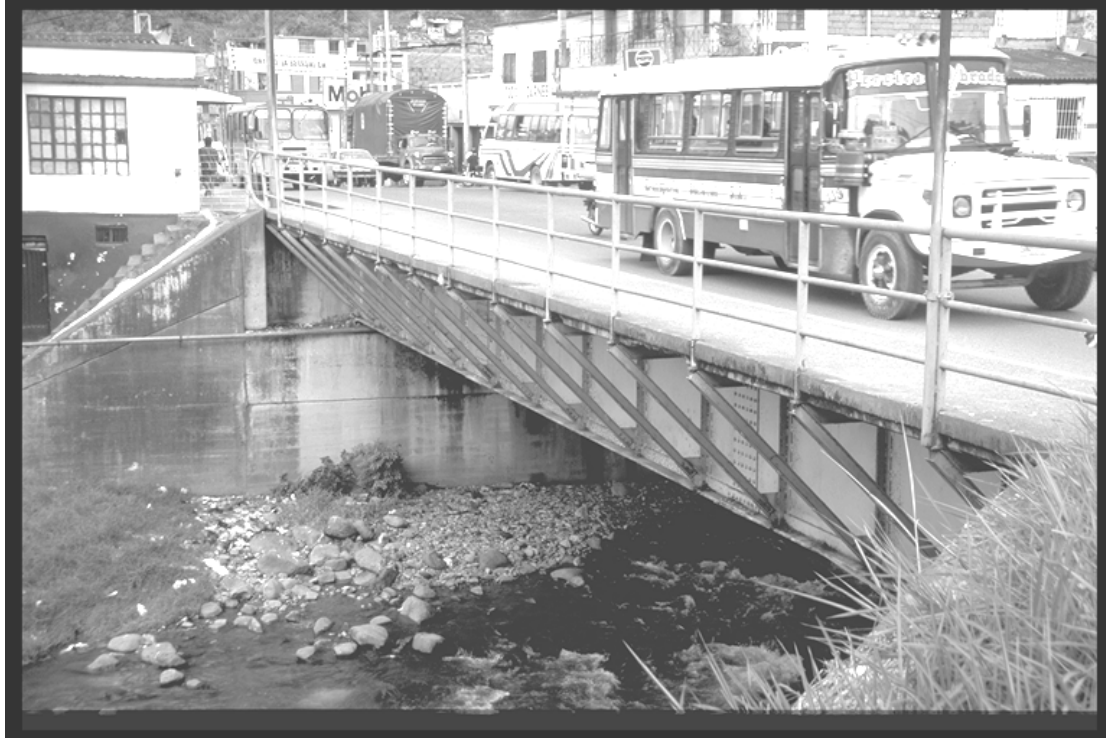
Figure 7.5: Single span steel plate girder bridge close to cable-stayed bridge in Pereira
