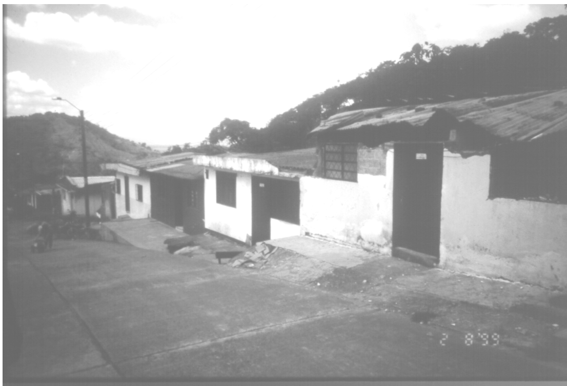
Figure 5.6: Single storey masonry buildings. Note section of wall missing in nearest building.
