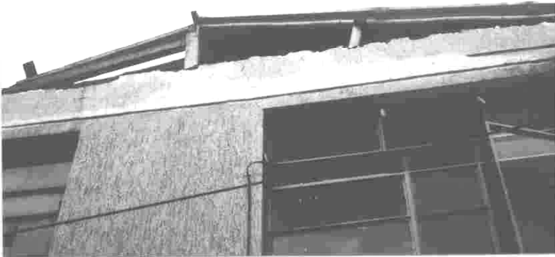
Figure 4.13: Collapse of free-standing masonry wall
