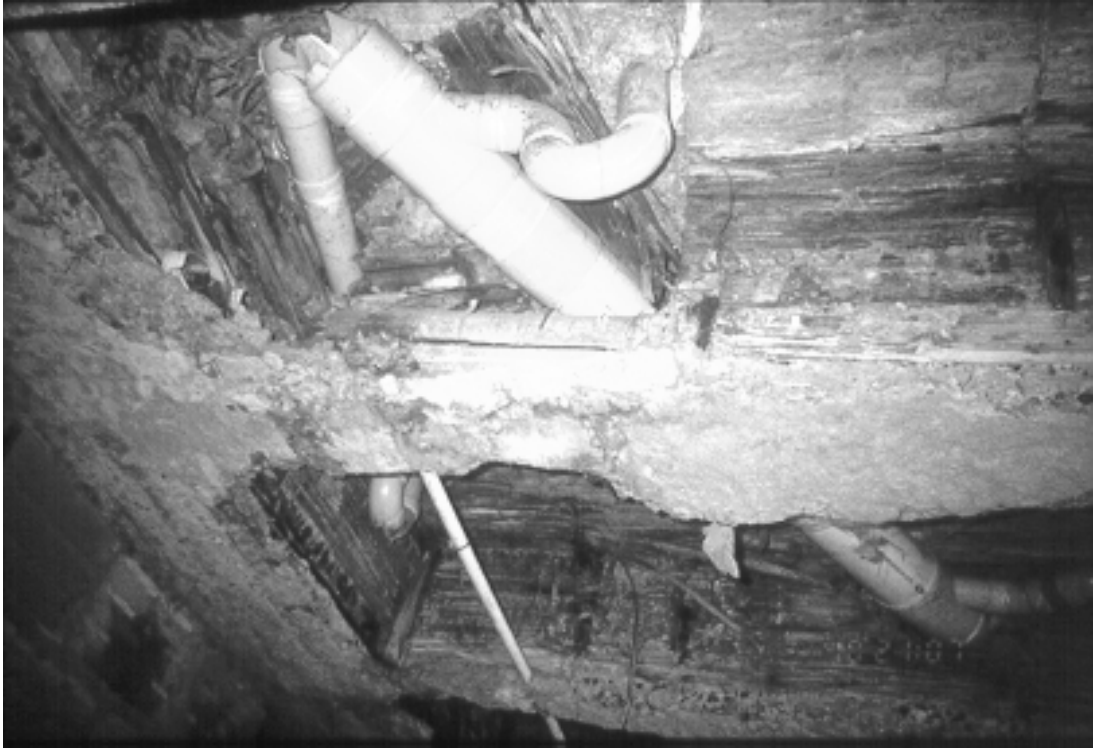
Figure 4.23: Concrete floor rib detail, showing poorly located service pipework
