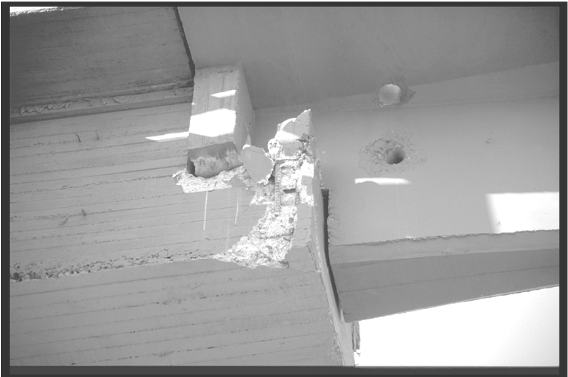
Figure 7.16: Detail of damage of similar footbridge – transverse displacement
