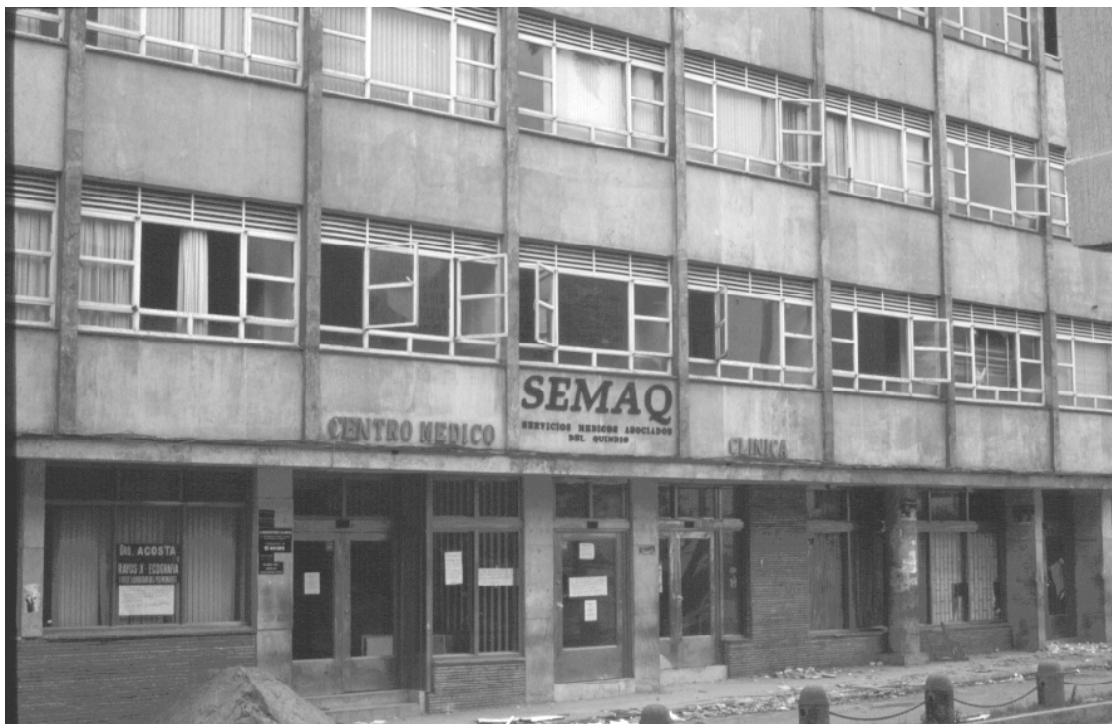
Figure 7.24: Hospital in Armenia city centre (pre-1984 design), closed due to non-structural damage after the earthquake
