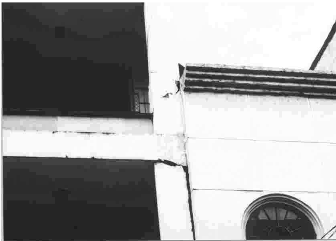
Figure 4.6: Shear failure of column
