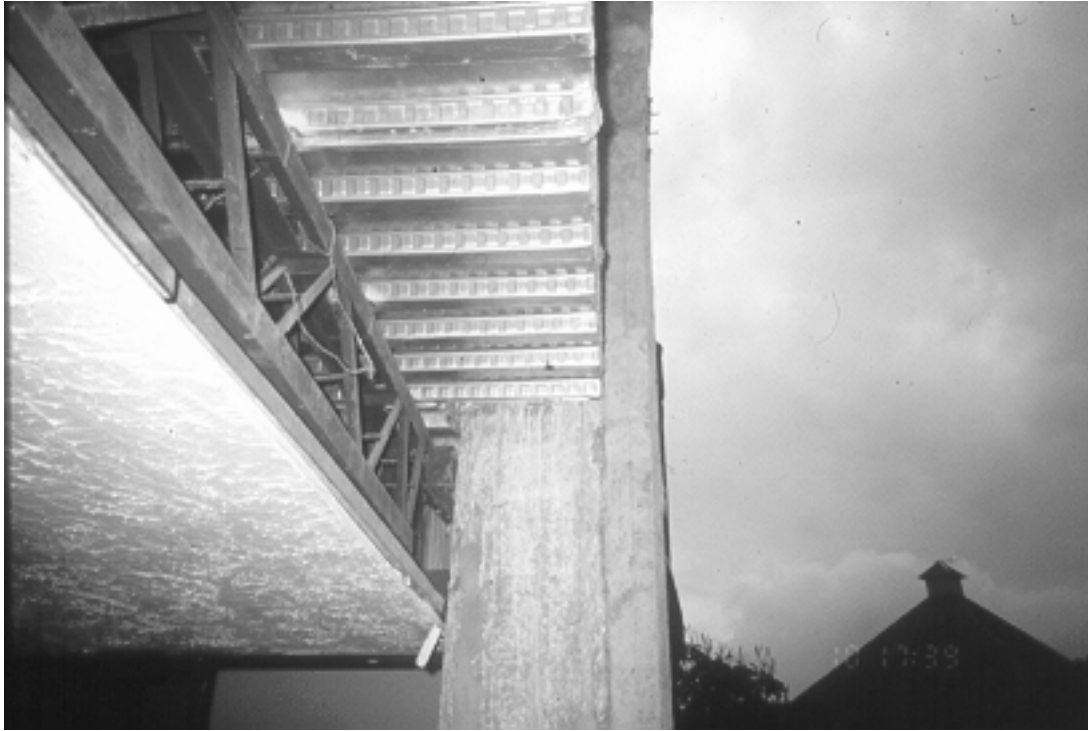
Figure 4.17: New steel truss floor beam with metal decking and RC slab over
