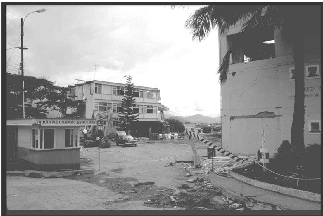
Figure 7.22: The police station in Armenia. The central block (centre of photo) had completely collapsed.
