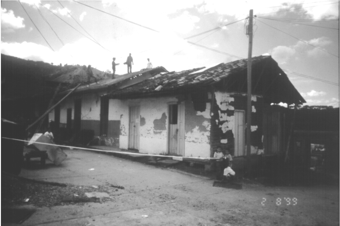
Figure 5.3: Separation of walls and roof of a bahareque construction in Córdoba
