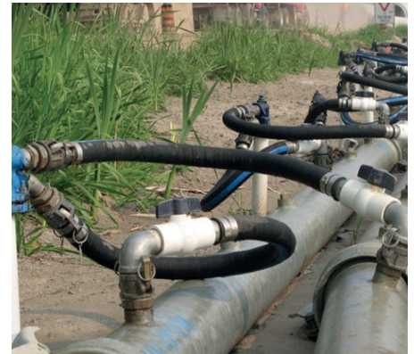
Figure 6 Ejector method of dewatering being used on site, with series of flow and return header pipes connected to series of wells
