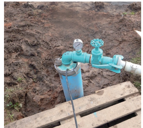
Figure 5 Wellhead of deep well being used for borehole pumping
