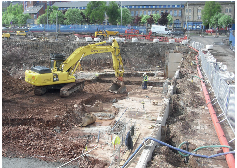
Figure 4 Shallow-well suction pump dewatering (along right margin of image) with header pipe (orange pipe) connected to shallow well riser pipes
