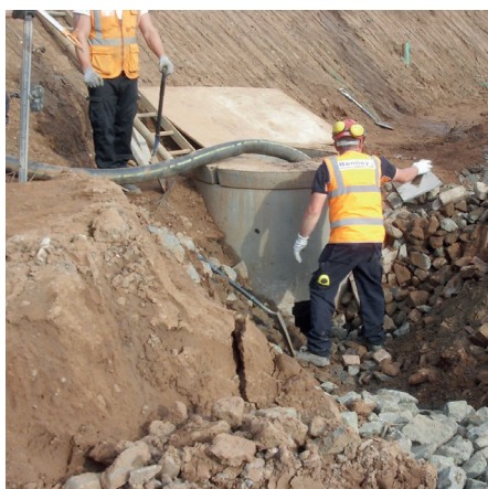
Figure 2 Sump pump dewatering on site. Large grey discharge pump hose emerging from sump
