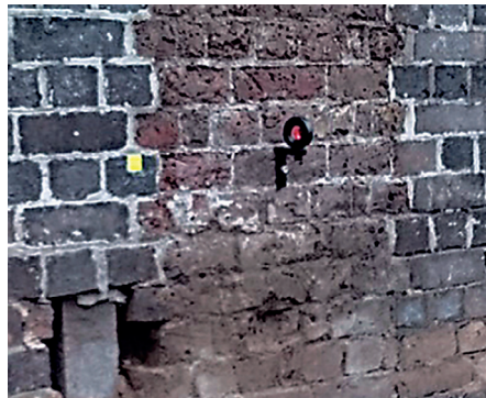
b) Prism on building facade – part of automated monitoring installation using Automated Total Stations
